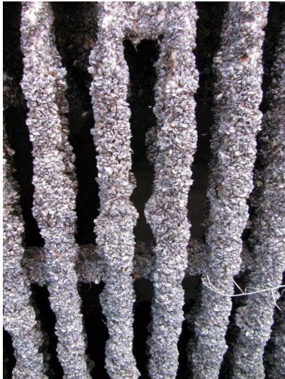
Figure 2. Lake Mead, Nevada Intake Trash Rack
