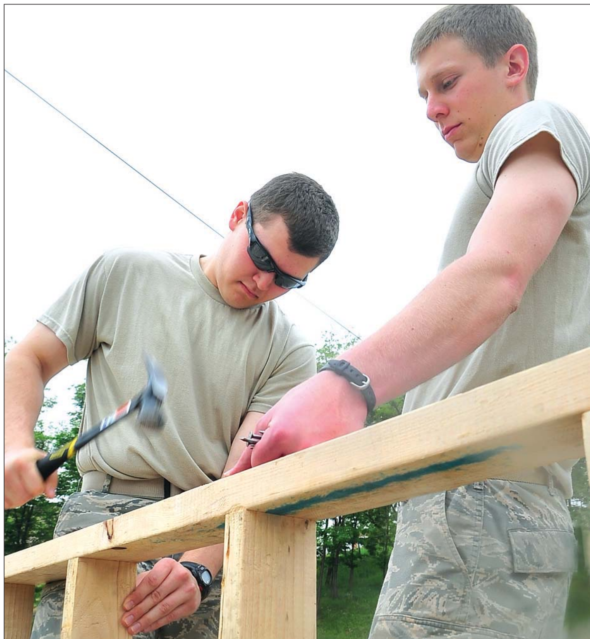
SENIOR AIRMAN ADAM GRANT Cadets 2nd Class Joshua Glass, and Reuben Luoma-Overstreet build a wall frame while working with the 51st Civil Engineer Squadron's Prime Base Engineer Emergency Force at Osan Air Base, South Korea, May 24.
