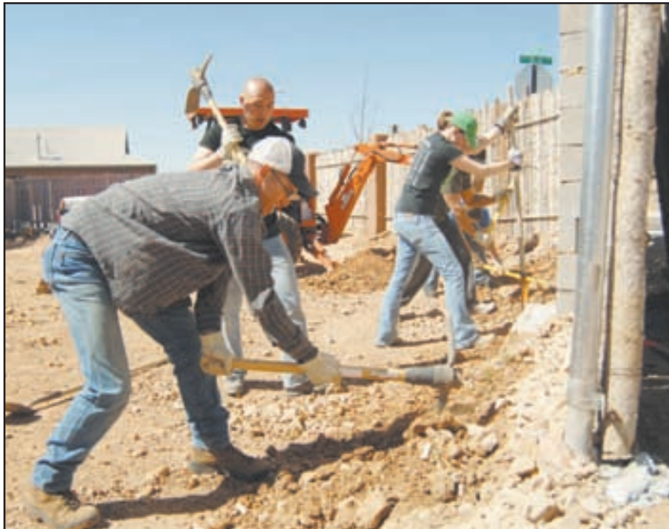
Cadet 3rd Class Ben Shoptaugh (front) and Cadet 4th Class Anthony Langdon take their turns with pick-axes as Cadet 2nd Class Dani Rogowski uses a shovel to clear away the broken rocks and dirt as fellow cadets make short work of a land-clearing project in Santa Fe, N.M.
