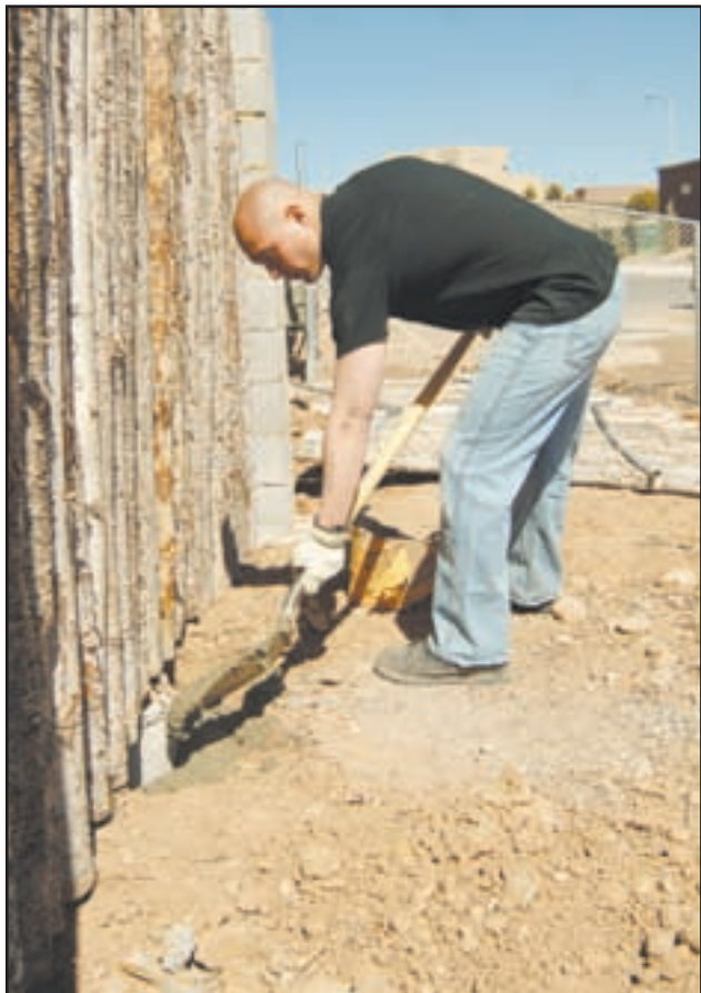
Cadet 4th Class Anthony Langdon, Cadet Squadron 33, adds concrete to secure new fence posts.
