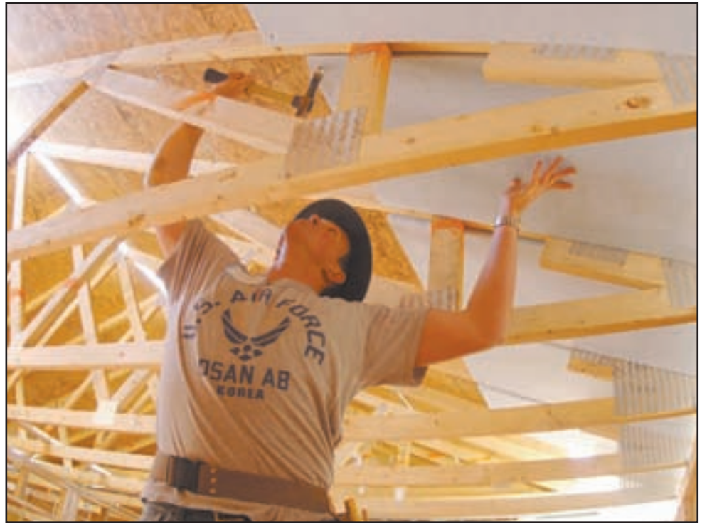
Cadet 3rd Class Matt Guertin holds insulation steady while nailing it in place.
