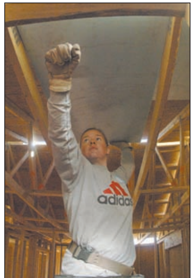
Cadet 4th Class Michelle Paranteau persuades a tight-fitting piece of insulation into place with her fist, while helping build a home during her spring break, via Habitat for Humanity.
