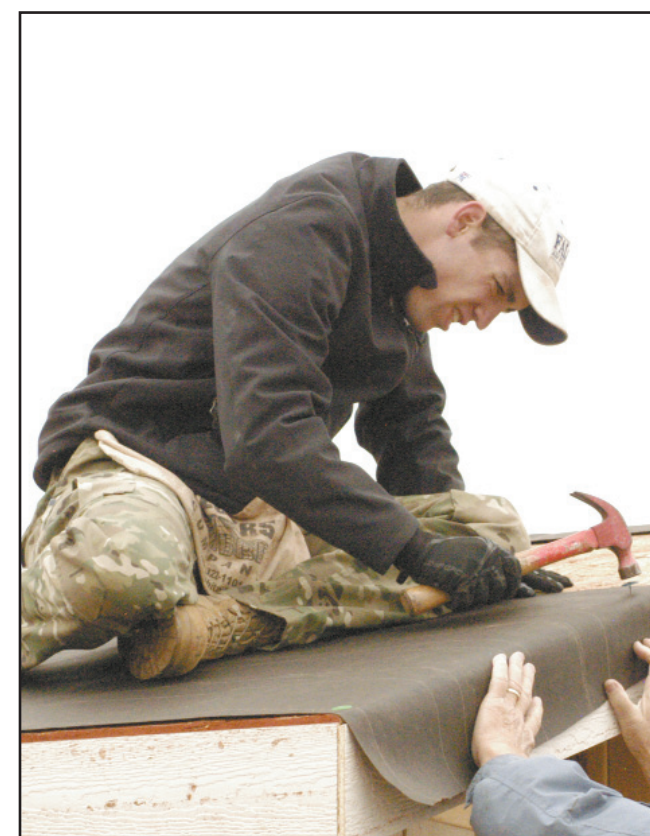
Cadet 1st Class Ben Shoptaugh from CS 12 weathersproofs the roof of a house in Wichita Falls.
