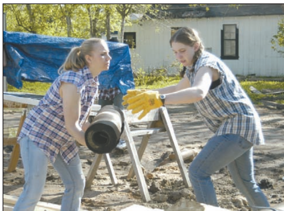
Cadet 3rd Class Sarah Sauter of CS 16 and Cadet 2nd Class Bridget Flatley of CS 37 work in muddy terrain while building a house as part of a Habitat for Humanity project March 22 in Victoria, Texas.
