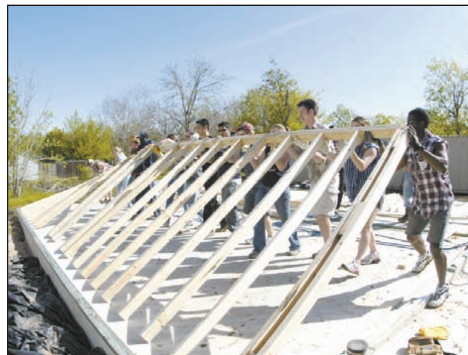
Cadets lift the west wall of a home in Victoria, Texas, March 22.
