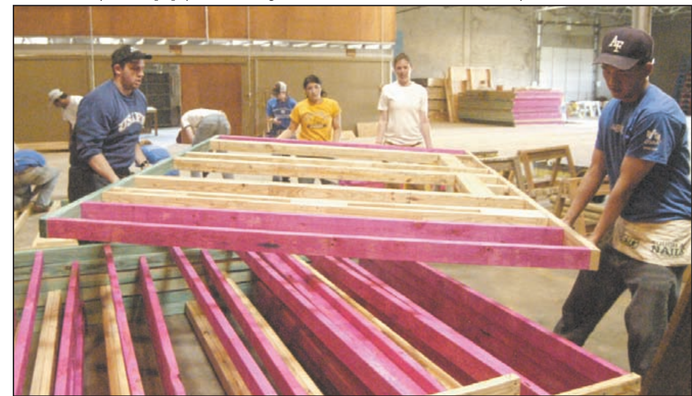
Cadet 1st Class Dan Paladino from CS 36, Cadet 2nd Class Paola Gavilanes from CS 24, Cadet 4th Class Kristin Cromwell of CS 29 and Cadet 1st Class Alex Chung from CS 16 stack a wall frame in a warehouse March 23 in Bryan, Texas.
