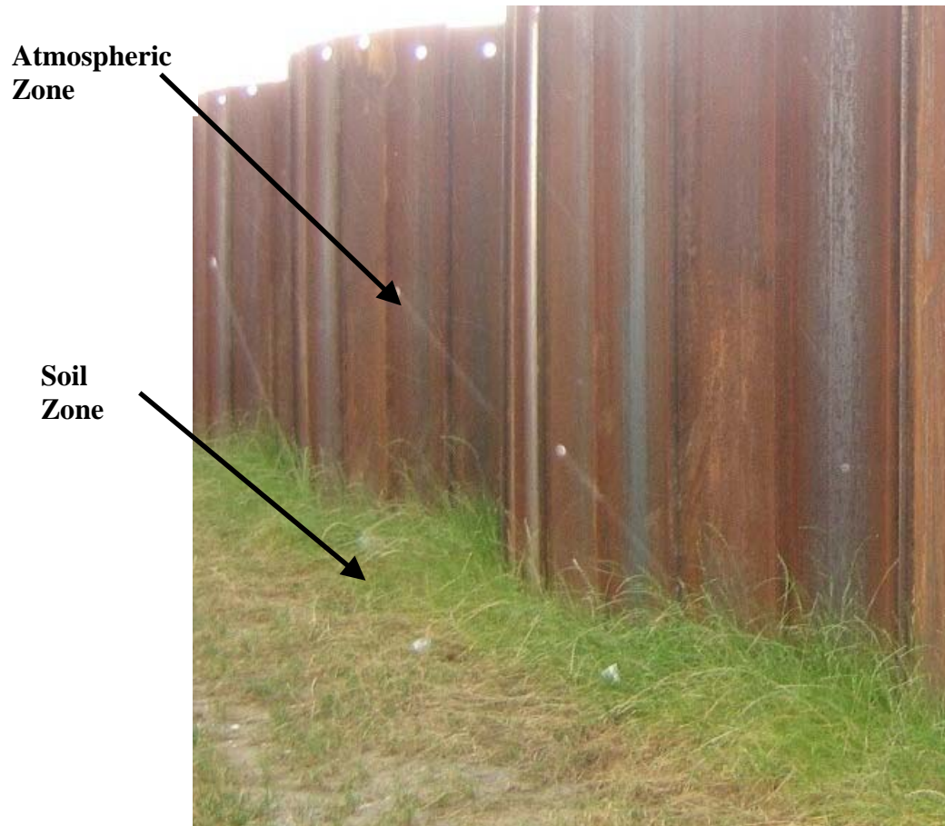
Figure 1.3-1. 17th Street Canal Sheet Piling – Typical Atmospheric and Soil Zones of Corrosion
