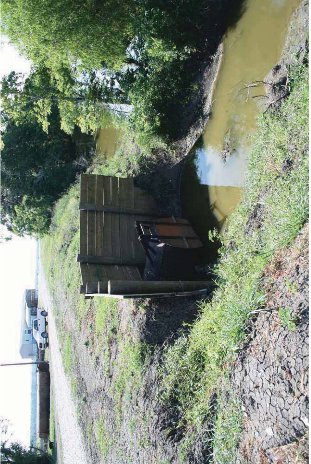
Figure 2. Culvert with Flap Gate at Tributary and Bayou Tortue Lower Reach Confluence
