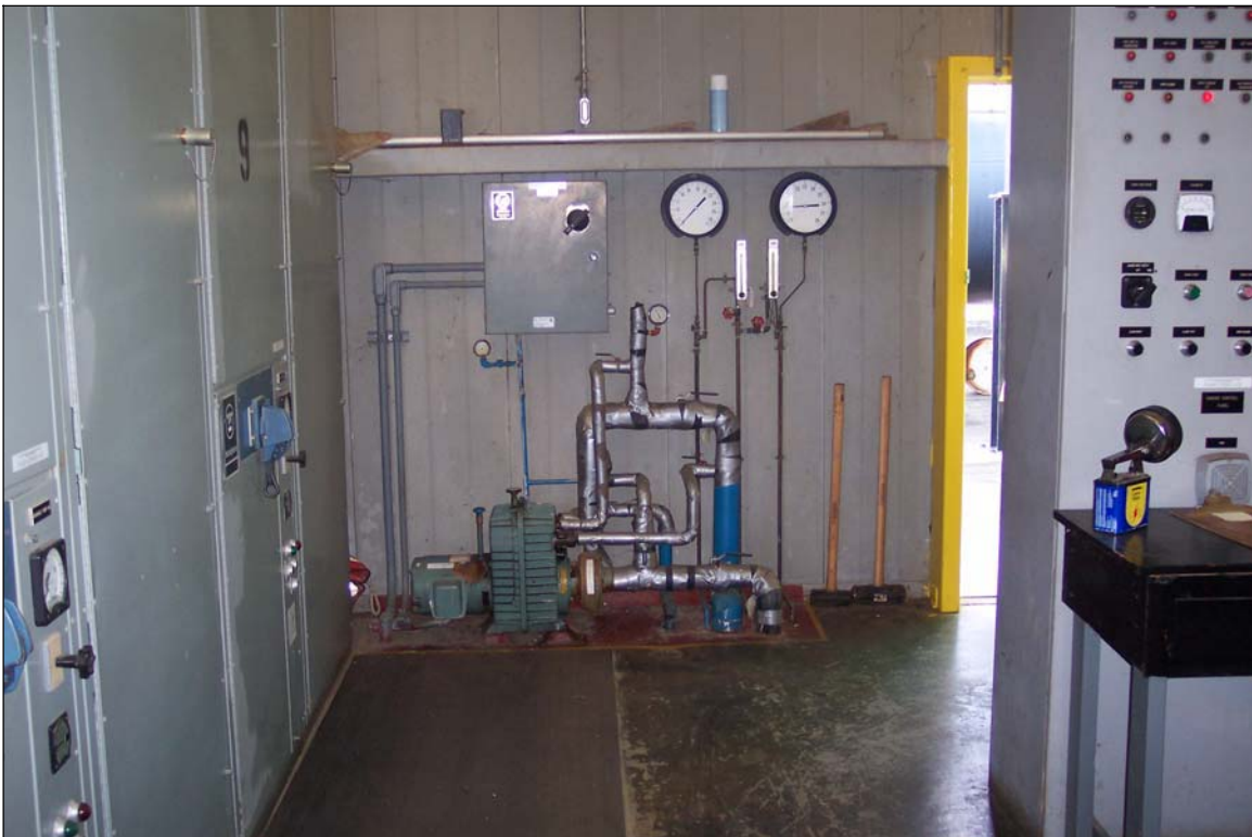
Photograph 8. Interior of pump station showing water service connection
