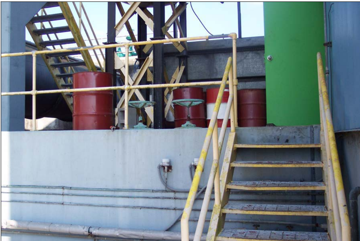
Photograph 10. Empty drums on pump station floor
