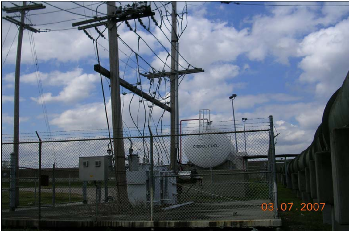
Photograph 7. Transformer station on subject property
