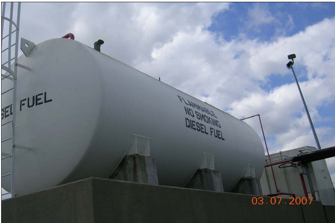
Photograph 6. Diesel fuel tank and containment basin
