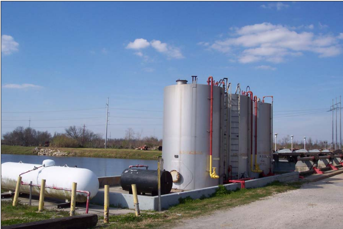
Photograph 3. Diesel, propane, and waste oil storage tanks
