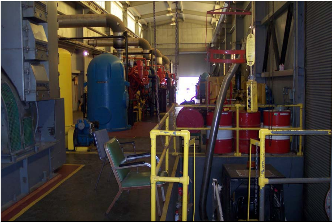
Photograph 9. Interior of pump station, oil storage
