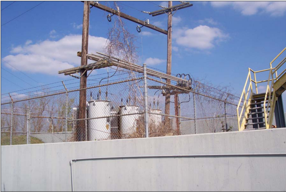
Photograph 5. Transformer station on subject property
