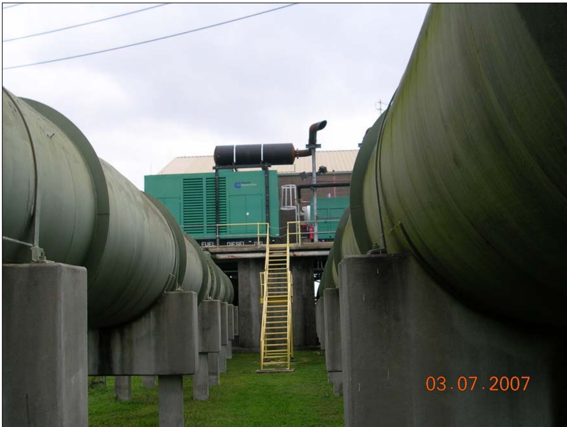
Photograph 5. View of pump station platform and generators toward the east
