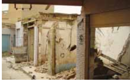
War-damaged Diyala suq.
