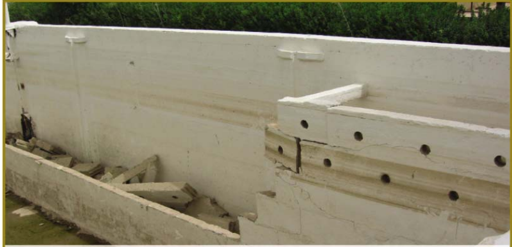
Al Wathba Water Treatment Plant: Train 1 settling tank shows a collapsed effluent weir wall
