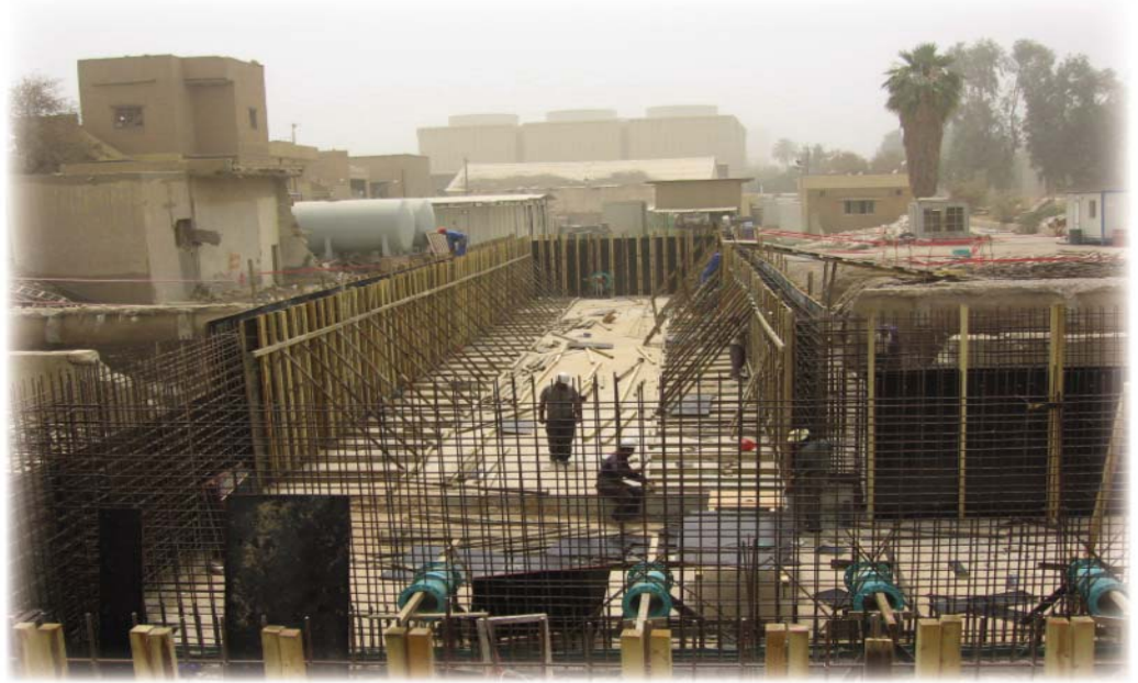
SIGIR TEAM TOURS WATER PLANT – An assessment team from the SIGIR inspects new construction at a central Iraq water treatment plant. SIGIR's engineer, auditor, and special agent determine the progress made in upgrading the facility with Iraq Relief and Reconstruction Funds and whether the upgrades meet contractual requirements.
