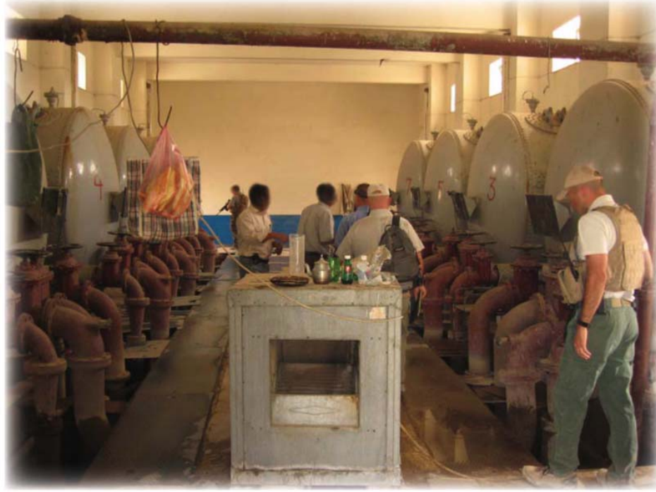
SIGIR TEAM TOURS WATER PLANT—An assessment team from the SIGIR inspects a water treatment plant in central Iraq to examine construction progress associated with an upgrade of the facility, paid for with Iraq Relief and Reconstruction Funds.
