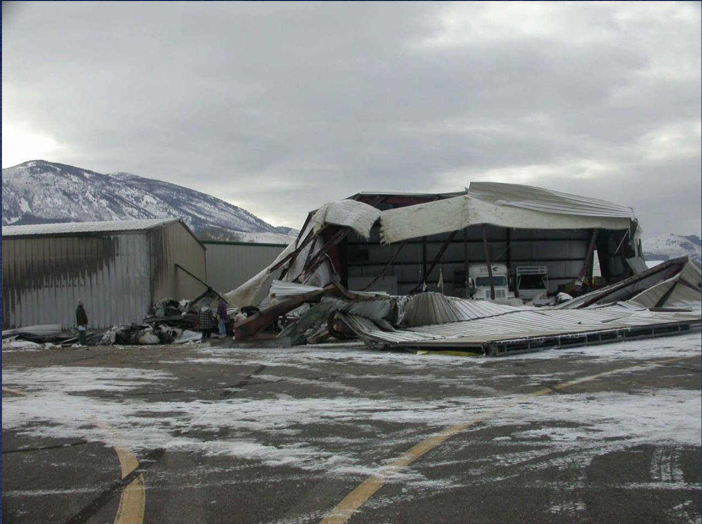
Image 2. Looking south toward front (north side) of impacted hangar. Wreckage is near left center of photo.
