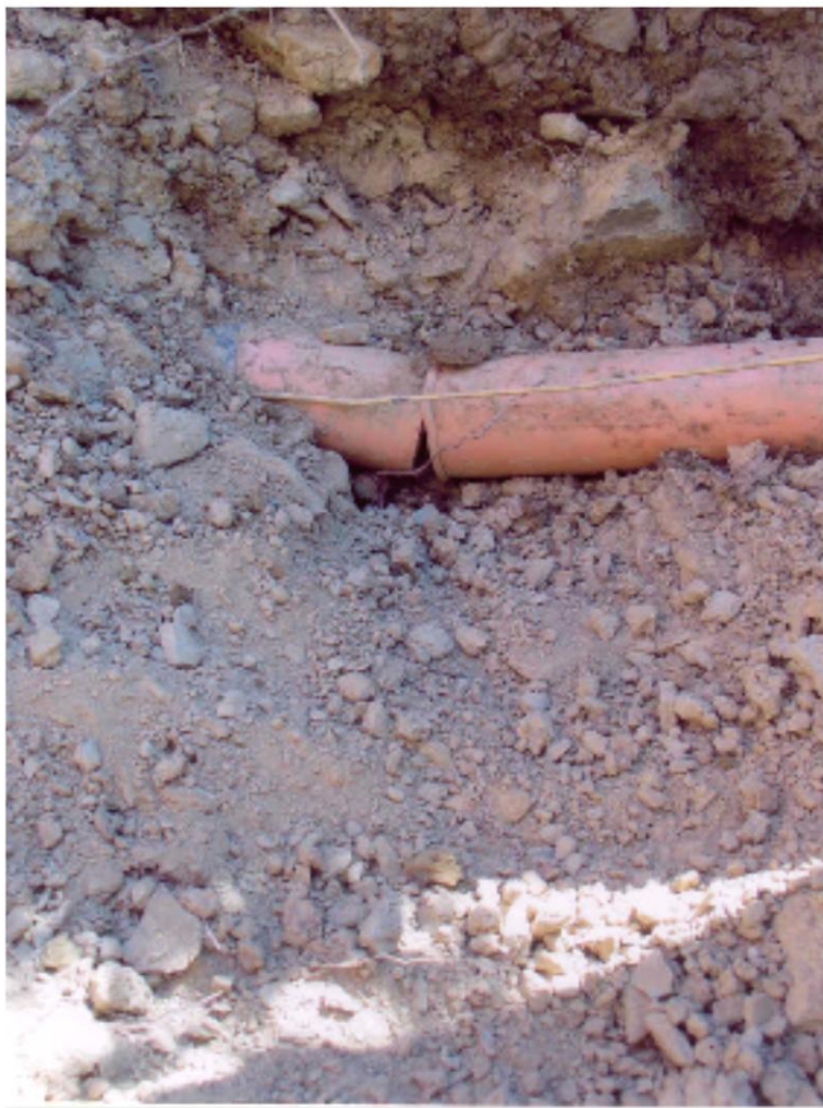
DuBois pipe failure
