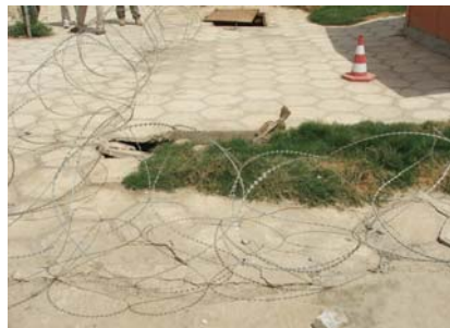
A collapsing septic system at Hilla Police Academy: an example of poor construction under contracts awarded to Philip Bloom.
