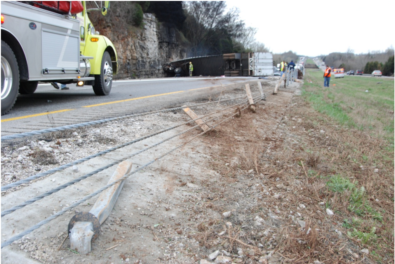
Figure 12. Overridden and damaged cable barrier.
