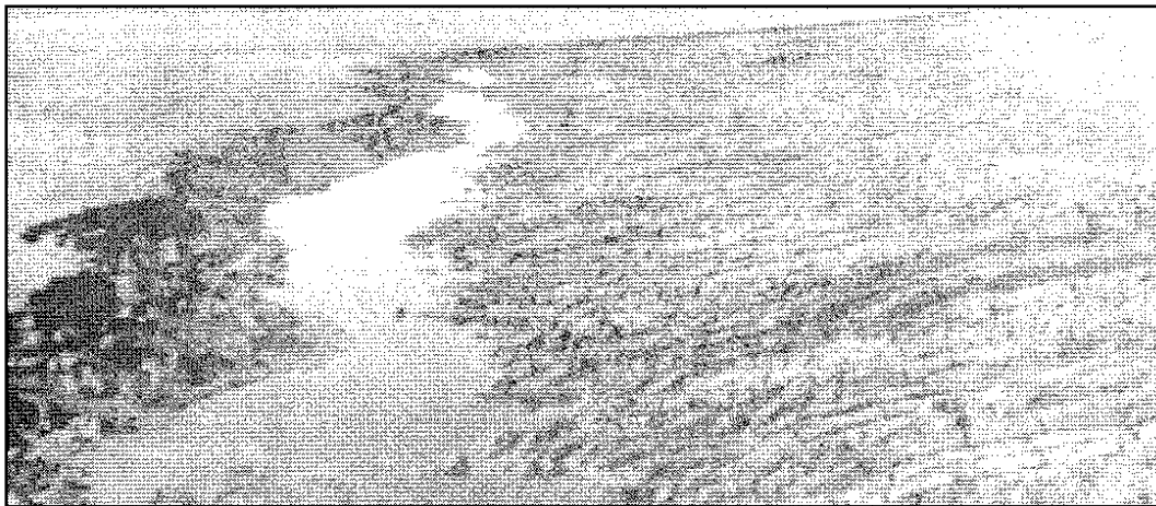
Figure B6. Construction of ditch 12 to 18 inches deep with excavated material cast on interior slope of perimeter dike.
