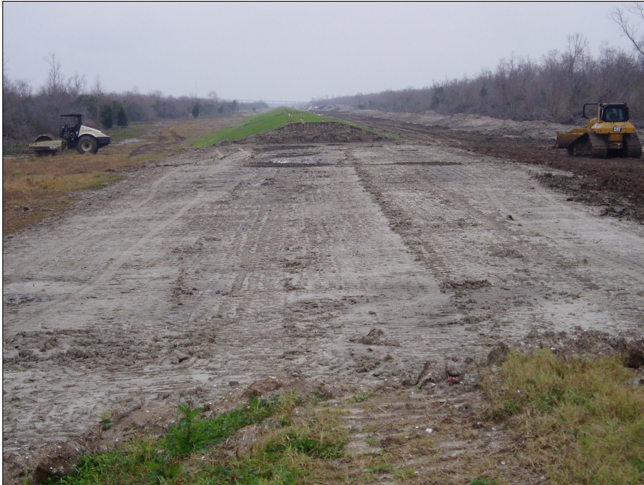
Figure 13. Flood control levee north of MRGO disposal area, presently under reconstruction. MRGO disposal area lies to the right of the photo with the north boundary running parallel to the levee.
