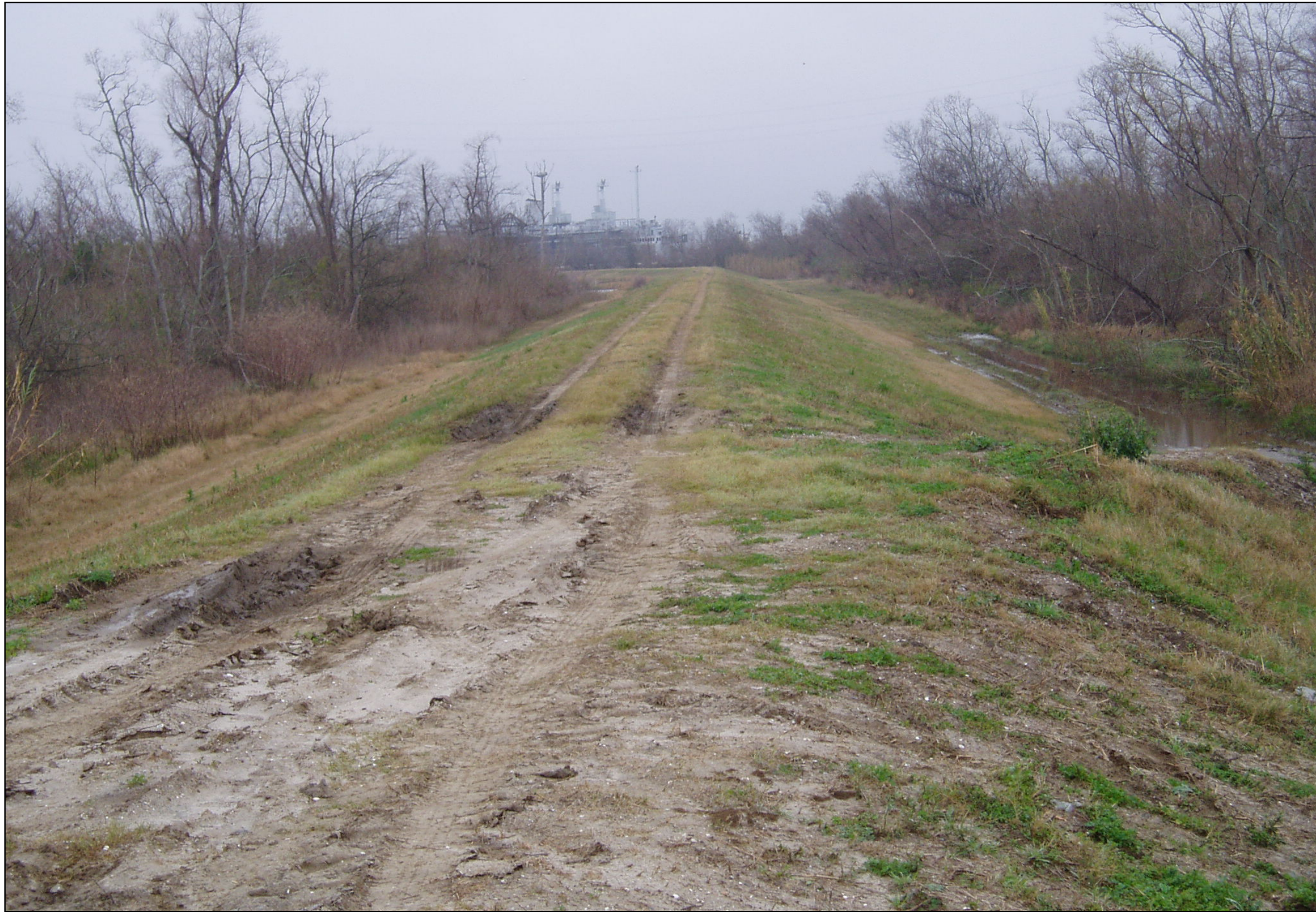
Figure 14. Existing flood control levee access to MRGO disposal site, looking west. Northwest corner of disposal site lies to the left, out of view of the camera. Florida Avenue Bridge in the distance.
