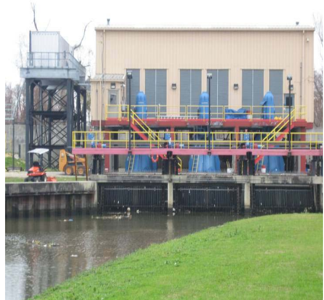
Photograph 1. Example of a Jefferson Parish Pump Station (Westwego #2; photograph taken on February 9, 2007).
