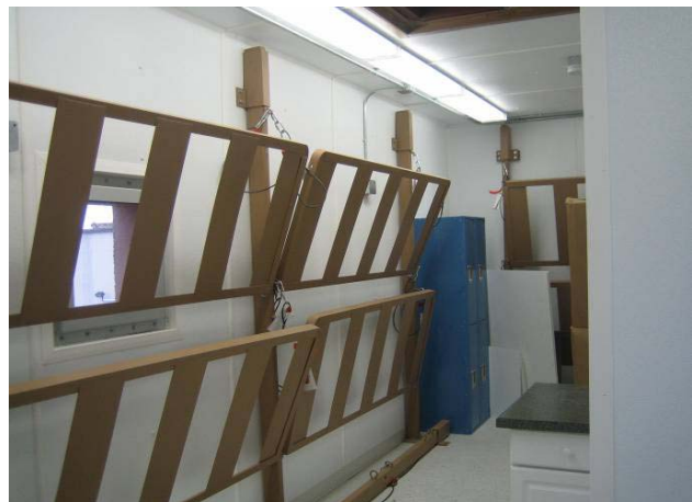
Photograph 3. Interior of completed safe room at the Duncan Pump Station (photograph taken on February 2, 2007).
