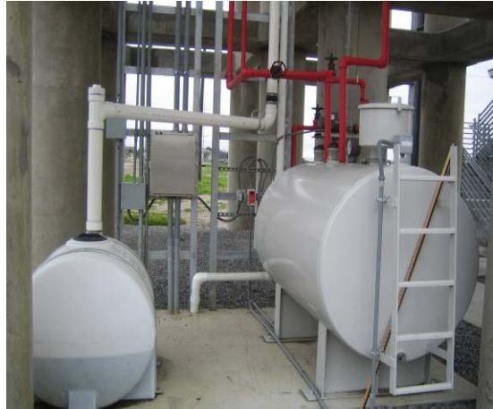
Photograph 4. 550-gallon diesel tank and septic tank at an existing safe room at the Duncan Pump Station (photograph taken on February 2, 2007)
