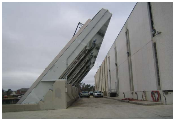
Photograph 5. Climber screen (to the left) at the Bonabel Pump Station (photograph taken on February 2, 2007).
