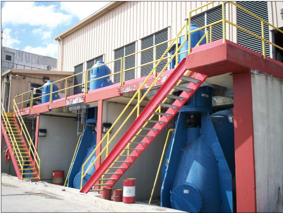
Photograph 3. Westwego pump station, view to the southwest
