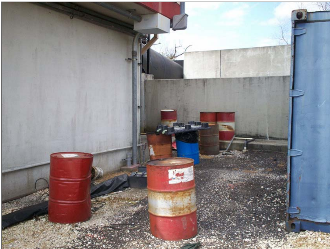
Photograph 4. Waste oil drums and stained ground adjacent to station
