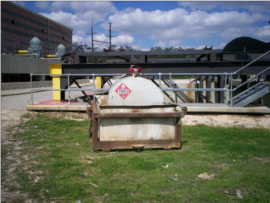
Photograph 7. Diesel fuel tank for construction in containment basin
