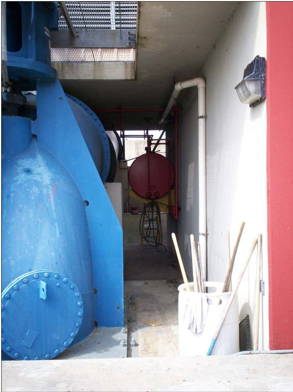
Photograph 14. Diesel day tank inside pump station
