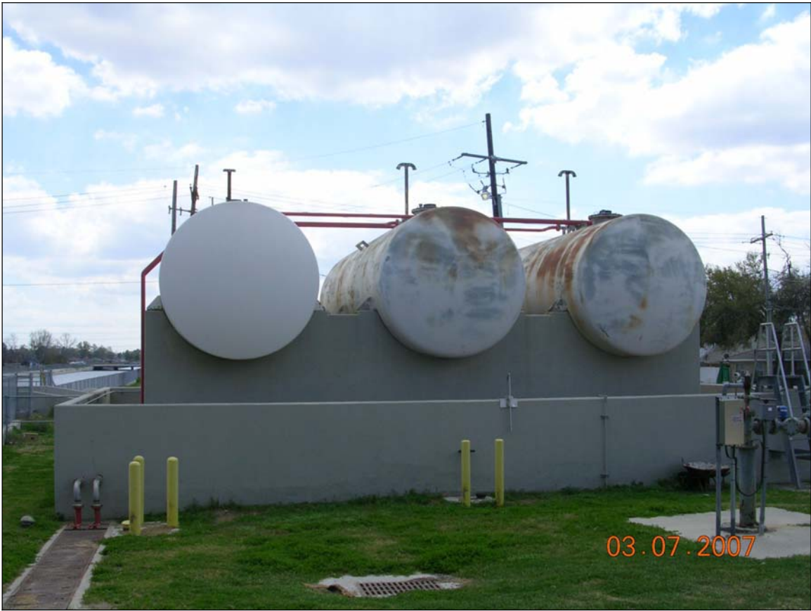
Photograph 7. Diesel storage tanks and containment basin
