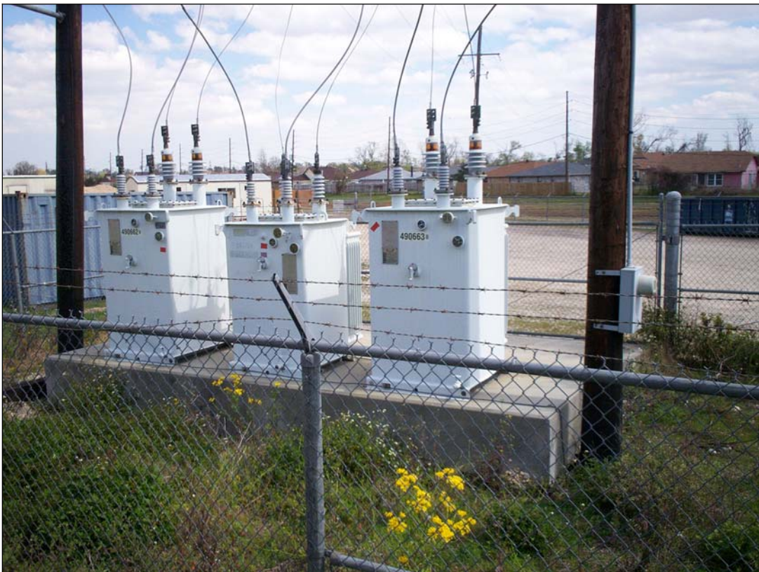
Photograph 8. Transformer station on subject property
