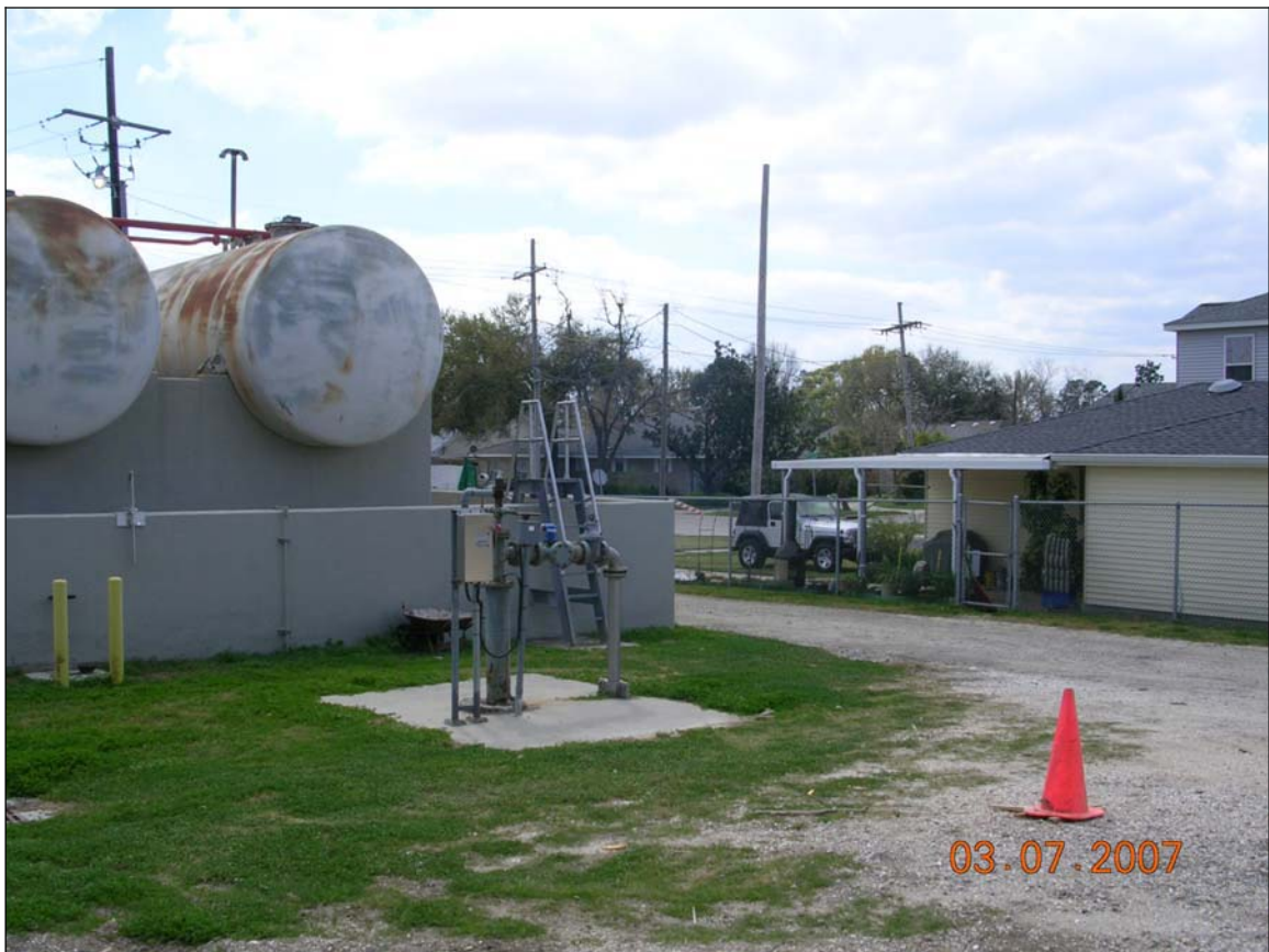
Photograph 6. Water well on subject property
