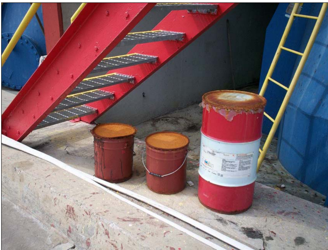
Photograph 12. Drums adjacent to pump station motors
