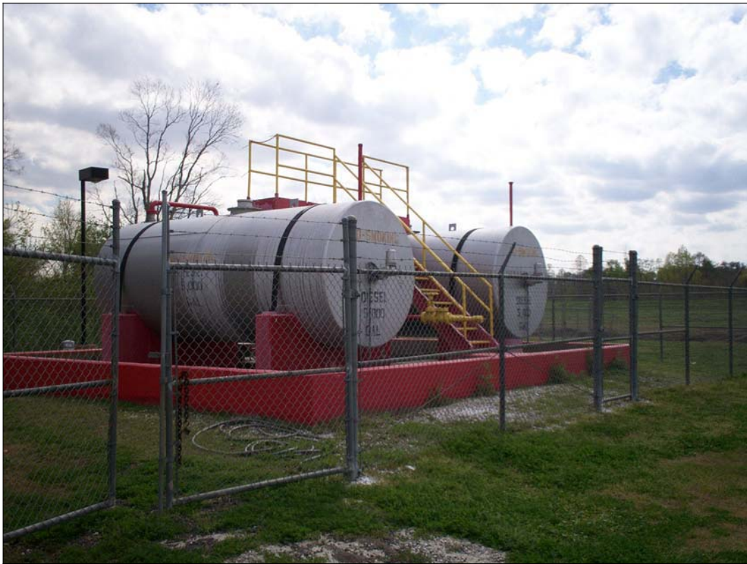
Photograph 9. Diesel storage tanks and containment basin
