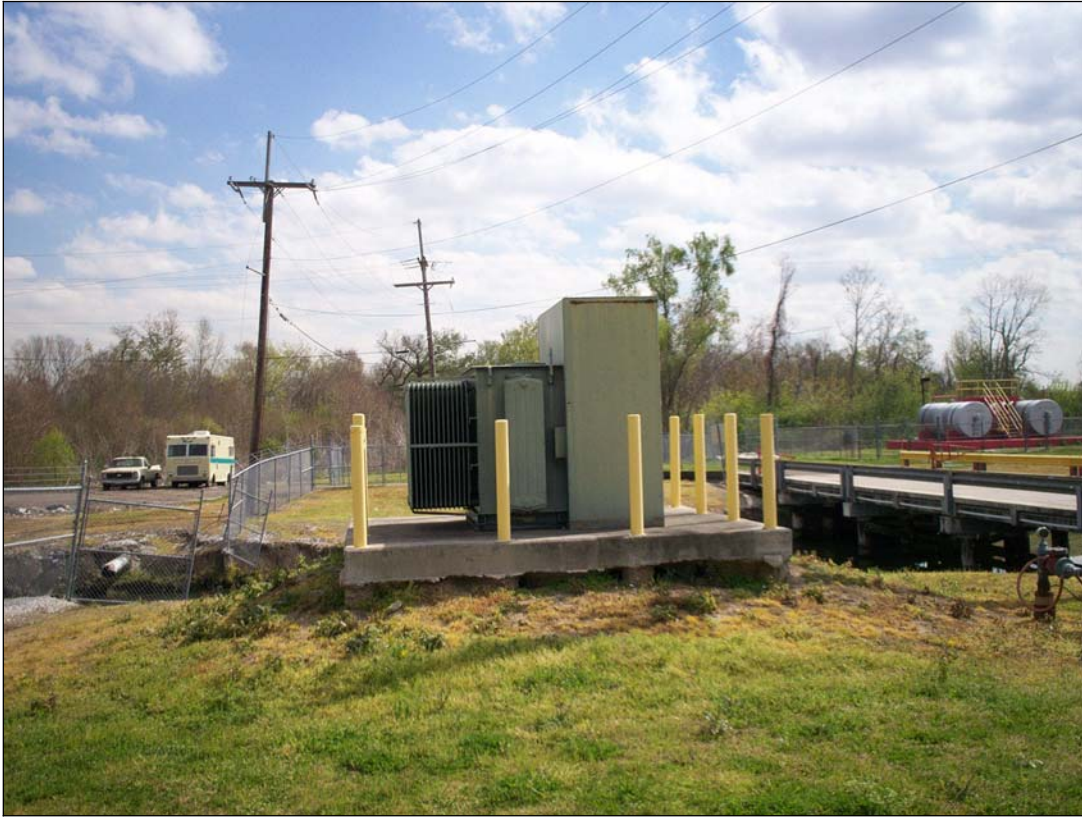
Photograph 7. Transformers on subject property
