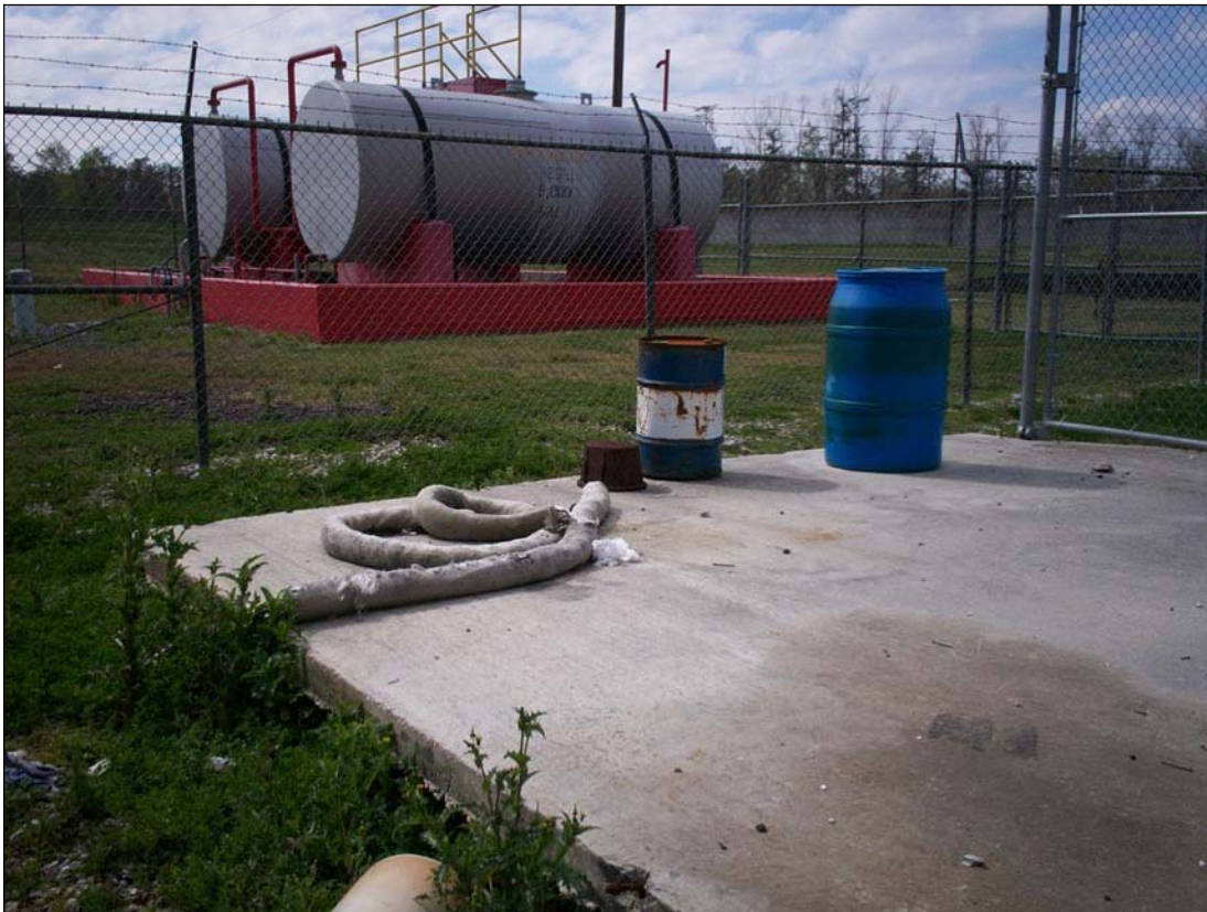
Photograph 8. Drums and staining on concrete storage yard pad
