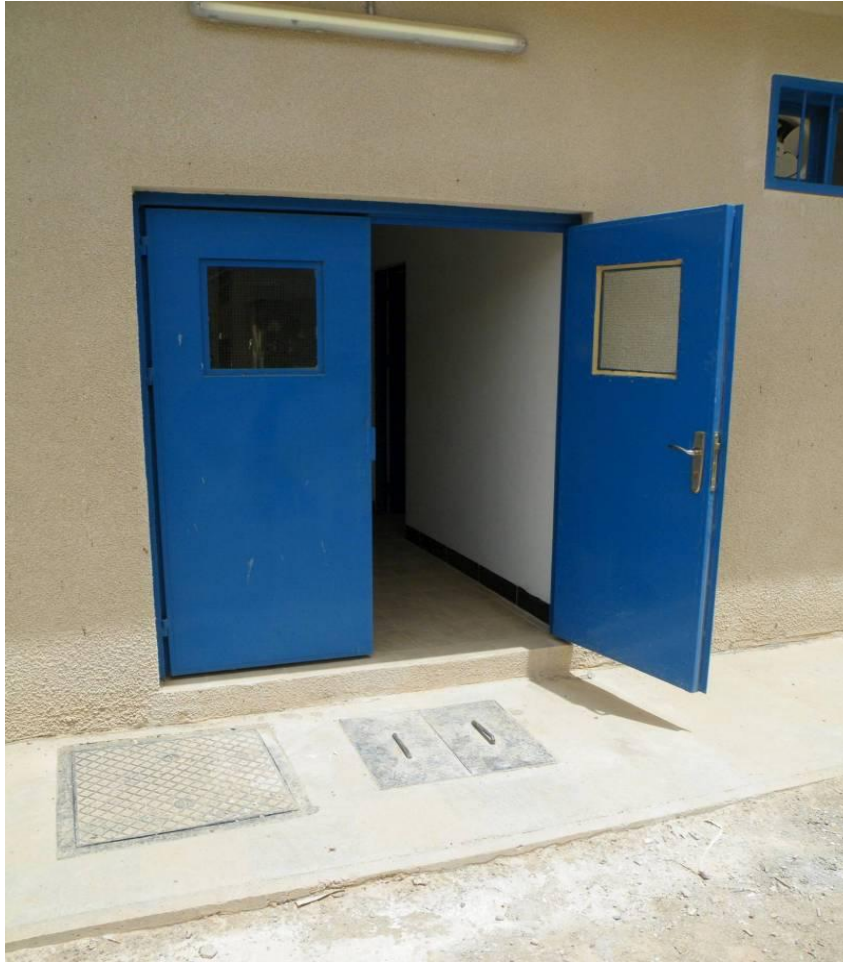
Site Photo 20. Tripping hazard outside the food storage and preparation building
