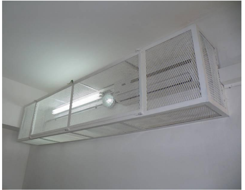
Site Photo 14. Metal cage protects the HVAC, light, and electrical wiring
