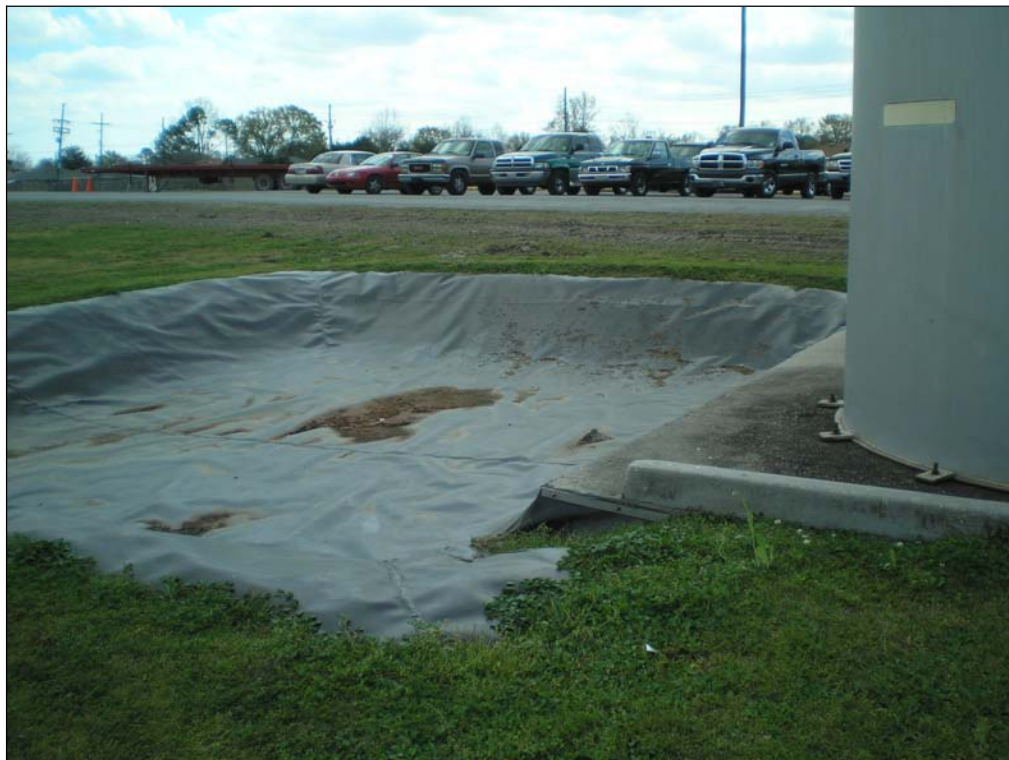
Photograph 12. Fuel spill/overflow containment basin
