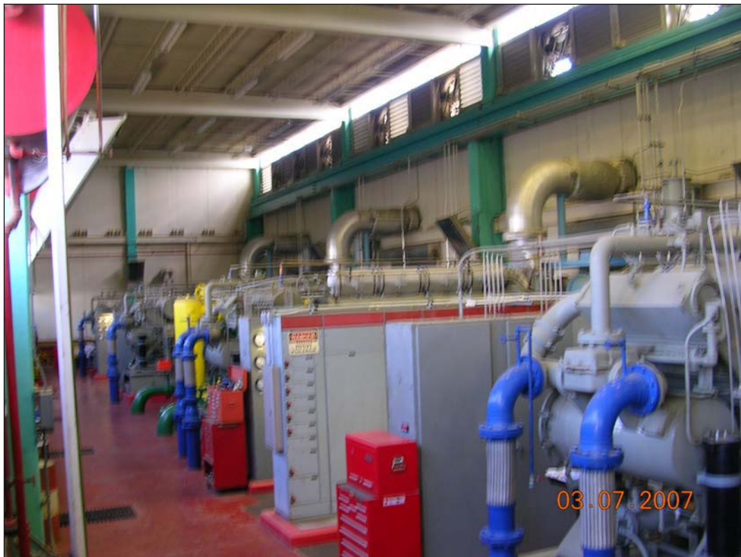
Photograph 11. Interior view of pump station
