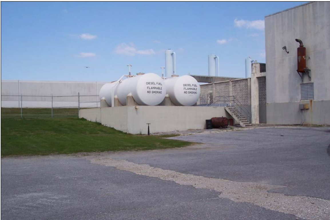
Photograph 2. Diesel storage tanks with containment basin
