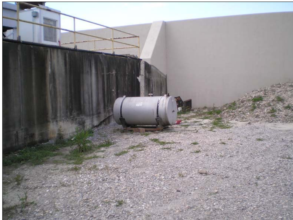
Photograph 8. Empty diesel tank near levee
