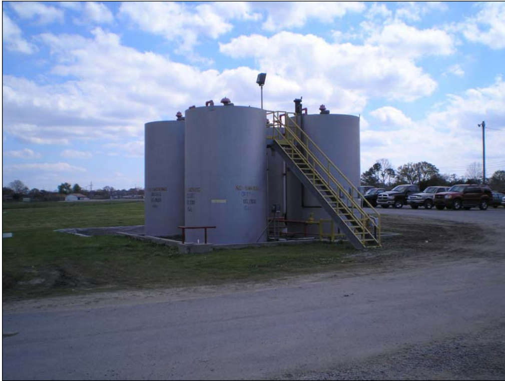
Photograph 11. Diesel storage tanks on subject property
