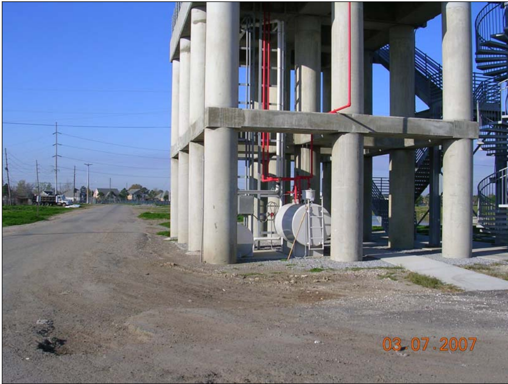
Photograph 1. Diesel tank at base of storm safe room
