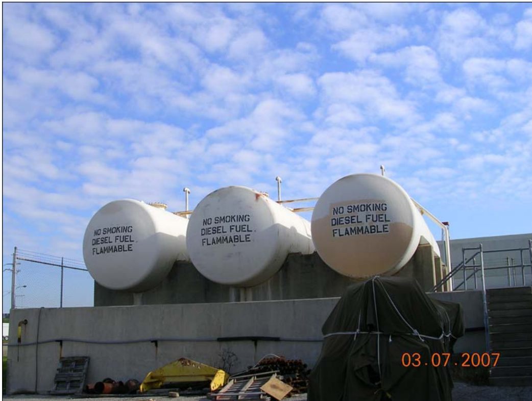
Photograph 4. Diesel storage tanks and containment basin
