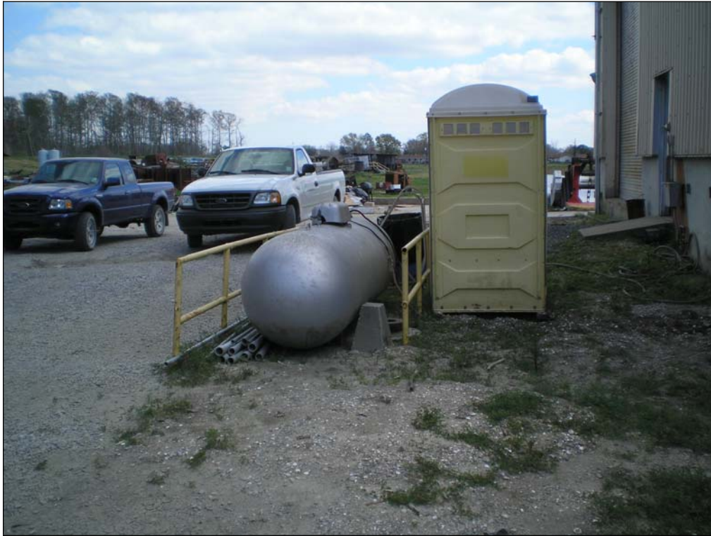
Photograph 9. Propane tank on subject property
