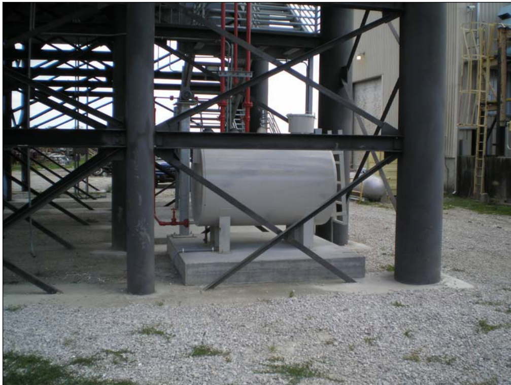
Photograph 6. Diesel storage tank under safe room
