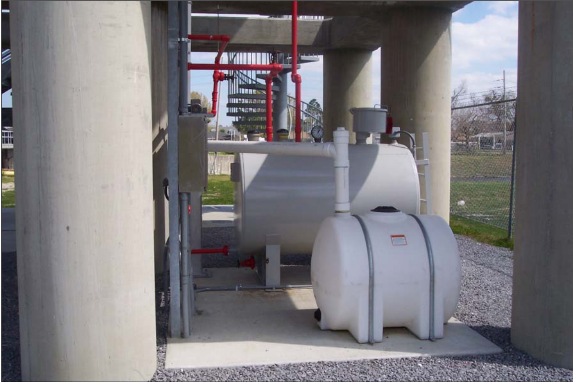
Photograph 1. Diesel tanks under safe room structure
