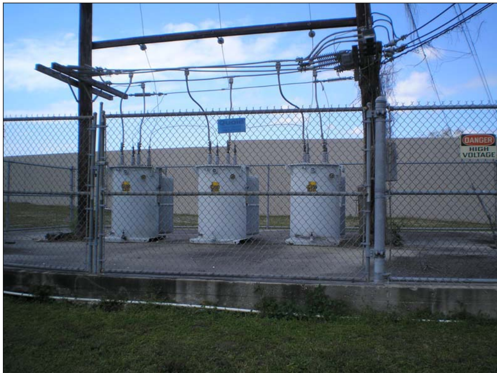
Photograph 10. Transformer substation on subject property
