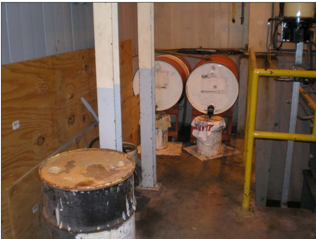
Photograph 22. Oil storage inside the station pump building
