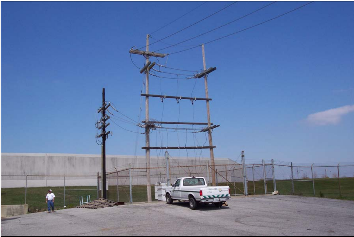
Photograph 3. Transformer station on subject property
