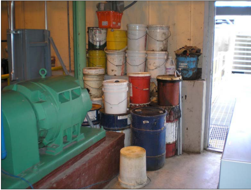
Photograph 21. Flammable liquids storage inside the station pump building
