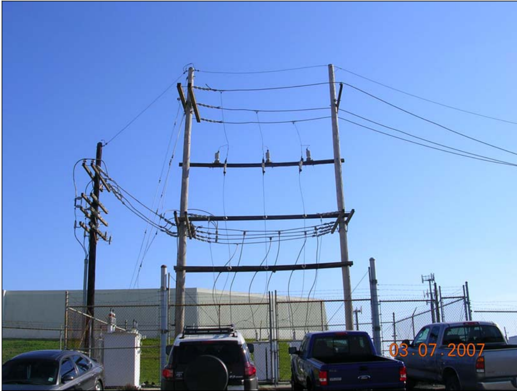
Photograph 3. Electrical transformers on subject property
