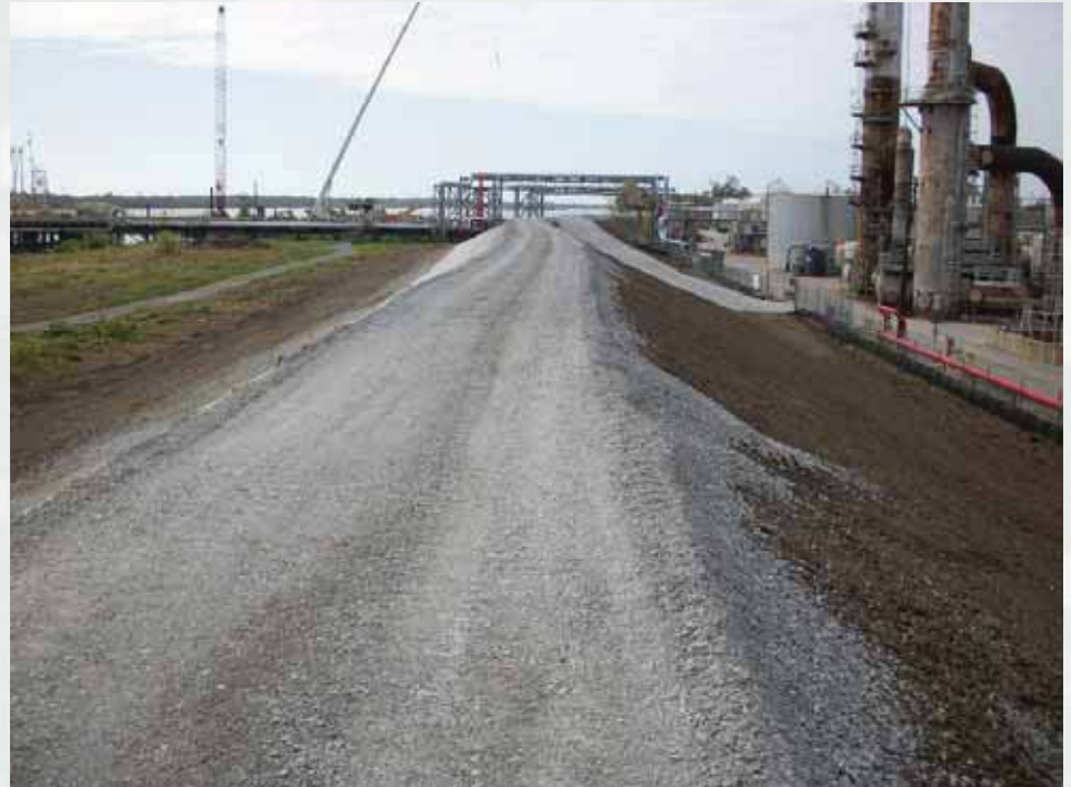
Engineered Alternative Measures were constructed primarily within existing right-of-way and with steep slopes.
