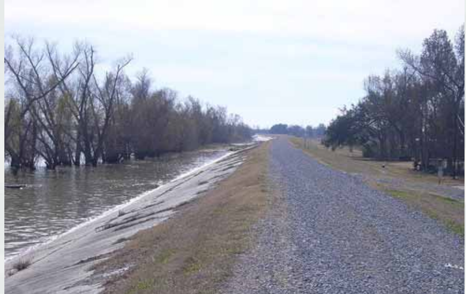
Many Mississippi River levee stretches include gravel topped crowns and concrete slope paving on the flood or protected side.
