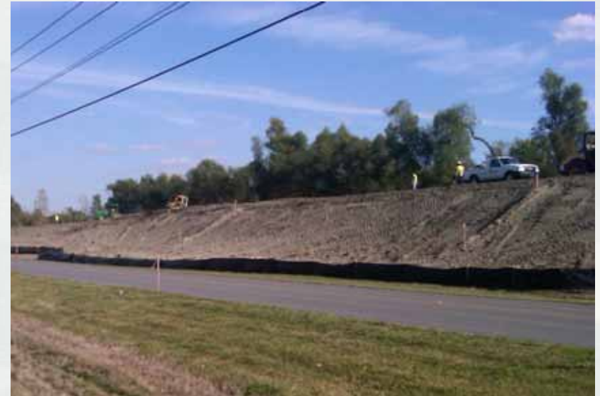
The Corps is constructing a 700 ft. demonstration section in Belle Chasse at the intersection of the river with F. Edward Hebert Blvd.
