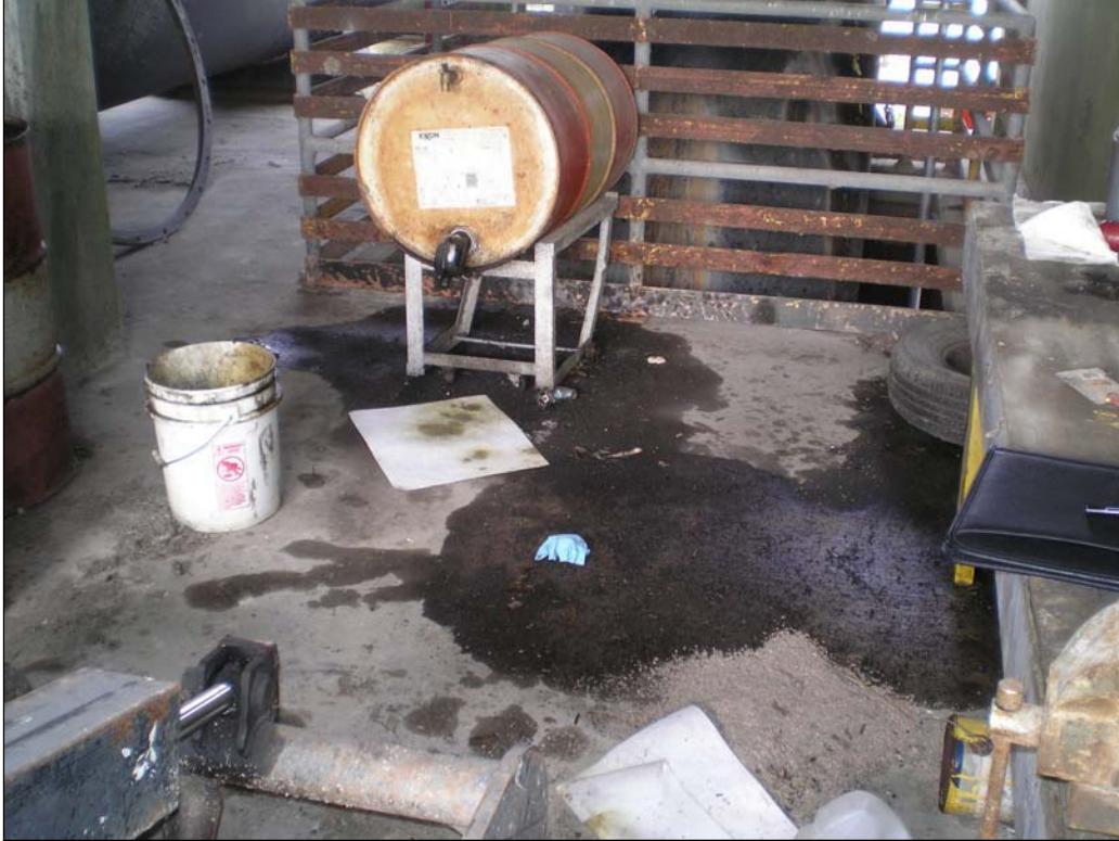
Photograph 3. Oil drums and stains inside old pump station building
