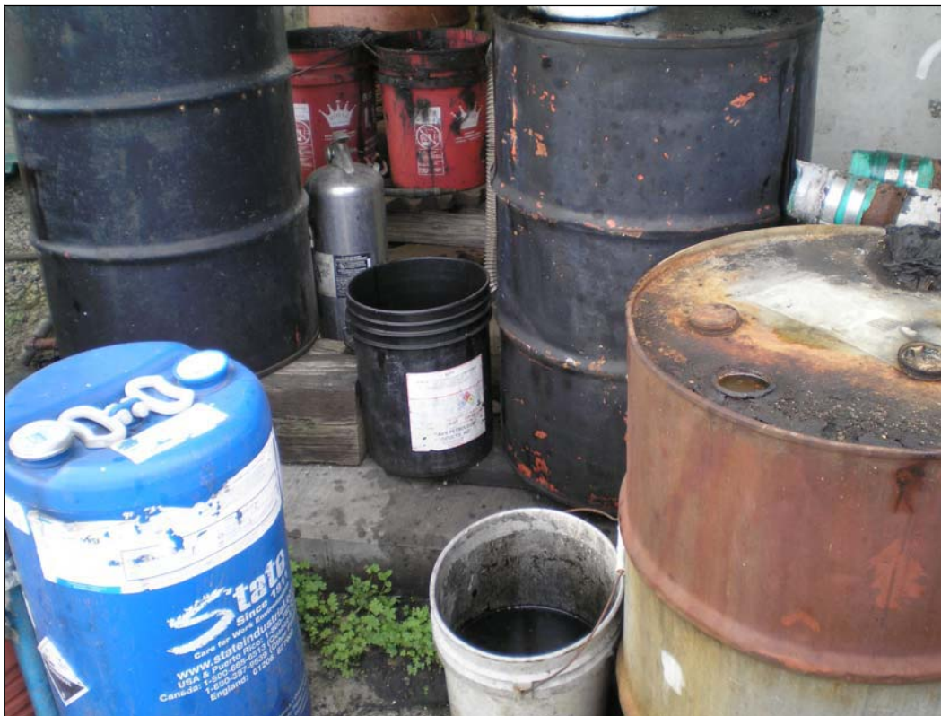
Photograph 14. Open oil containers and spills adjacent to the pump building
