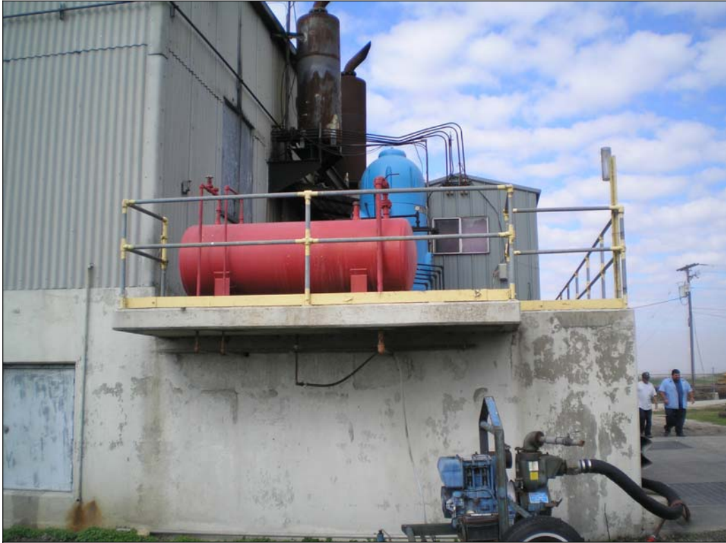
Photograph 15. Diesel storage day tank on deck of pump station building
