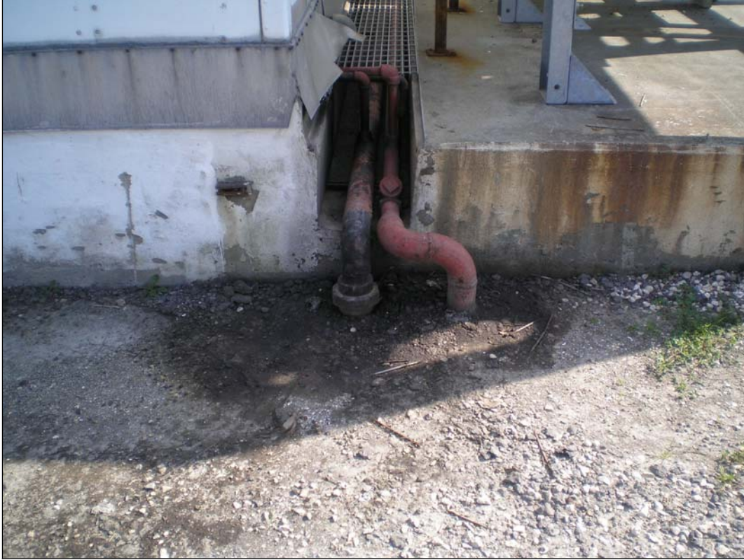
Photograph 13. Oil stained soil adjacent to generator station
