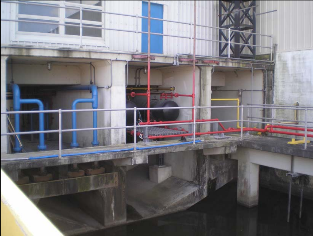
Photograph 4. Day tank diesel storage and intake sump of pump station
