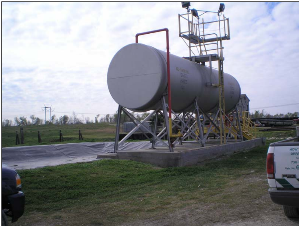
Photograph 6. Diesel storage tank with spill containment basin
