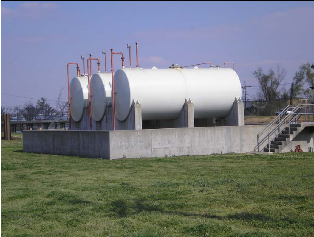
Photograph 9. Diesel fuel storage tanks with spill containment basin
