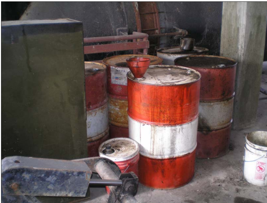
Photograph 4. Oil drums and spills inside old pump station building
