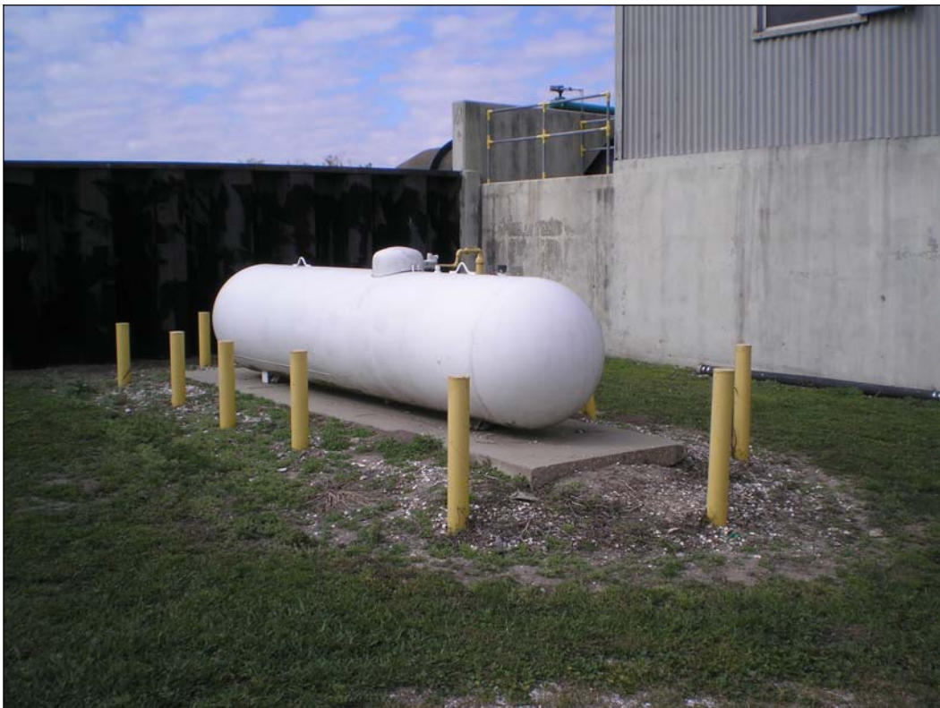
Photograph 16. Propane tank adjacent to pump building
