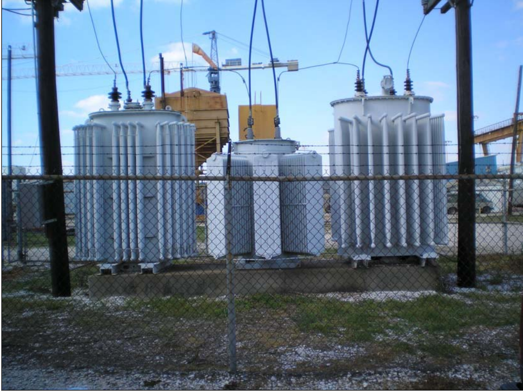
Photograph 5. Transformer station adjacent to pump station
