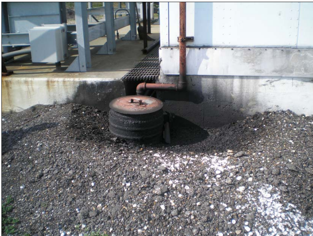
Photograph 12. Oil stained gravel adjacent to generator station
