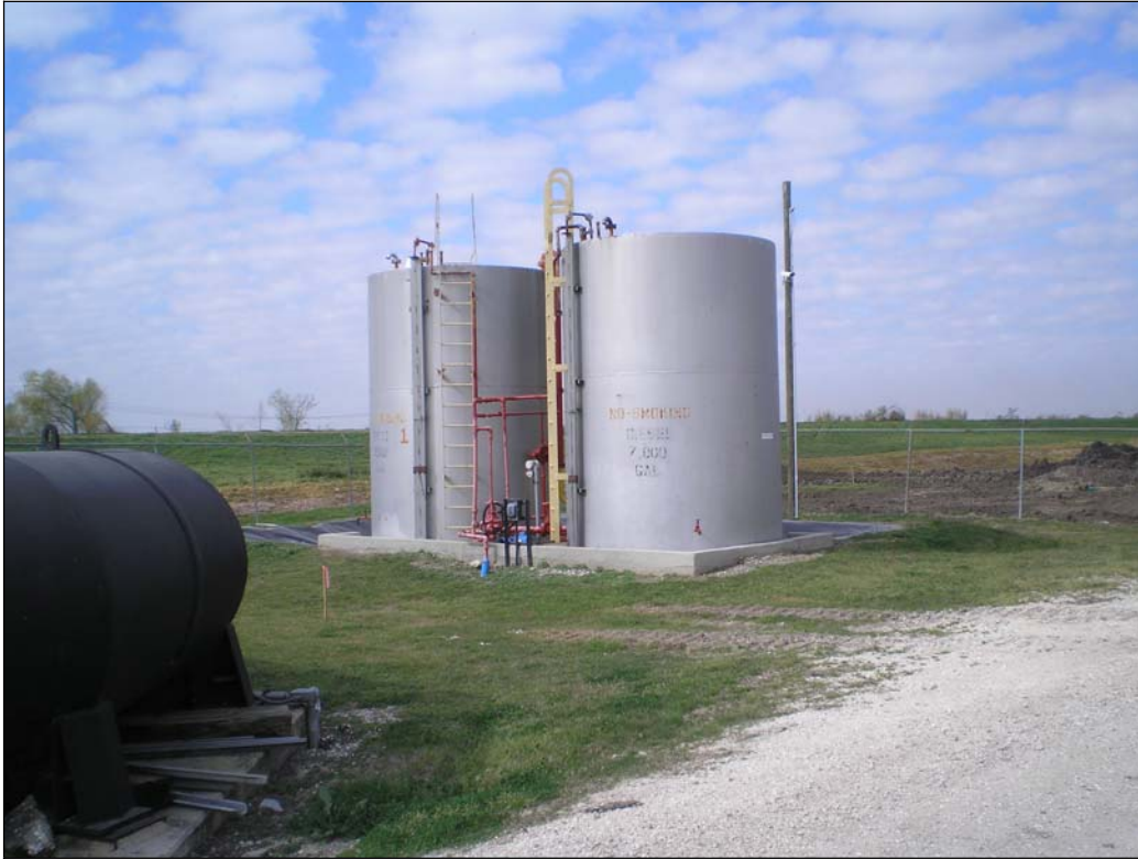
Photograph 7. Diesel storage tanks with spill containment basin
