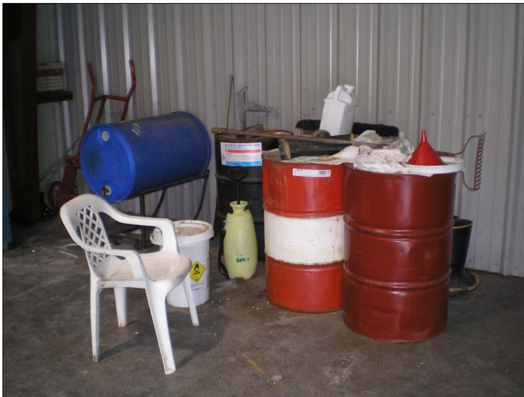
Photograph 2. Oil containers stored inside pump station
