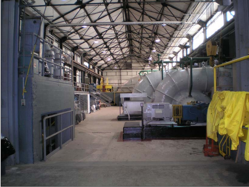
Photograph 3. Interior view of pump station, view to the south
