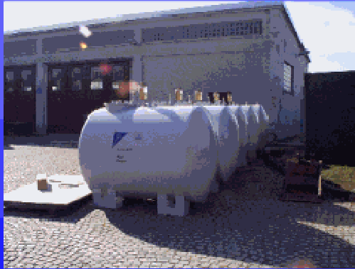
Fuel Storage on Hardstand with POL Separator
