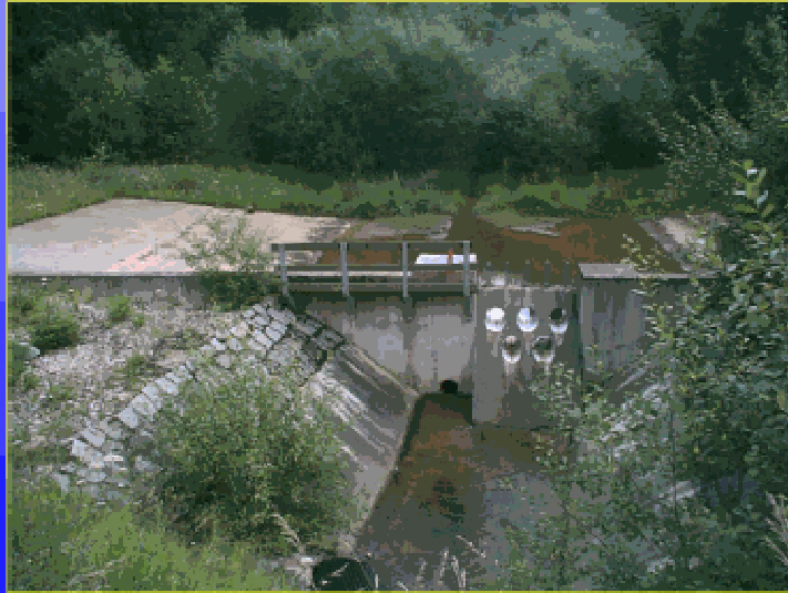
Check Dam at Grafenwoehr Training Area
