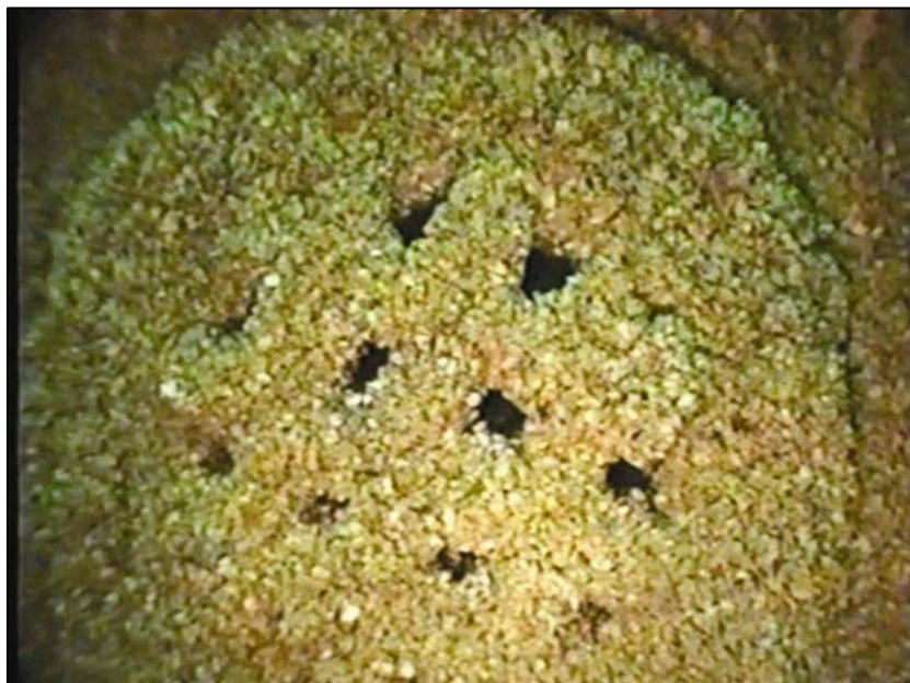
Figure 9. Underwater photo showing mussels covering the Davis Dam domestic water intake grate (photo courtesy of LC Diving and Marine Operations, 2008).
