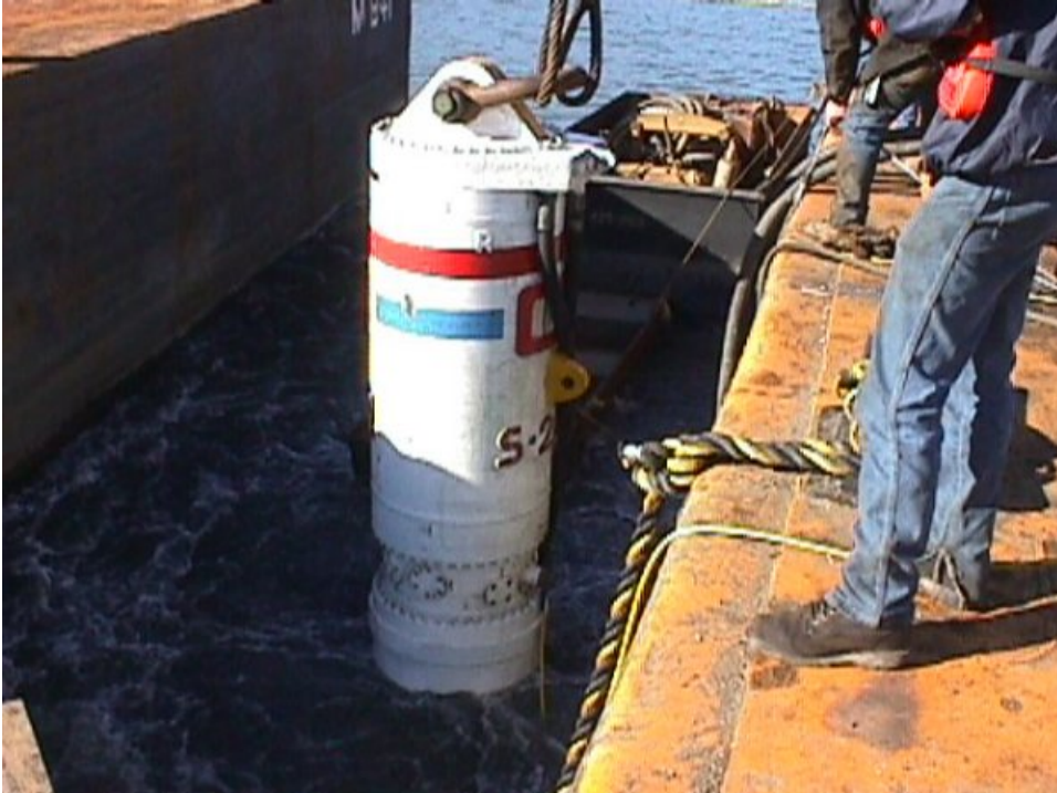
Boh Brothers Construction Company drives a 48-inch diameter test pile underwater. The pilings for the new lock will be driven underwater in the existing canal. January 2000.
