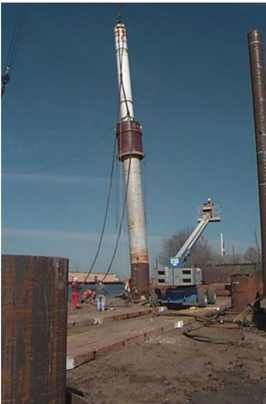
Boh Brothers Construction Company drives a 48-inch diameter steel pipe pile with an IHC 200-S hydraulic hammer. January 2000.
