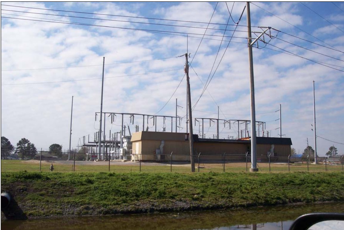
Photograph 18. Electric power substation adjacent to project corridor
