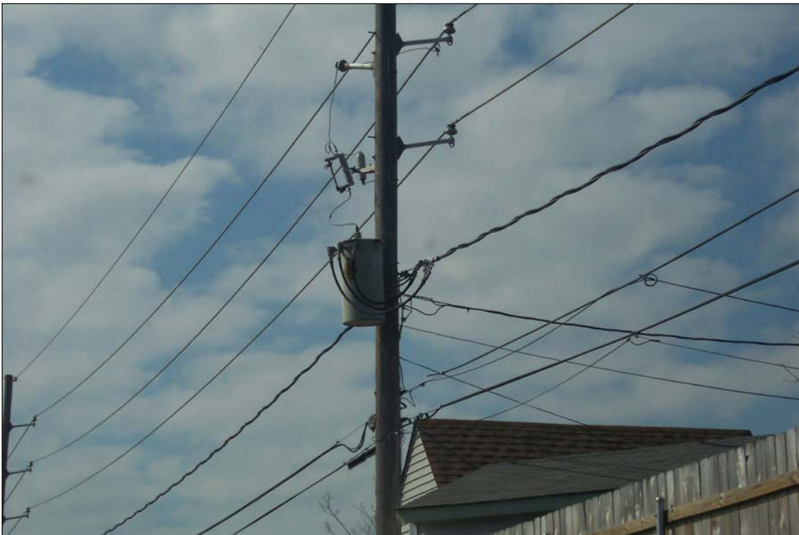
Photograph 16. Transformer adjacent to project corridor
