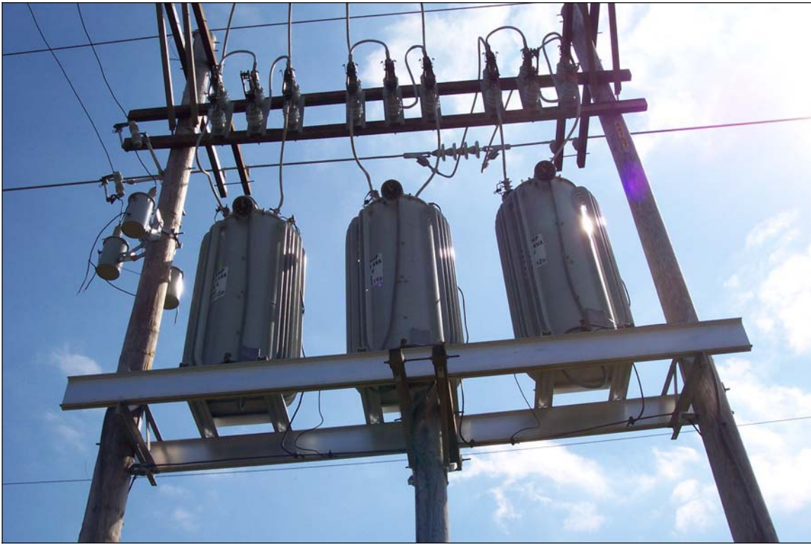
Photograph 15. Transformers adjacent to project corridor
