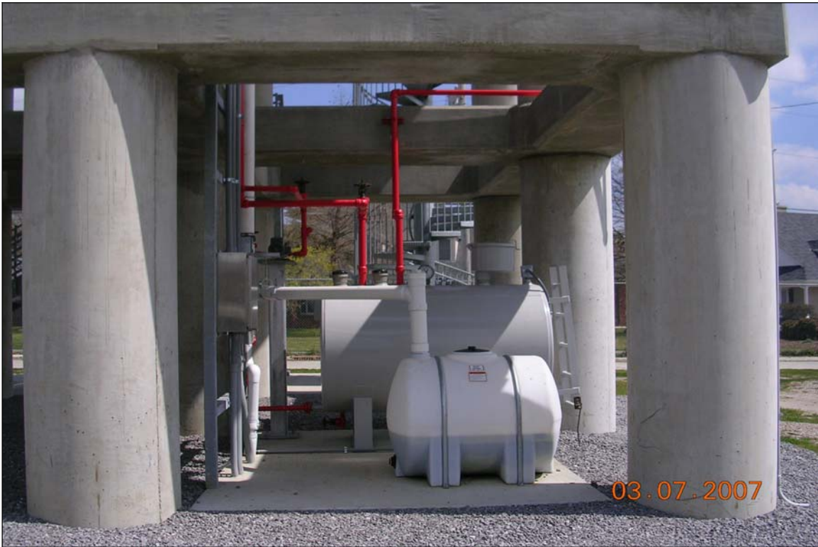
Photograph 7. Diesel tanks under safe room
