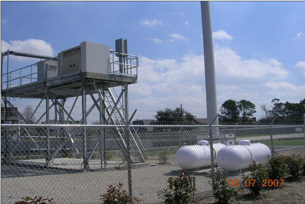
Photograph 3. Propane tanks adjacent to generators for cell tower
