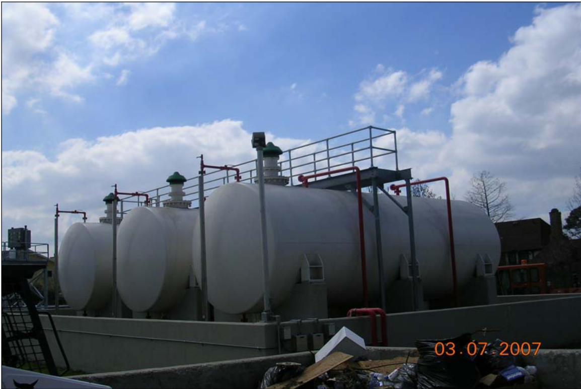
Photograph 5. Diesel storage tanks with containment basin
