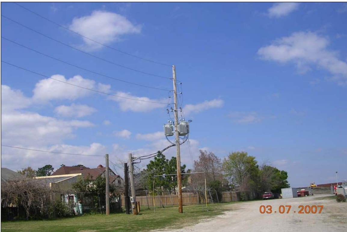
Photograph 2. Transformers on subject property
