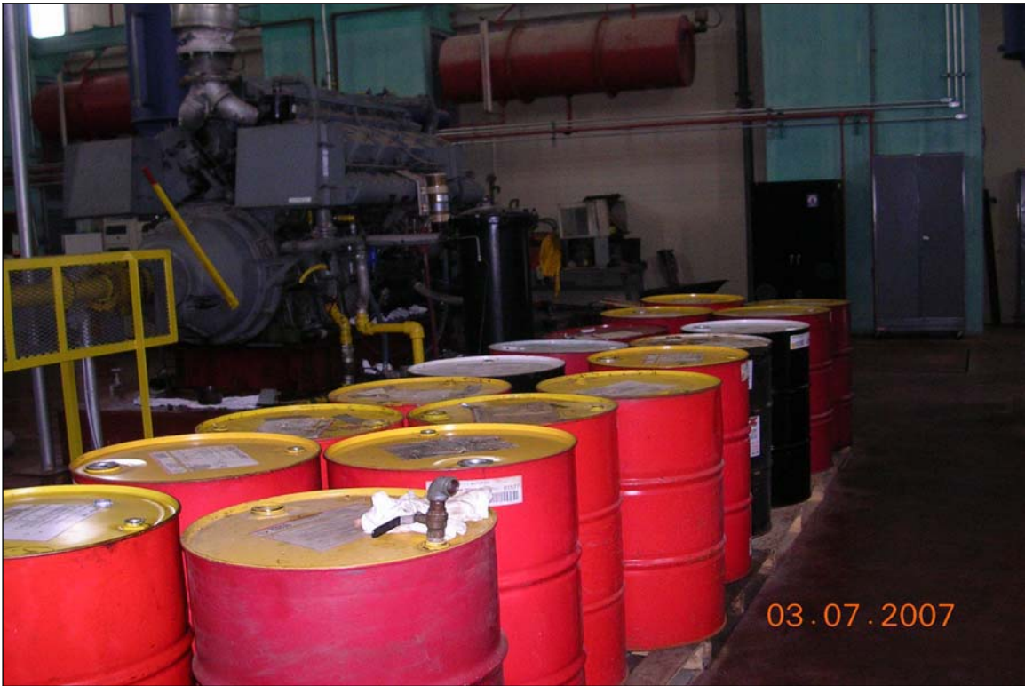
Photograph 11. Oil drums stored inside pump station building
