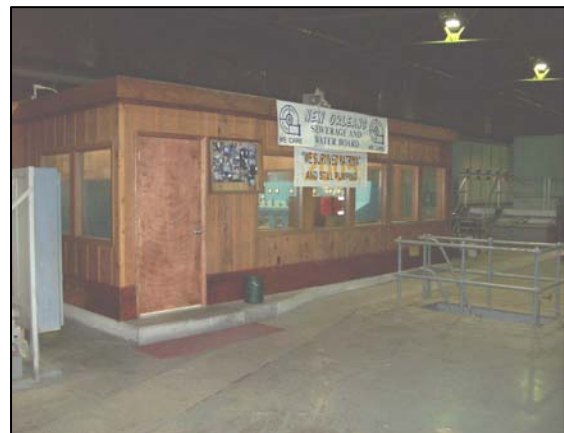
Photograph 4. Operator control room at DPS 1. Photo taken on April 22, 2008.
