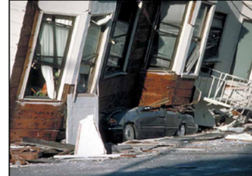
Structural failure and sinking of an apartment building in San Francisco Marina District, 1989 Loma Prieta earthquake (Nakata, 2002).
