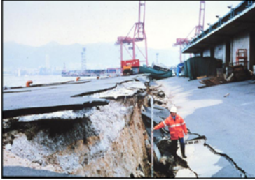
Extensive liquefaction damage to port facilities in 1995 Kobe, Japan, earthquake, due to tilting and displacement of quay walls, caused a US $10 billion loss (Iai, 1996).
