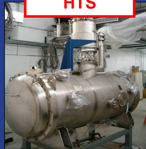
MP9 Clean Room
