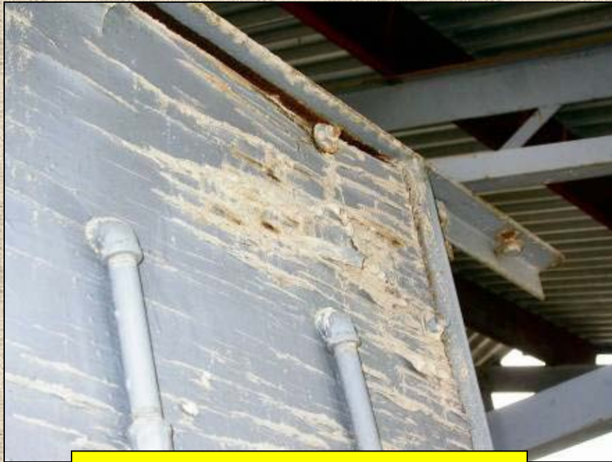
Deteriorating and delaminating
