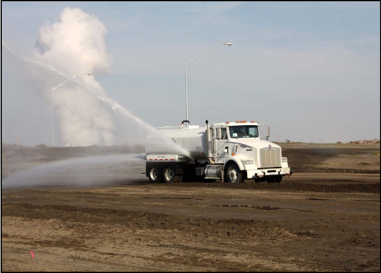
White Shield/Apollo began infrastructure work at the 618-10 Burial Ground last month and is scheduled to complete the project by February 2011. (Photo 5)
