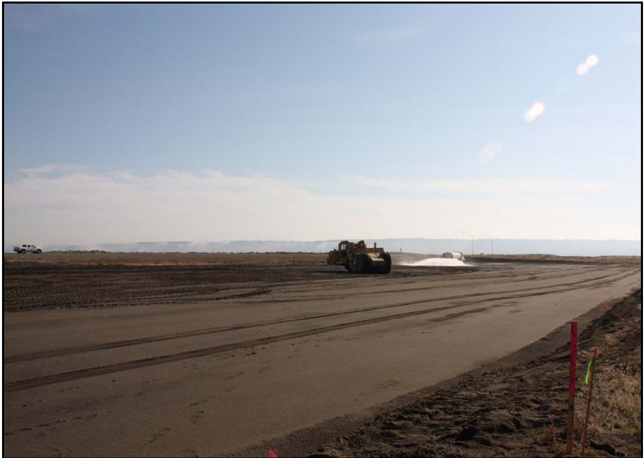
Washington Closure subcontractor White Shield/Apollo continues work on the new trailer complex site at the 618-10 Burial Ground. (Photo 4)
