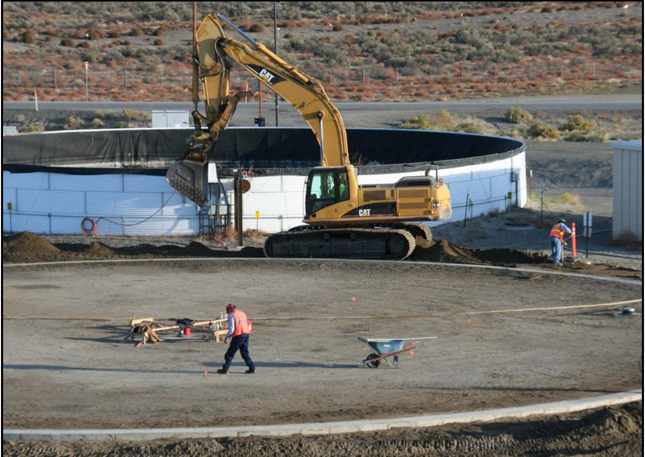
The project team completed backfill work around the foundation of leachate holding tank No. 4 at the Environmental Restoration Disposal Facility. Tank No. 2 (background) will be removed early next year. (Photo 3)
