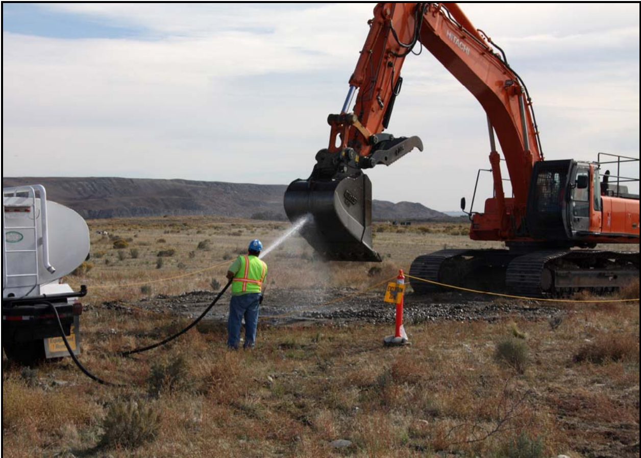
Washington Closure Hanford subcontractor Ojeda Business Ventures conducts potholing activities at 100-F-55. (Photo 6)
