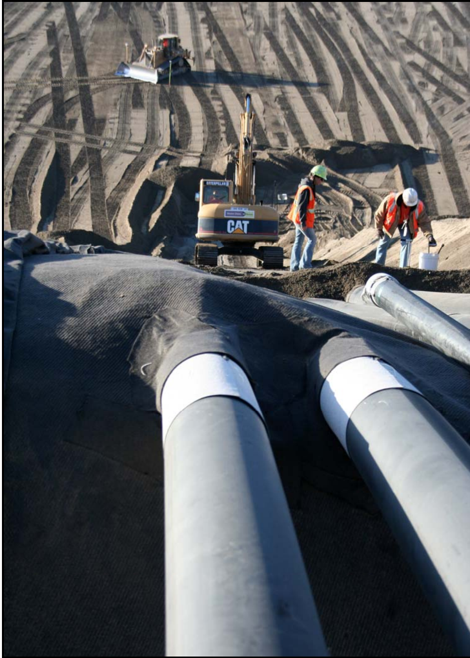
The secondary riser pipes from the sump to the crest pad building were installed in super cell 9 at the Environmental Restoration Disposal Facility. (Photo 2)
