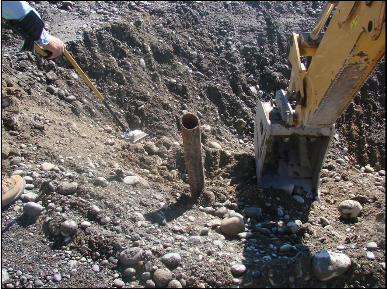
Confirmatory sampling was performed on Site 100-D-83. The site contains a compilation of underground pipelines that transported treated water.
