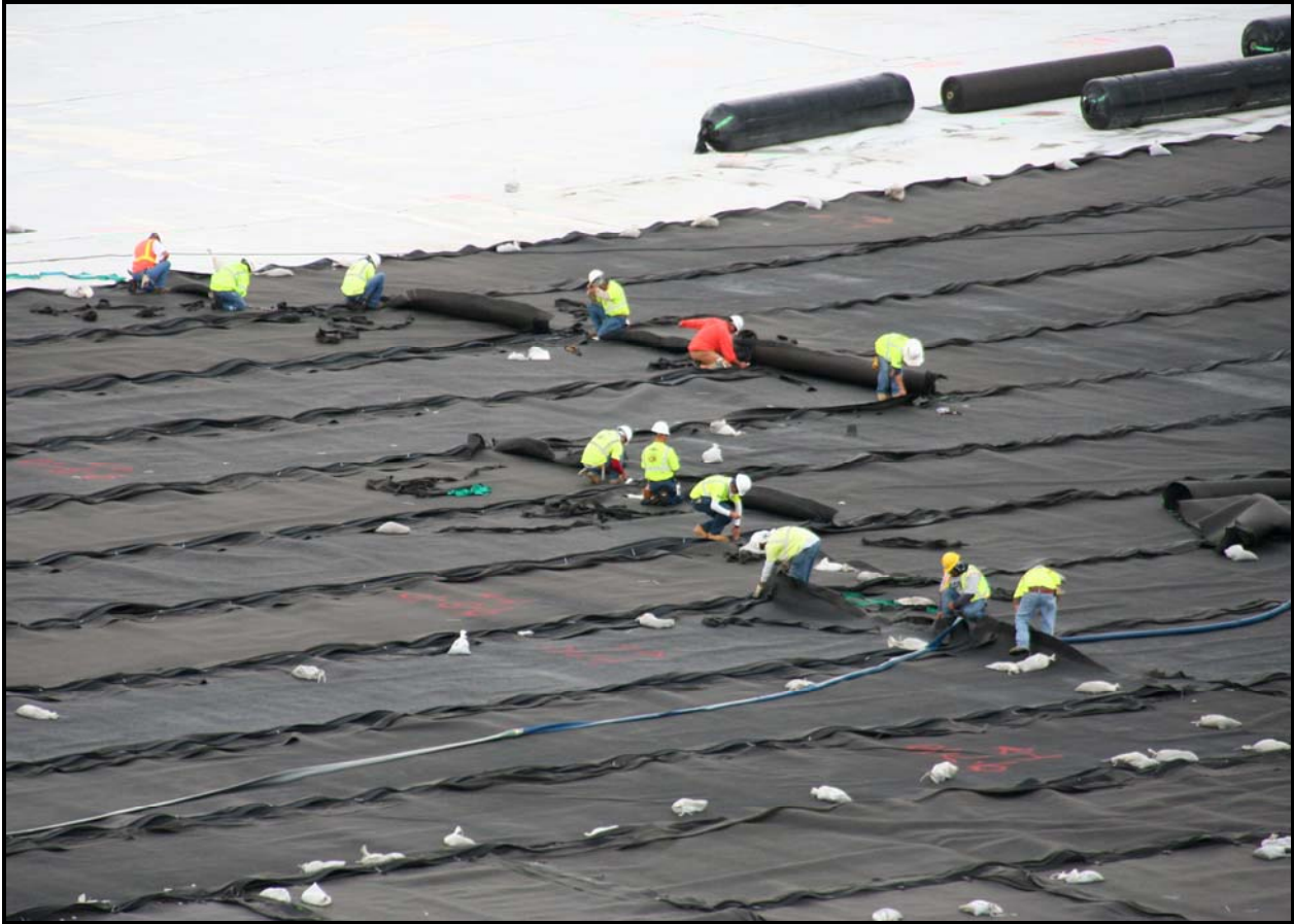
Work continues on the installation of the geocomposite layer in super cell 10 at the Environmental Restoration Disposal Facility.
