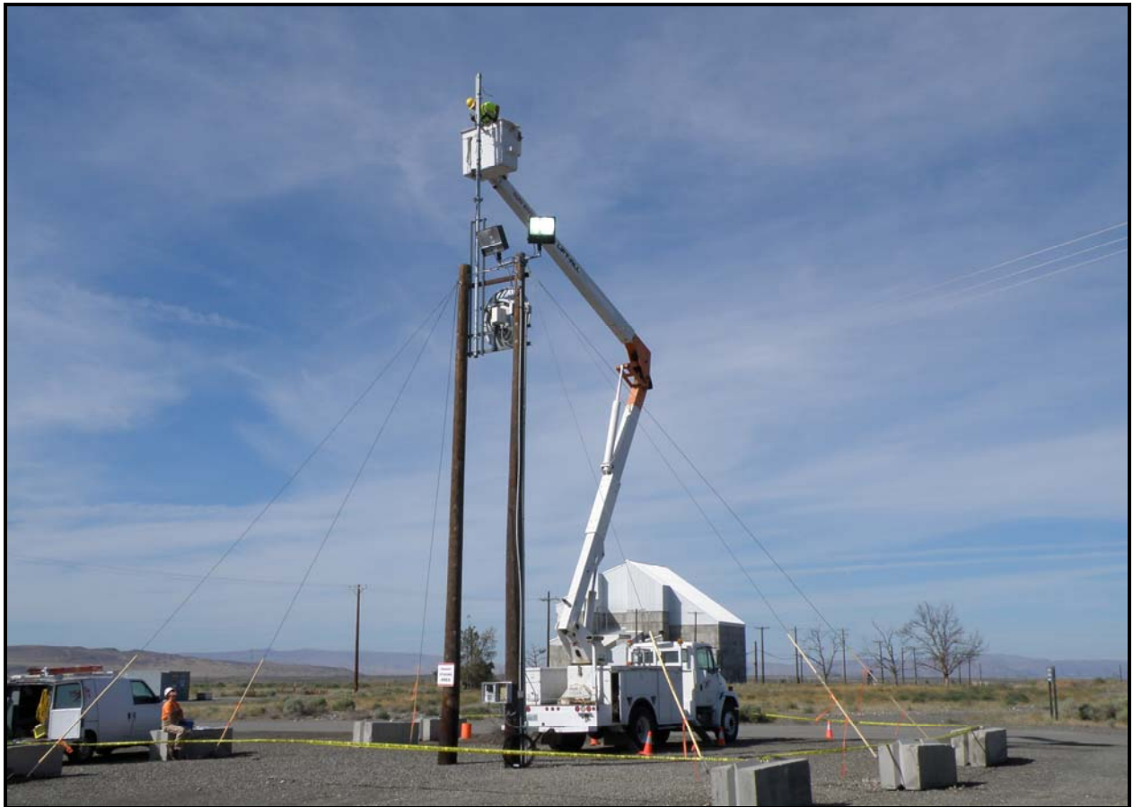
Workers install microwave connection to provide communications for 100-F Area. Washington Closure Hanford subcontractor Ojeda Business Ventures is scheduled to begin remediation of 18 waste sites next week.
