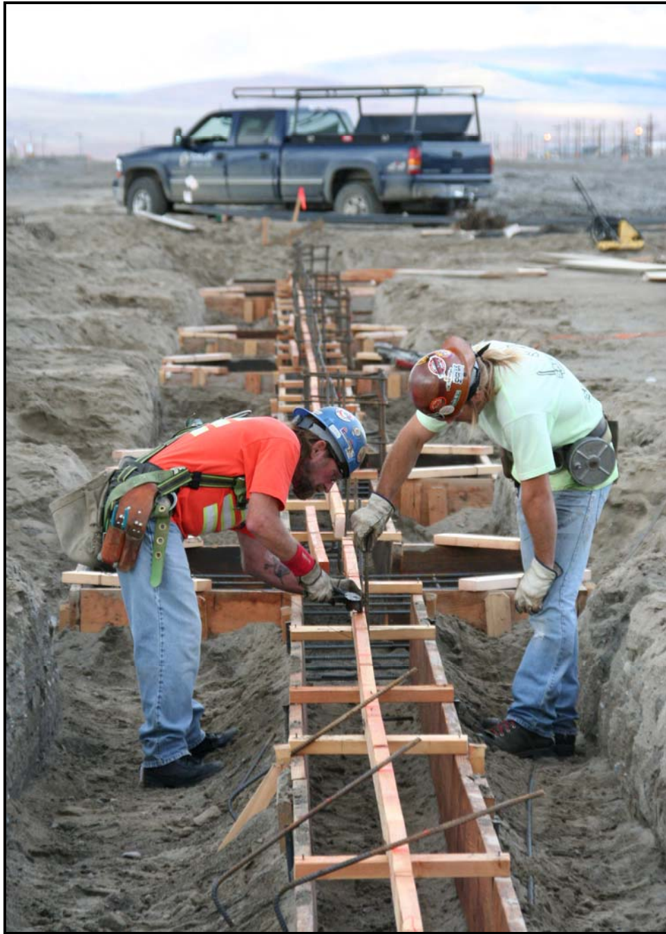
Workers install rebar in preparation for pouring the container maintenance facility's concrete foundation at the Environmental Restoration Disposal Facility.
