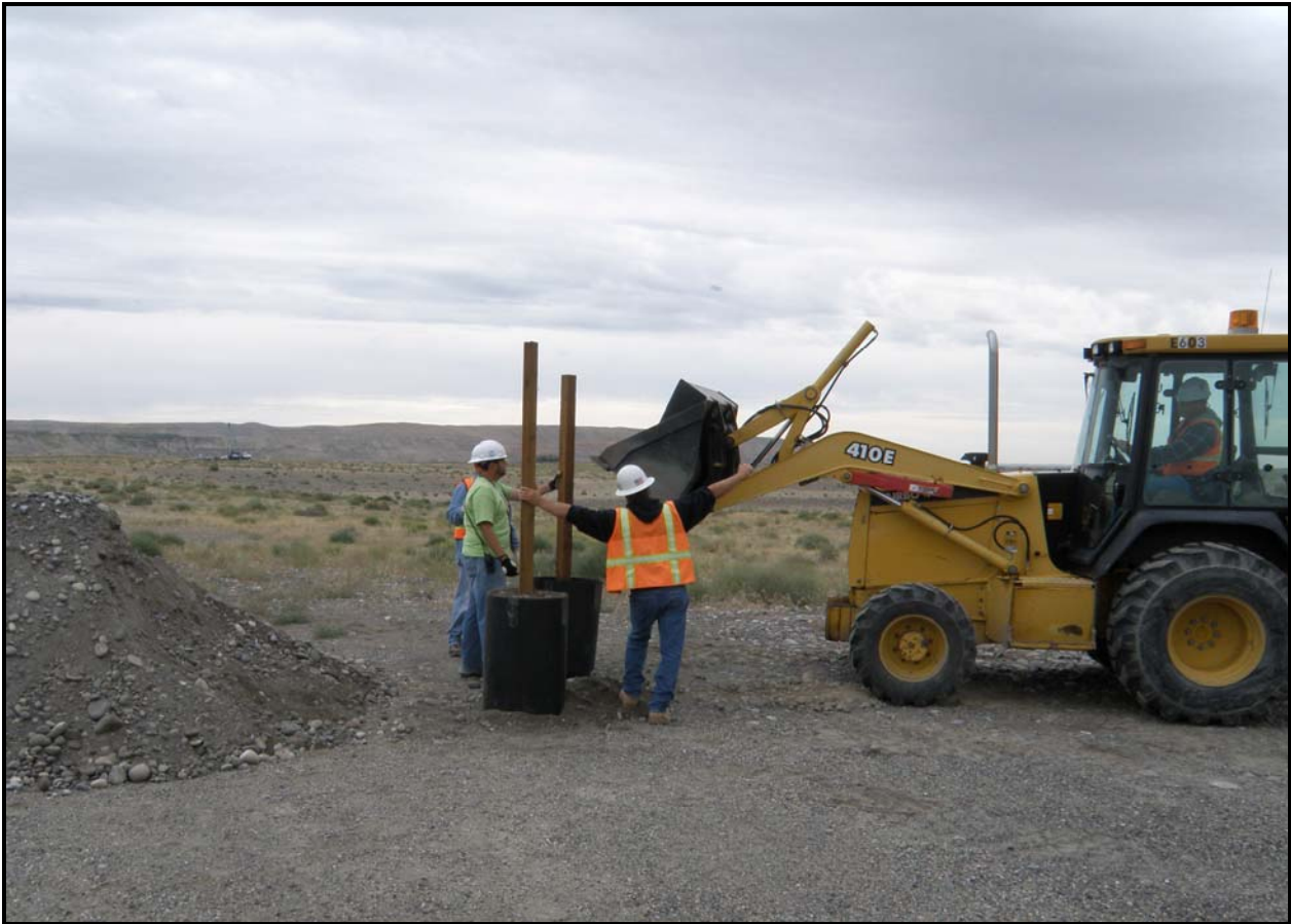
Workers prepare to install posts for signage in preparation of remediation at 100-F Area.
