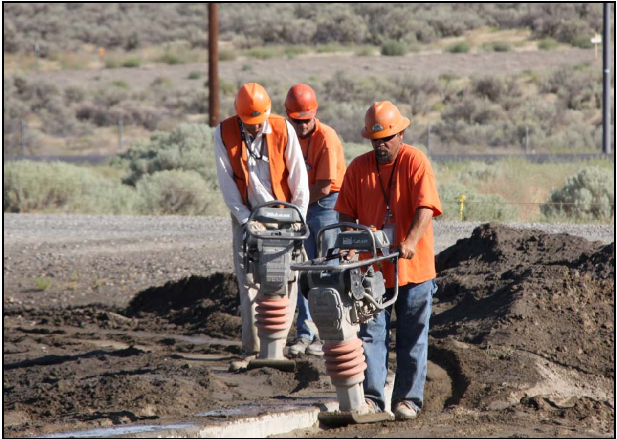
DelHur Industries personnel compact the area around the concrete foundation of the new leachate holding tank at the Environmental Restoration Disposal Facility.
