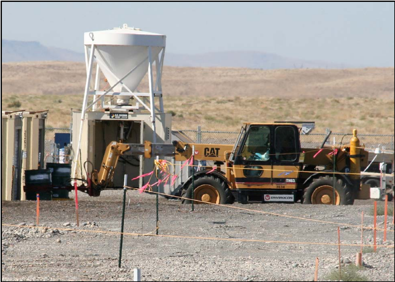
A telehandler transports a concreted drum to a mobile nondestructive assay system for processing at the 618-10 Burial Ground.
