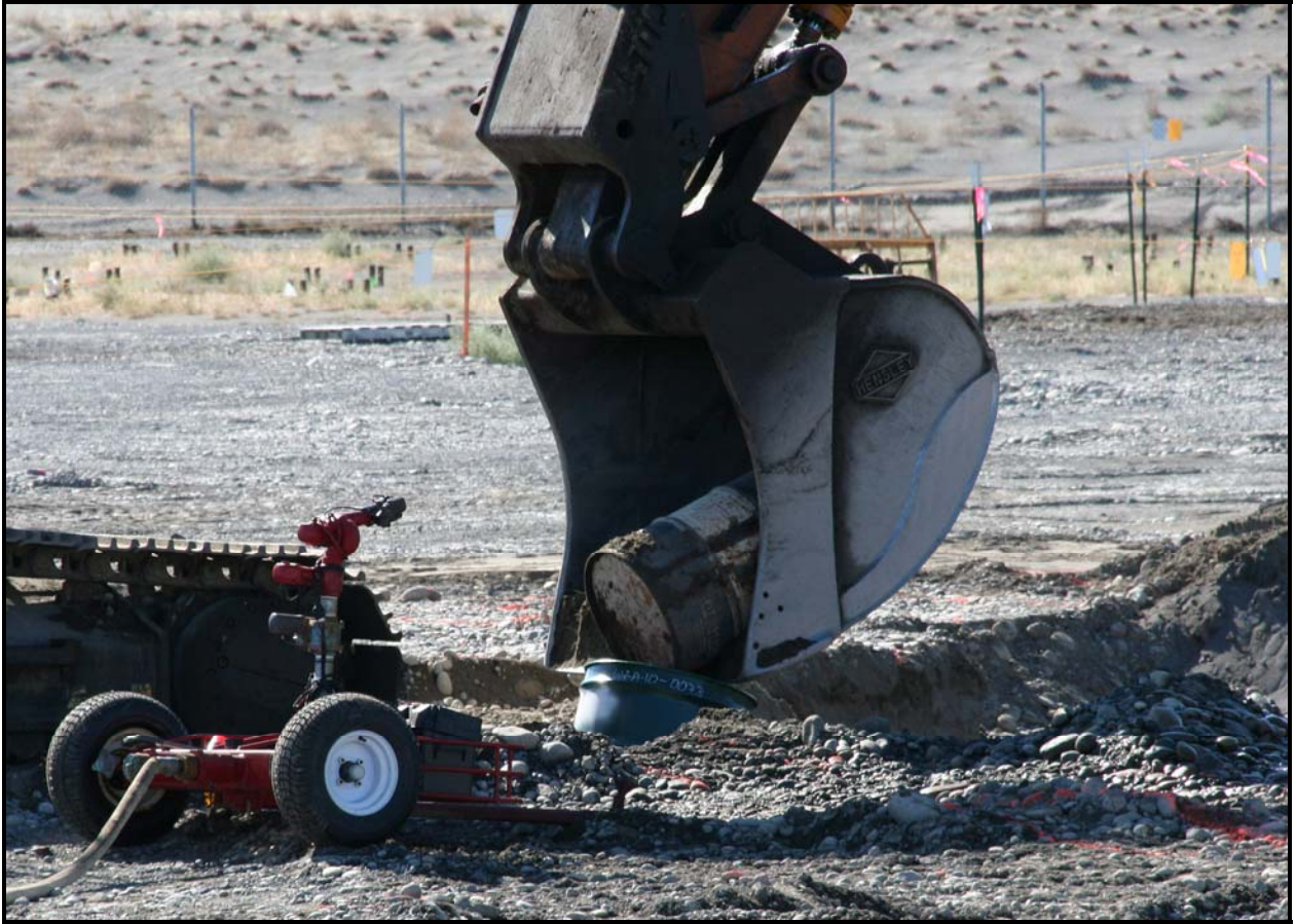
The primary excavator operator carefully places a concreted drum into a salvage container at the 618-10 Burial Ground.
