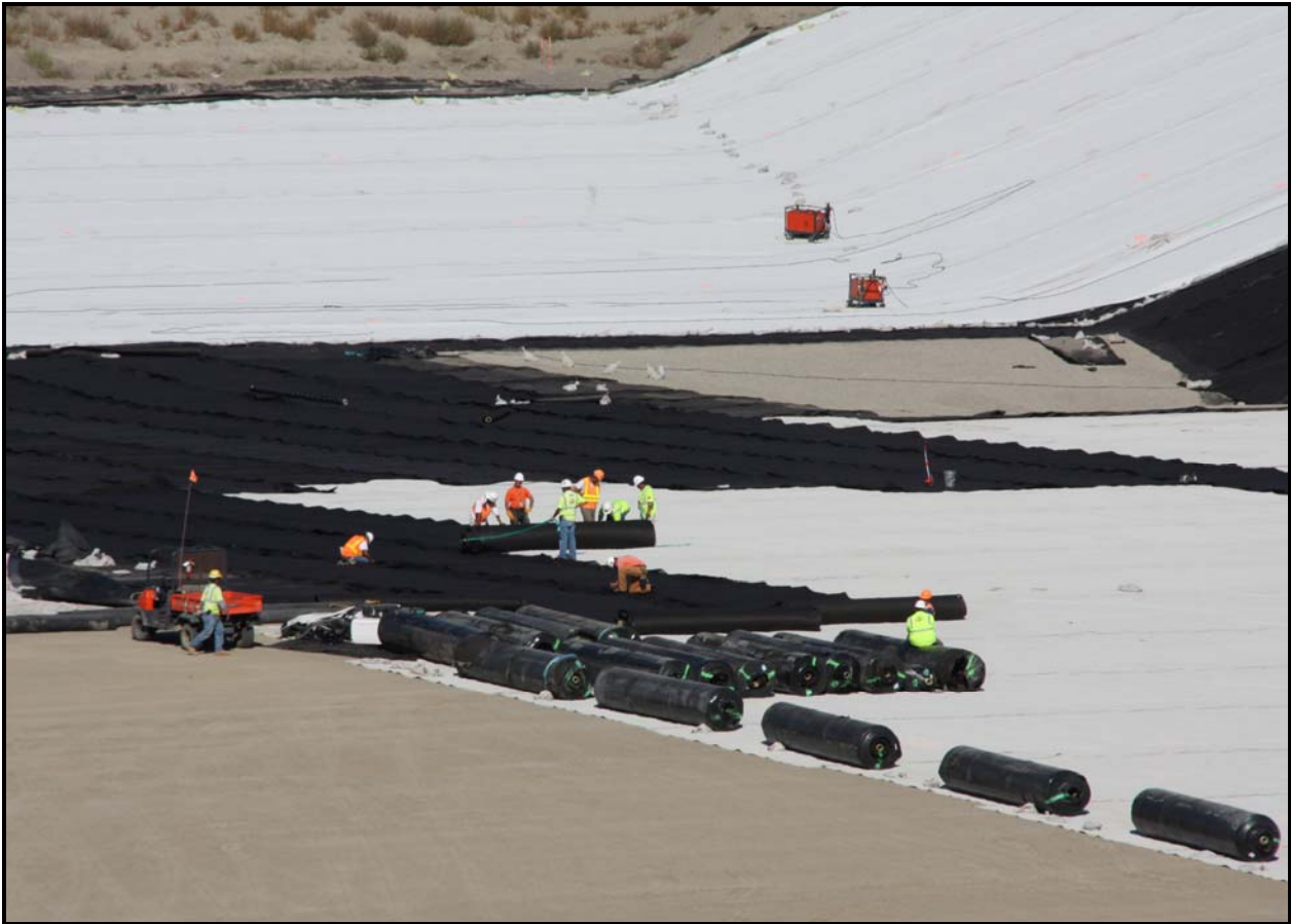
Workers from Environmental Specialties International install the geocomposite layer in super cell 9 at the Environmental Restoration Disposal Facility.
