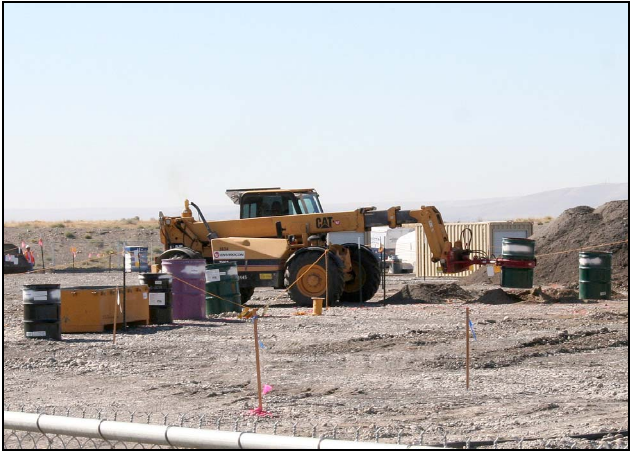
A telehandler picks up a concreted drum that was unearthed from a trench at the 618-10 Burial Ground.
