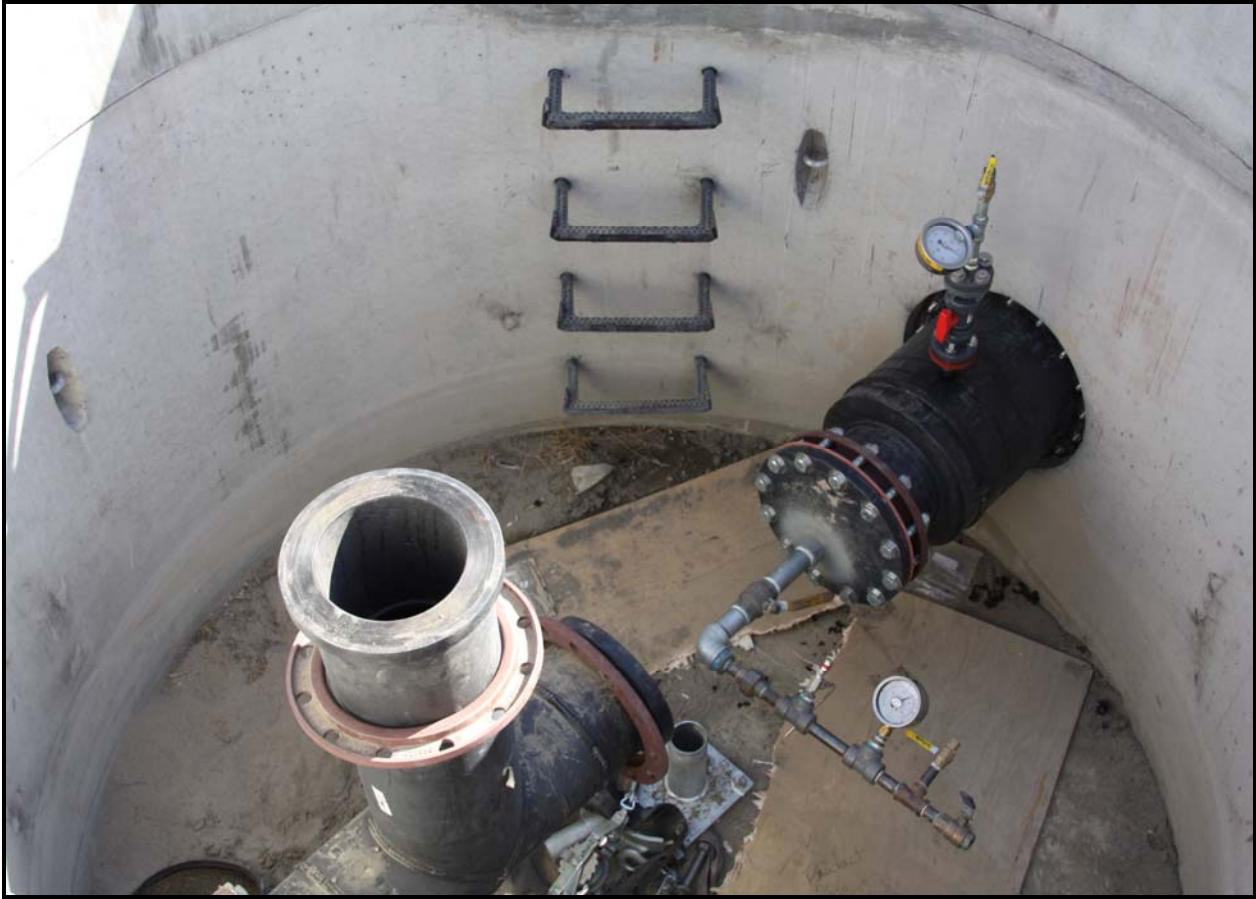
A look inside a manhole shows the leachate transmission line from the super cells to the leachate holding tank at the Environmental Restoration Disposal Facility.
