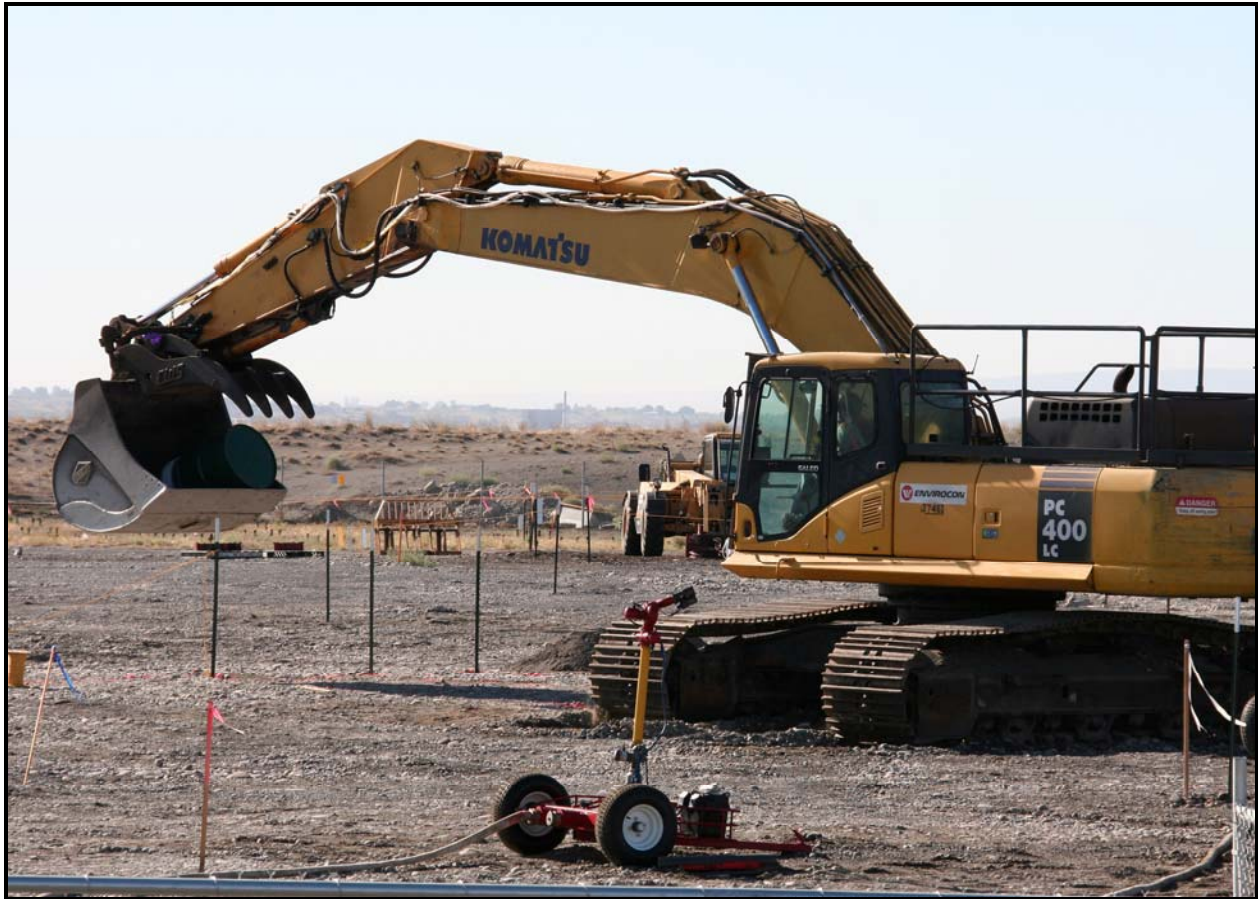
The primary excavator operator picks up an 85-gallon salvage container during intrusive characterization field operations at the 618-10 Burial Ground.
