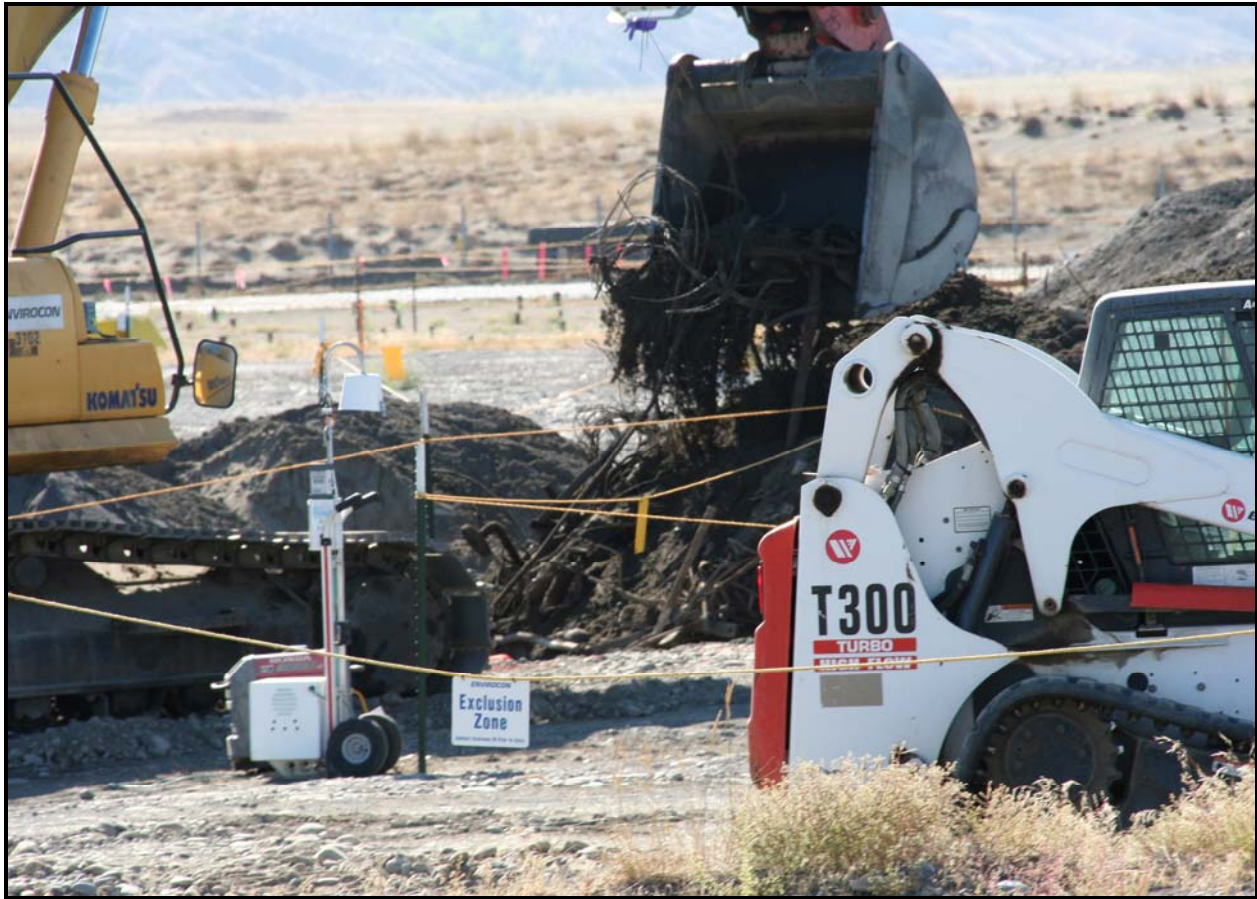
The secondary excavator clears debris from a trench at the 618-10 Burial Ground.
