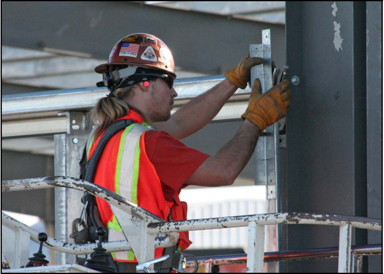
An ELRFowler employee constructs window frames at the equipment facility/operations center at ERDF. (Photo 2)
