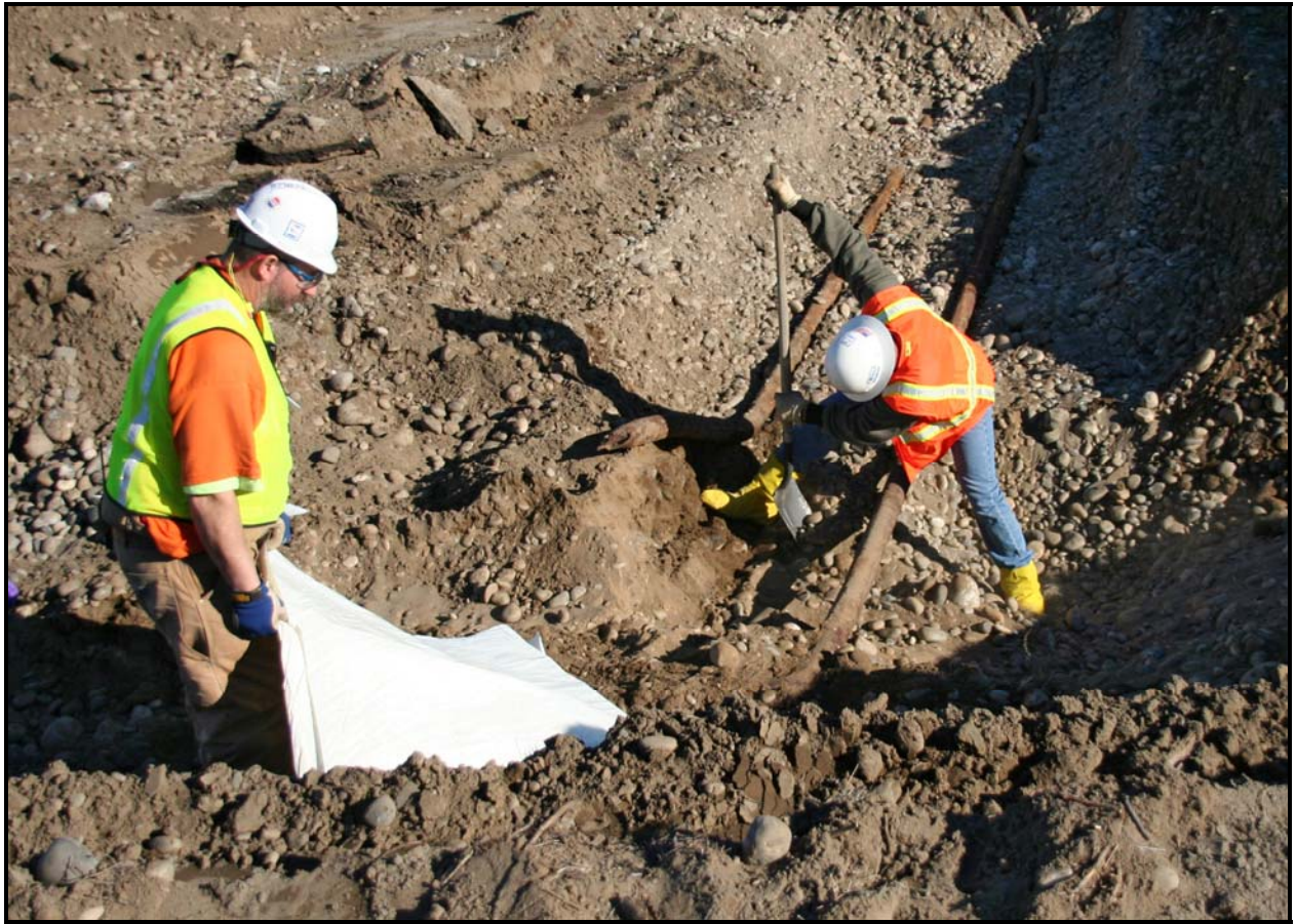
Ojeda personnel work to prepare a pipe for sampling at 100-F-26:7. (Photo 7)
