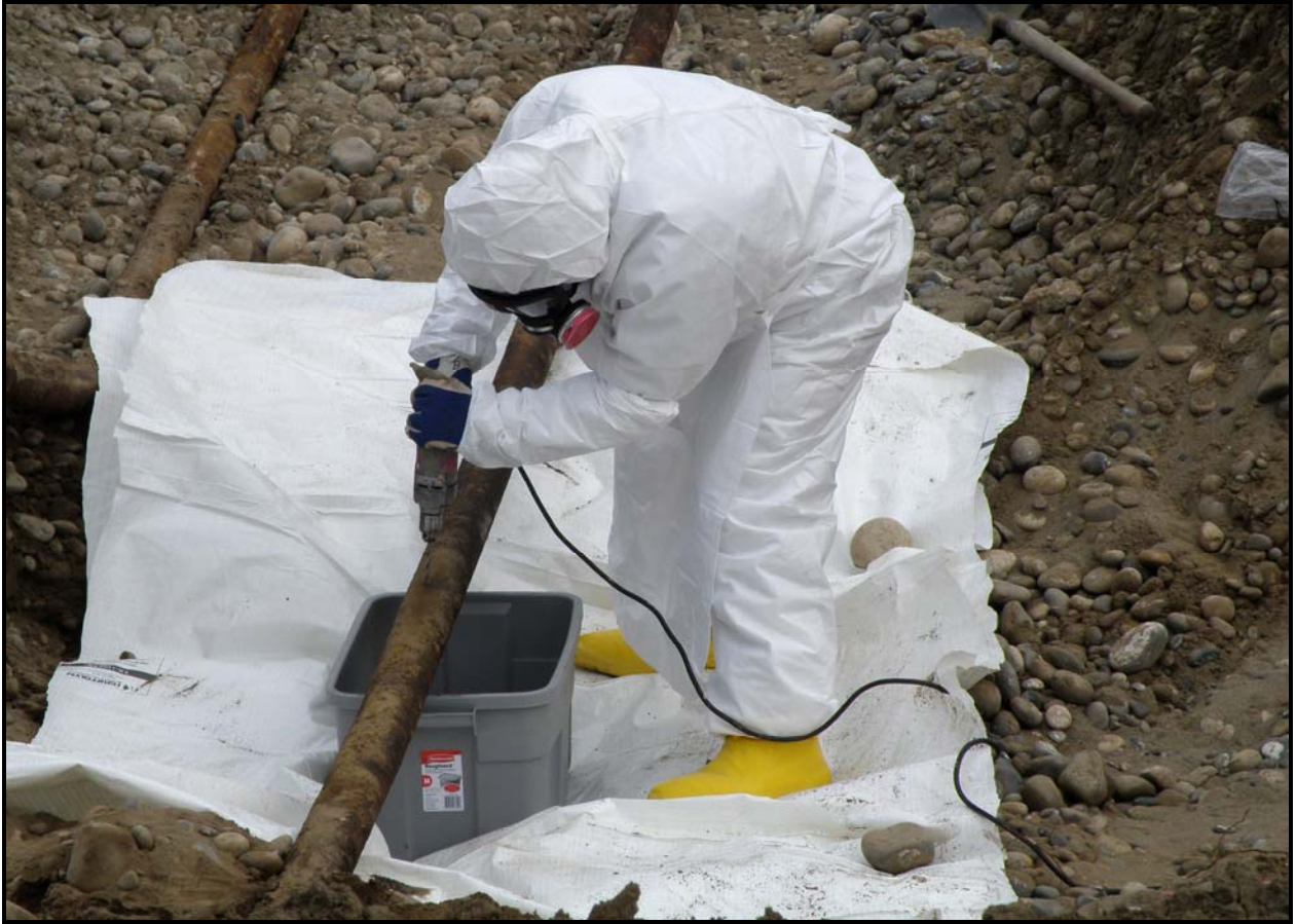
A worker uses a hot tap to drain a pipe for sample at 100-F-26:7. (Photo 8)
