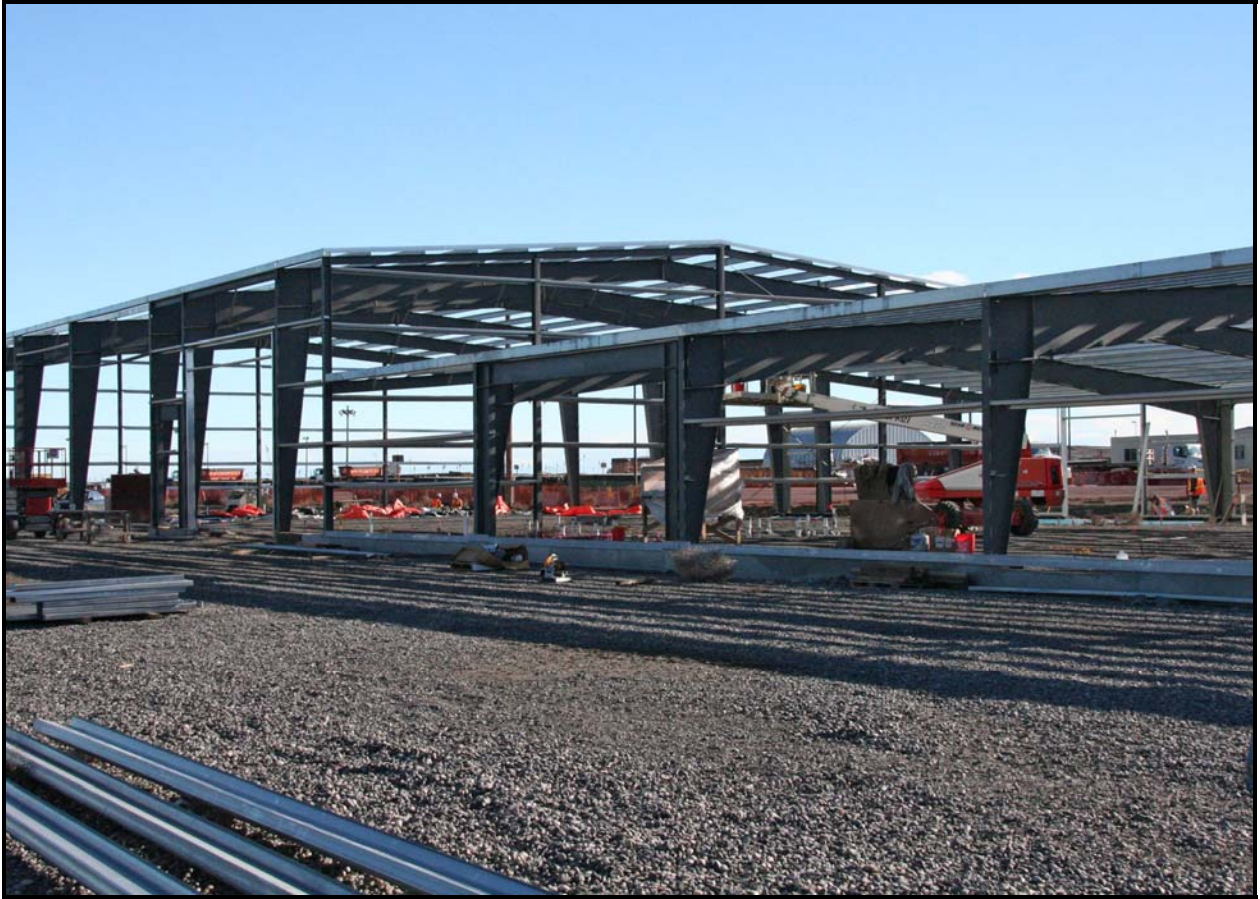
ELRFowler has completed erection of the structural steel of the equipment facility/operations center at ERDF. Work is under way to construct the window and door frames. (Photo 3)
