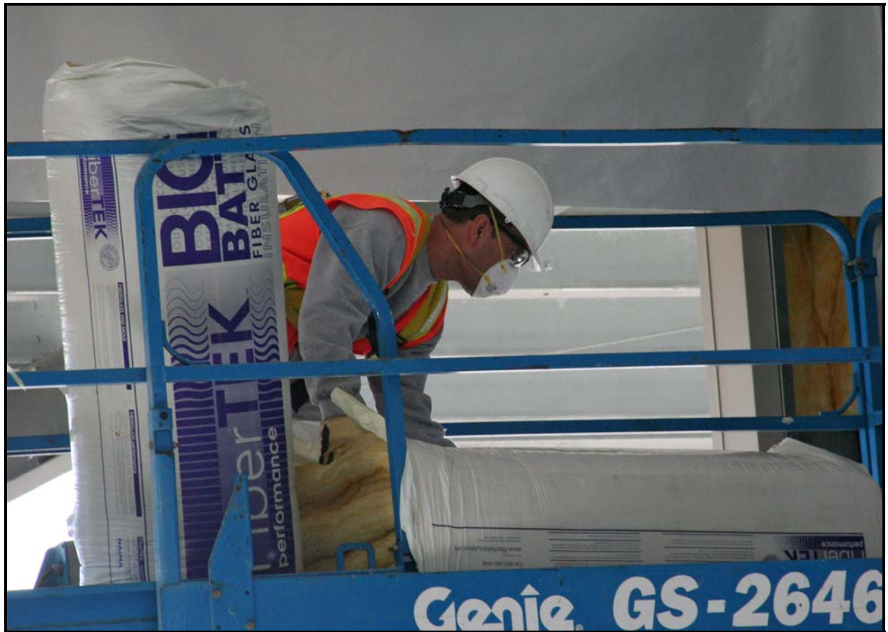
An employee with Washington Closure Hanford subcontractor ELRFowler installs insulation in the walls of the container maintenance facility at ERDF. (Photo 1)
