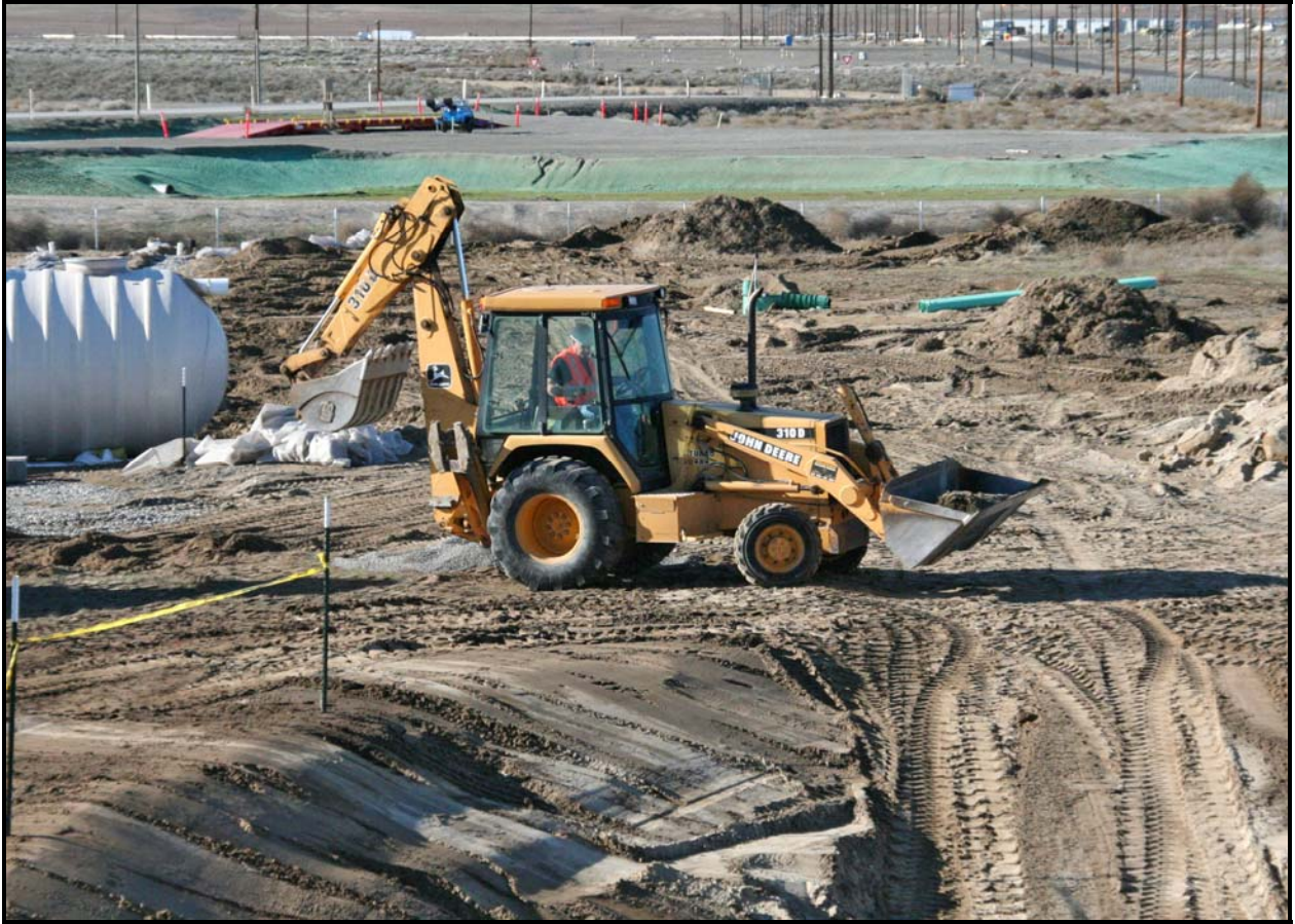
Washington Closure subcontractor DelHur Industries digs a hole for a new septic tank at ERDF. (Photo 4)
