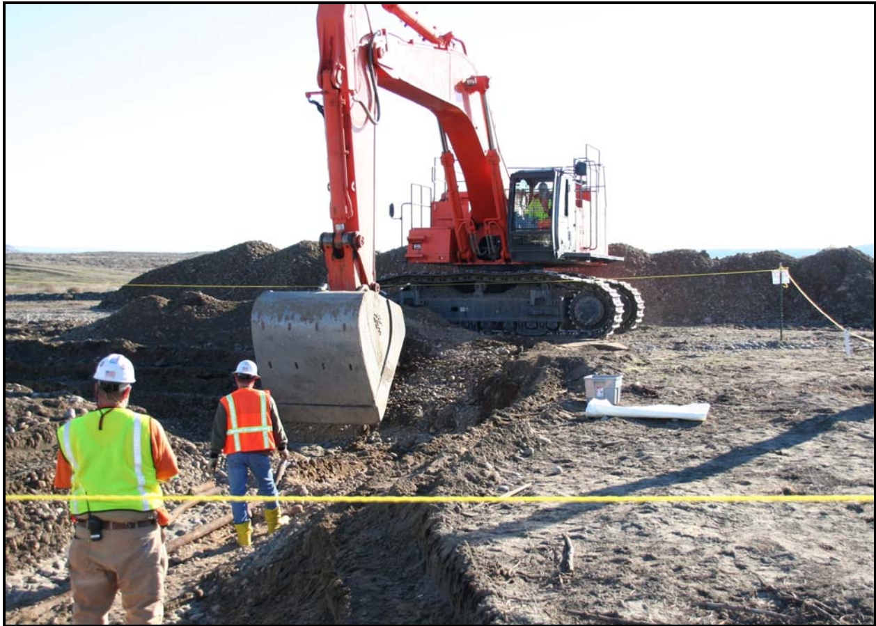
Washington Closure Hanford subcontractor Ojeda Business Ventures uncovers sodium dichromate and sodium silicate pipelines at 100-F-26:7. (Photo 6)
