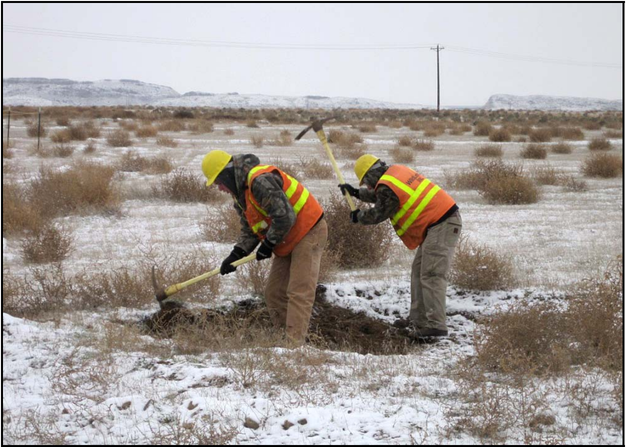
Workers revegetate Segment 1 site 600-346, one of four small fly-ash dump areas with metal debris. (Photo 8)
