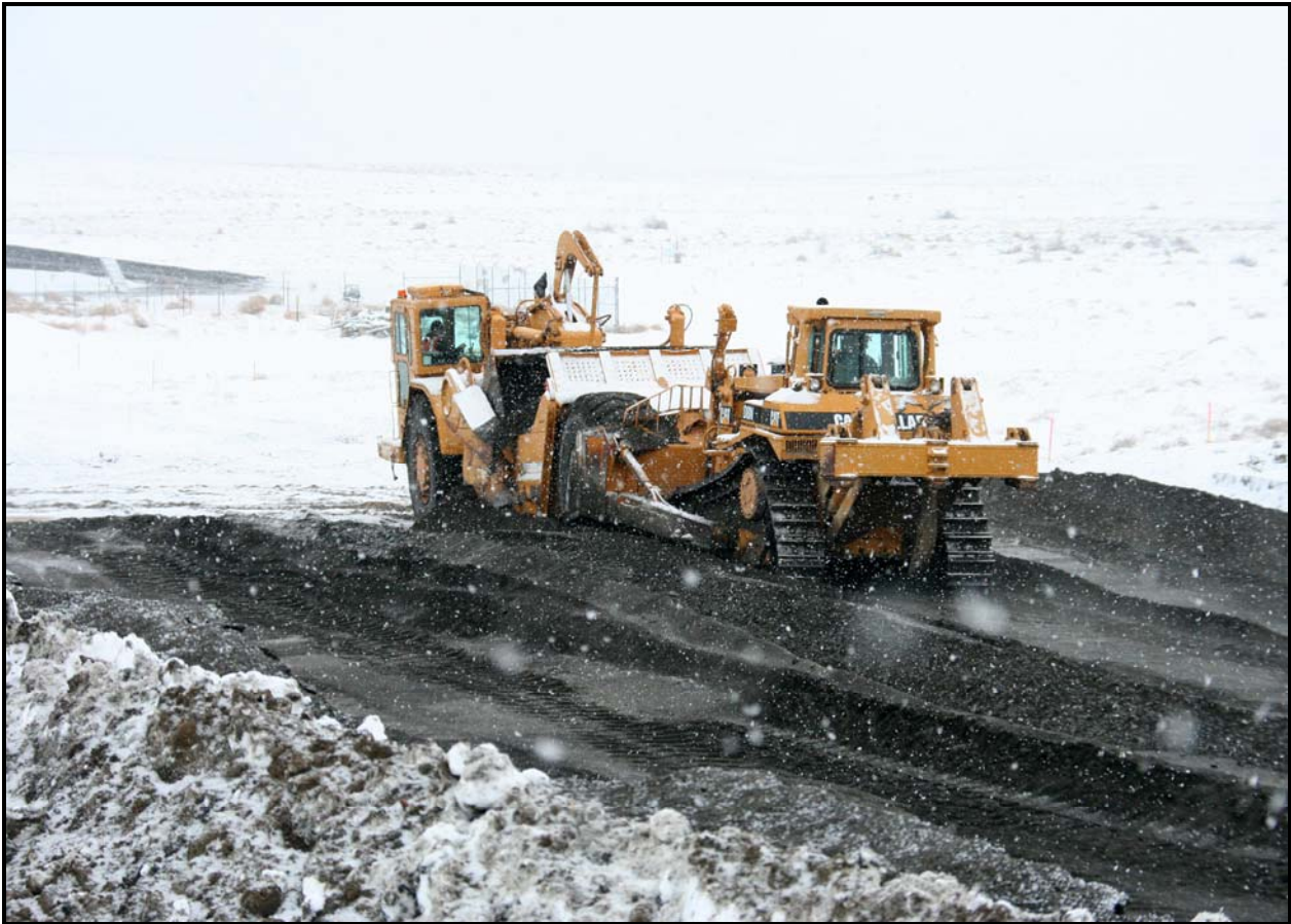
Washington Closure Hanford subcontractor White Shield/Apollo constructs roads at the 618-10 Burial Ground. The infrastructure work is scheduled to be completed in February. (Photo 5)
