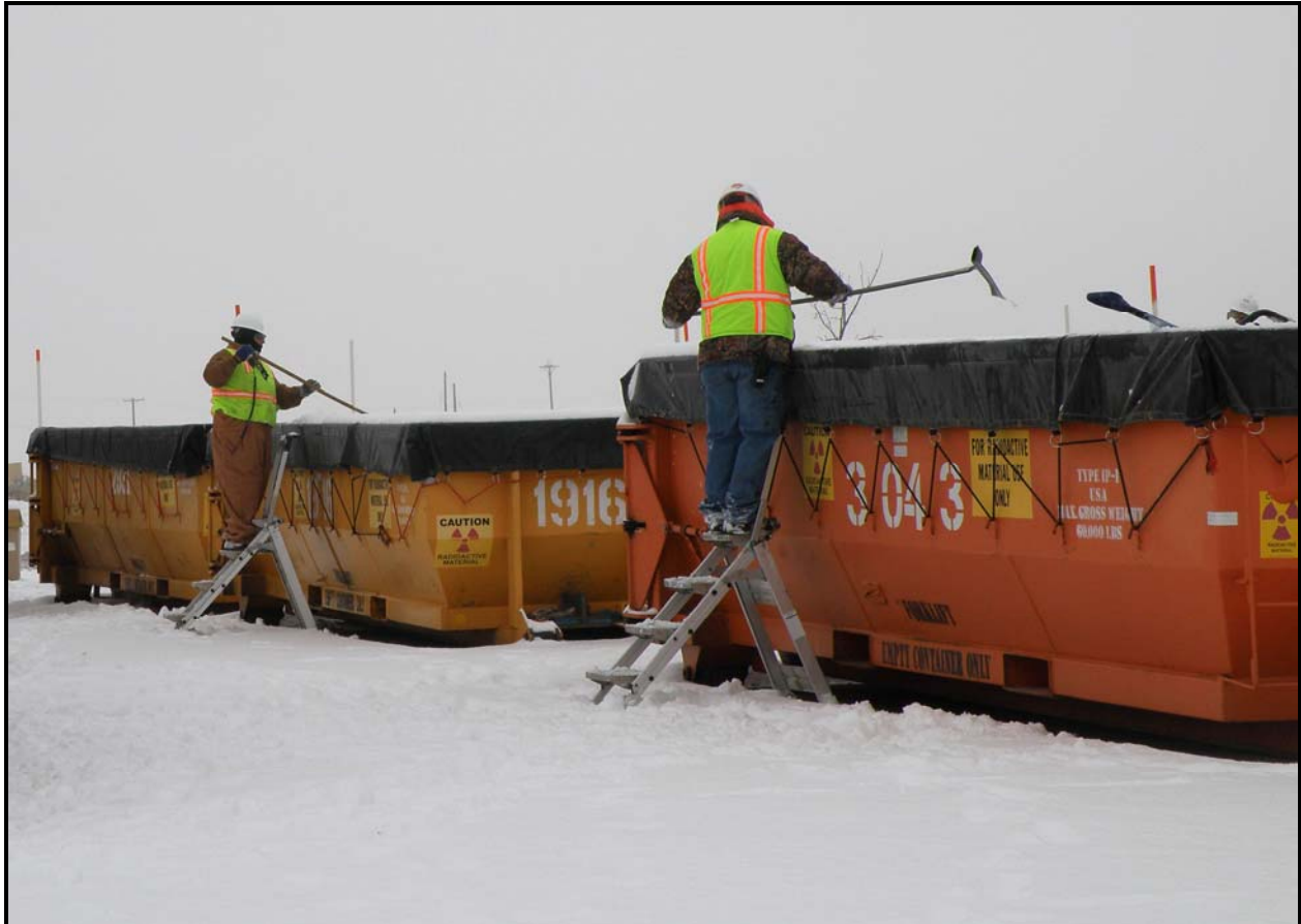
Workers brush off snow from waste containers at 100-F Area. Excavation and loadout activities continued at sites 100-F-47 and 100-F-48. (Photo 6)
