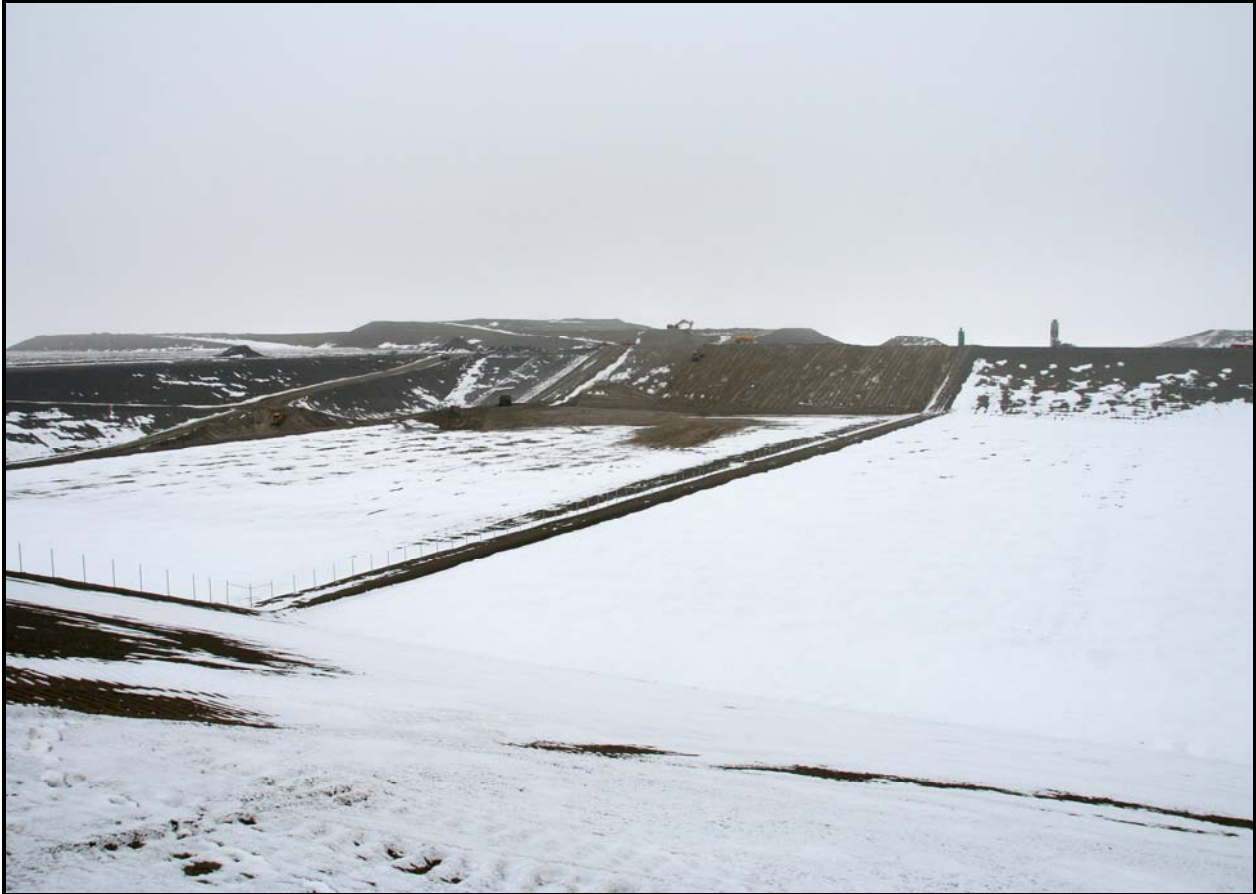
Washington Closure subcontractor TradeWind Services completed placement of the operations layers in super cells 9 and 10 at the Environmental Restoration Disposal Facility. (Photo 1)
