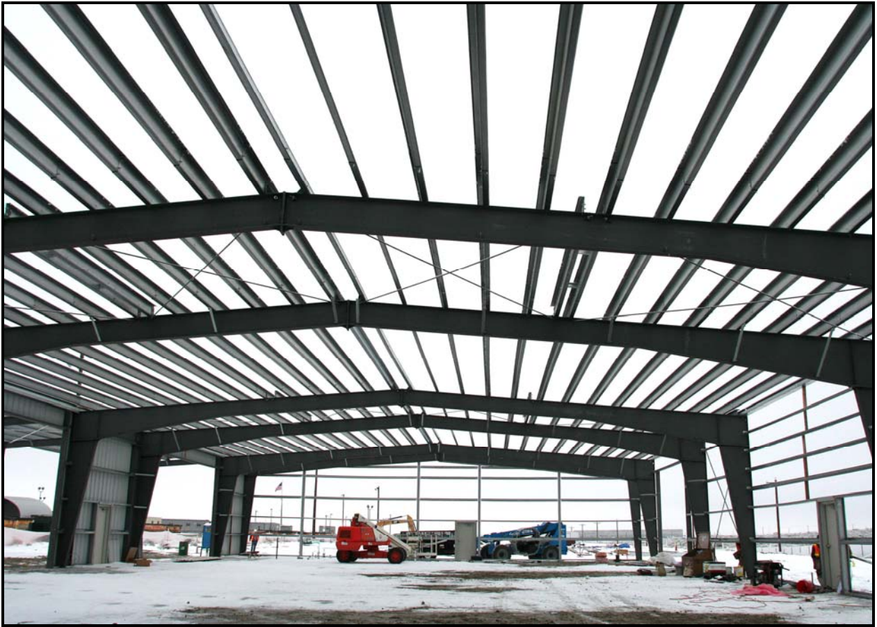
Washington Closure Hanford subcontractor Fowler General Construction erected the container maintenance facility's steel skeleton at the Environmental Restoration Disposal Facility. (Photo 2)
