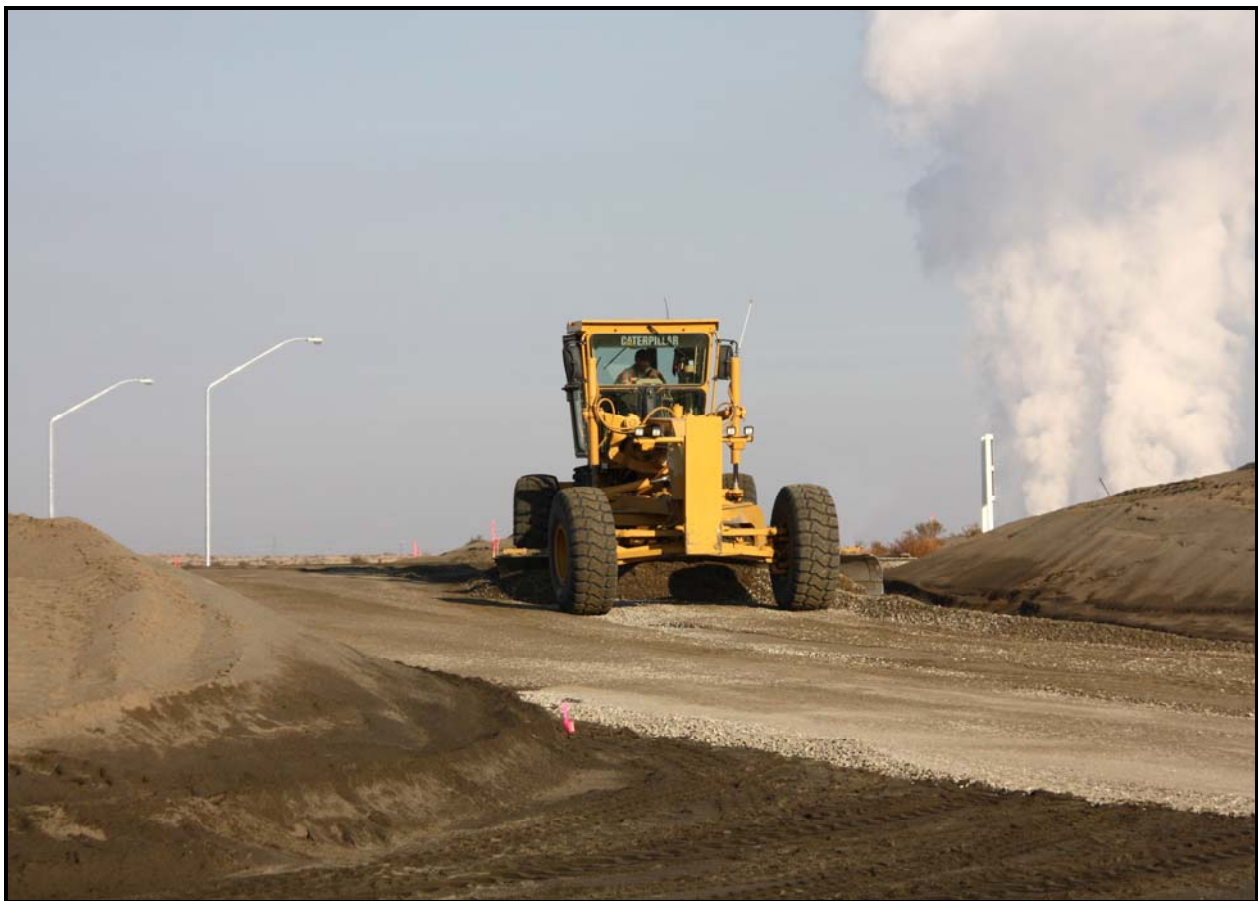
Washington Closure Hanford subcontractor White Shield/Apollo prepares to spread gravel on the office trailer site at the 618-10 Burial Ground. (Photo 6)
