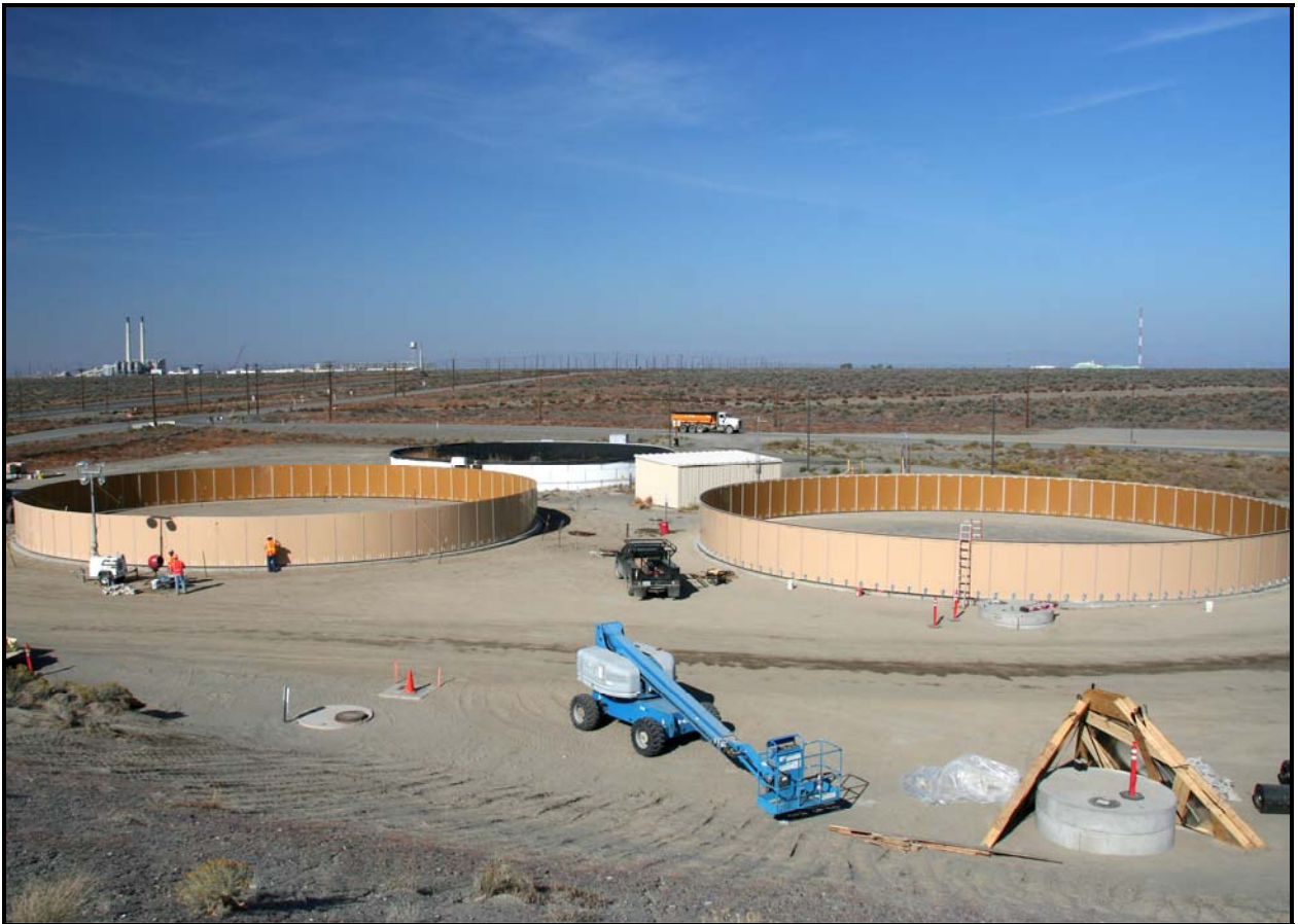
The new replacement tanks each will have a capacity of 425,000 gallons, over 150,000 gallons more than the original tanks. (Photo 2)
