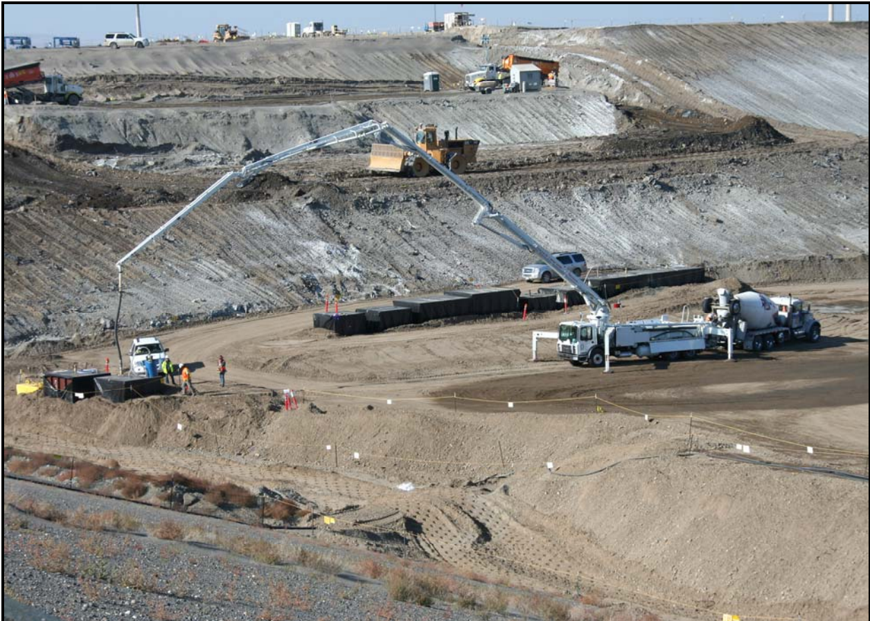
A pump truck provides concrete for grouting two hot cells from the 327 Building. The pump truck will support the new batch plant at the Environmental Restoration Disposal Facility. (Photo 5)
