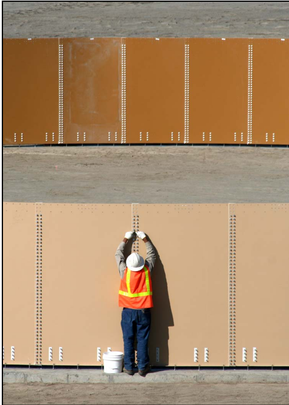
A worker from Washington Closure Hanford subcontractor DelHur Industries assembles the sidewalls for one of the two new leachate storage tanks at the Environmental Restoration Disposal Facility. (Photo 3)
