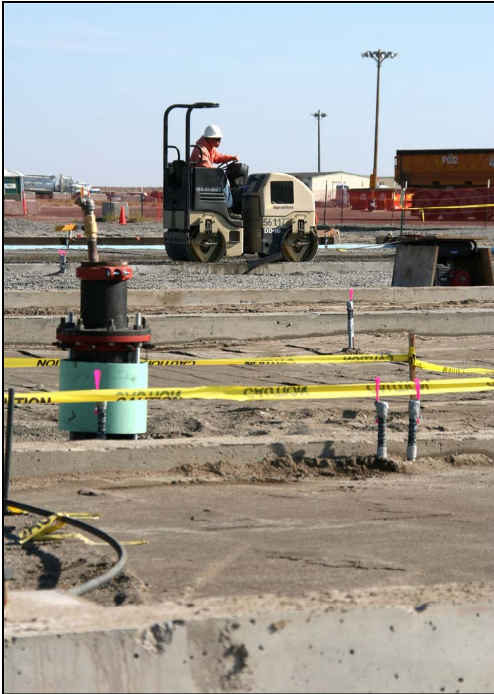
Washington Closure Hanford subcontractor Fowler General Construction installs underground utilities at the container maintenance facility. (Photo 4)
