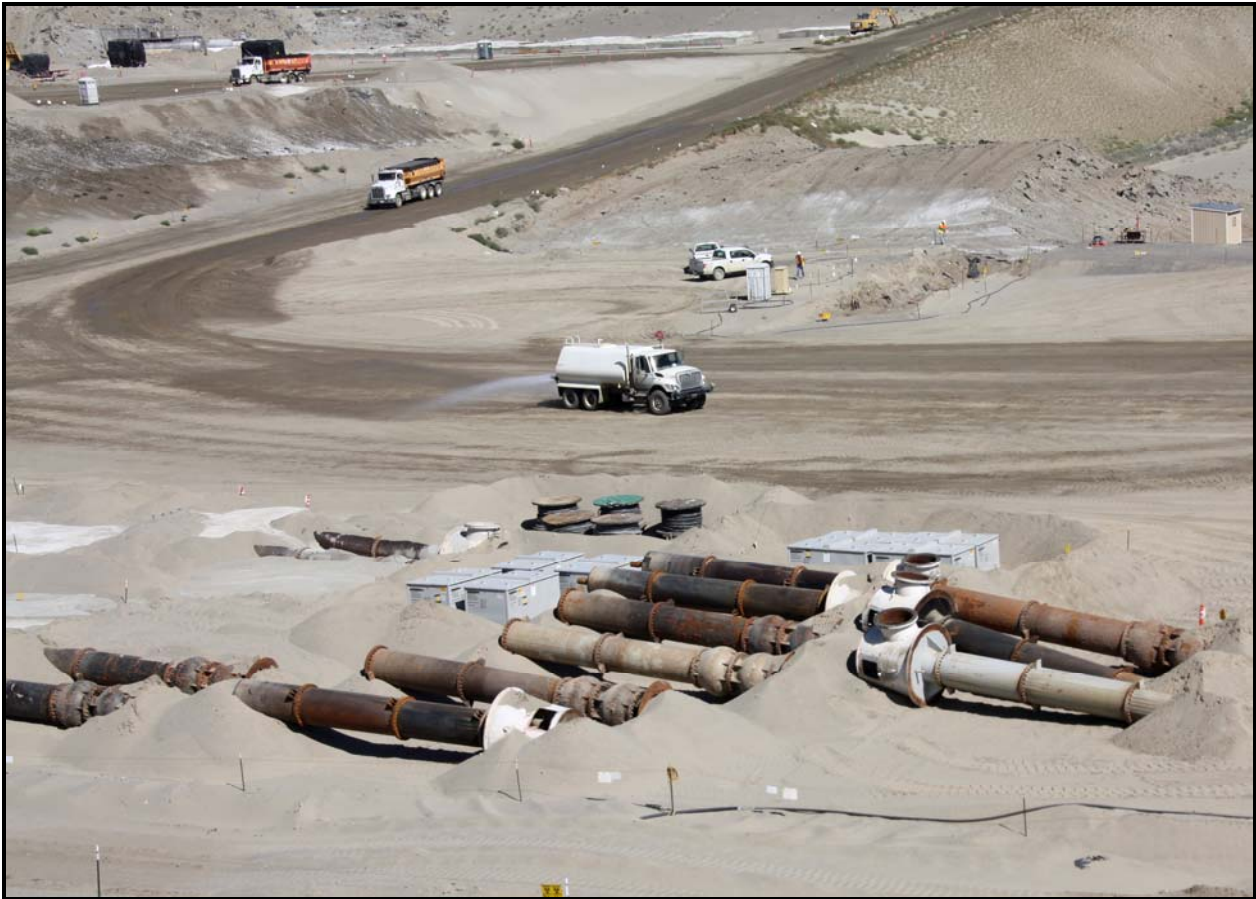
Pumps from the water intake structures at K Area are being disposed in super cell 9 at the Environmental Restoration Disposal Facility. (Photo 2)
