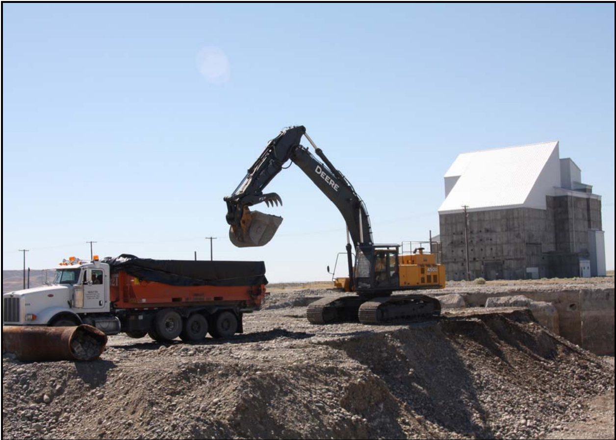
Washington Closure Hanford subcontractor Ojeda Business Ventures continues to excavate and load out concrete and underlying soil at 100-F-57. (Photo 6)
