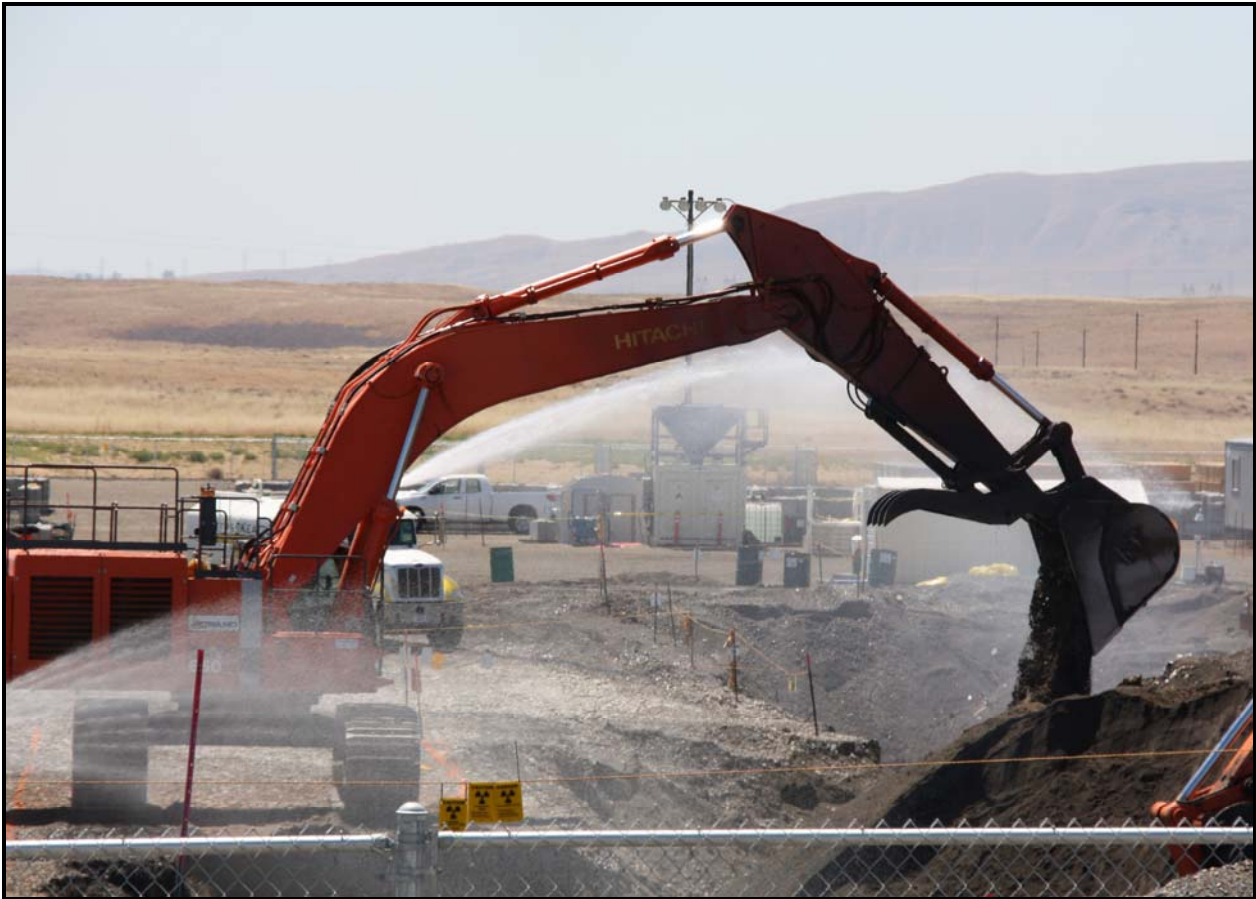
Washington Closure Hanford has encountered concreted drums and numerous bottles on the north side of the 618-10 Burial Ground. (Photo 4)
