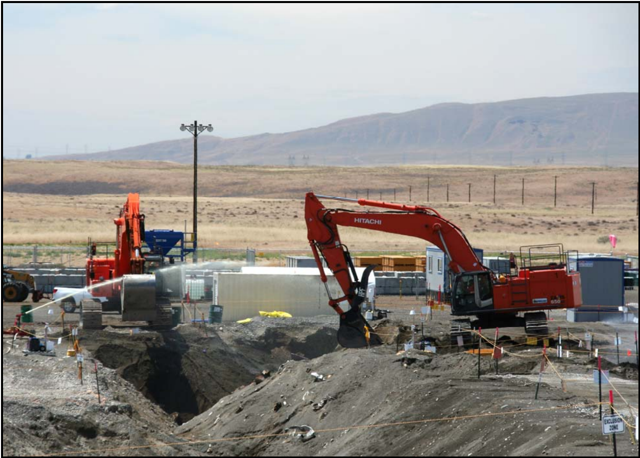
Washington Closure continues trench excavation of the 618-10 Burial Ground. So far, several concreted drums and other containers that contain uranium have been found. (Photo 4)
