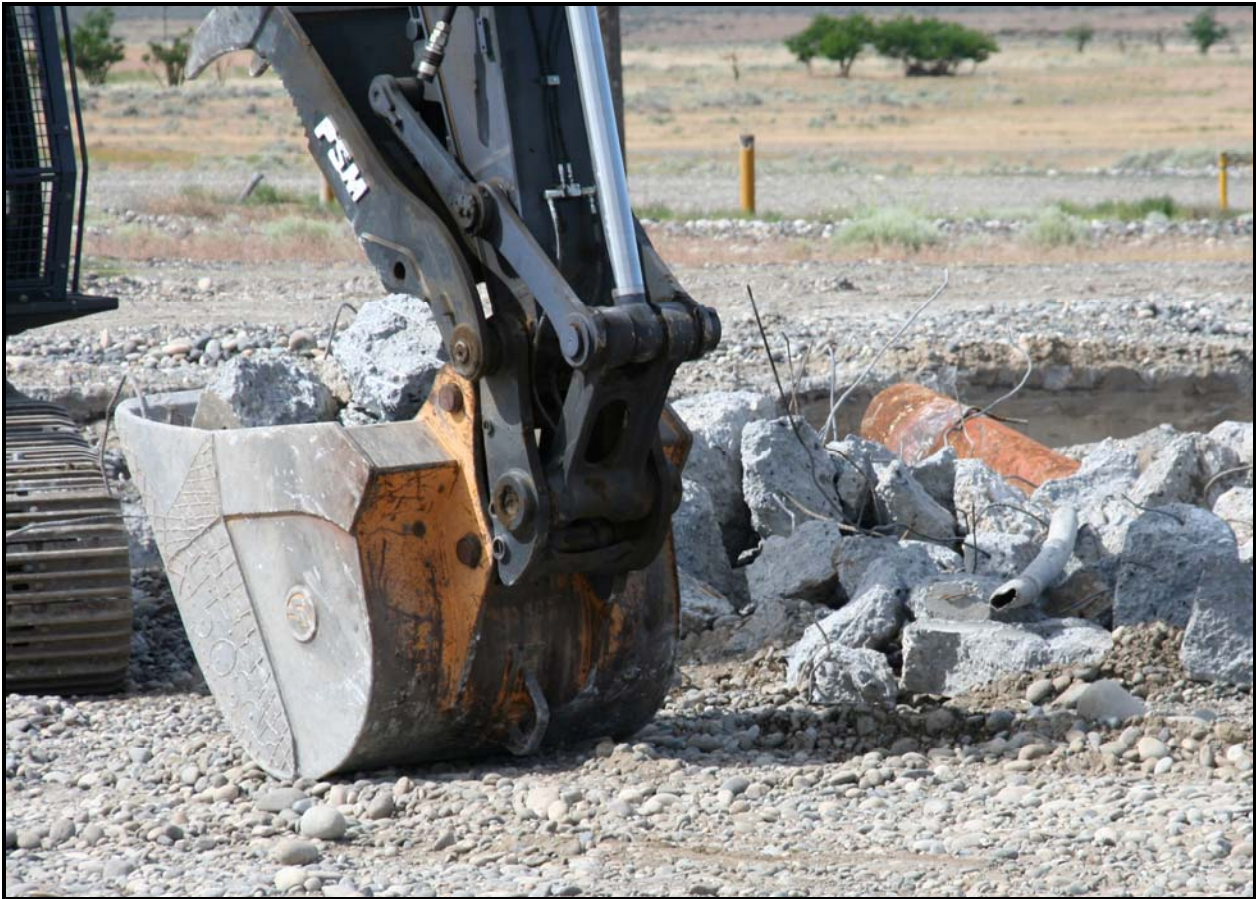
The stained concrete and underlying soil at 100-F-57 contains hexavalent chromium. (Photo 7)
