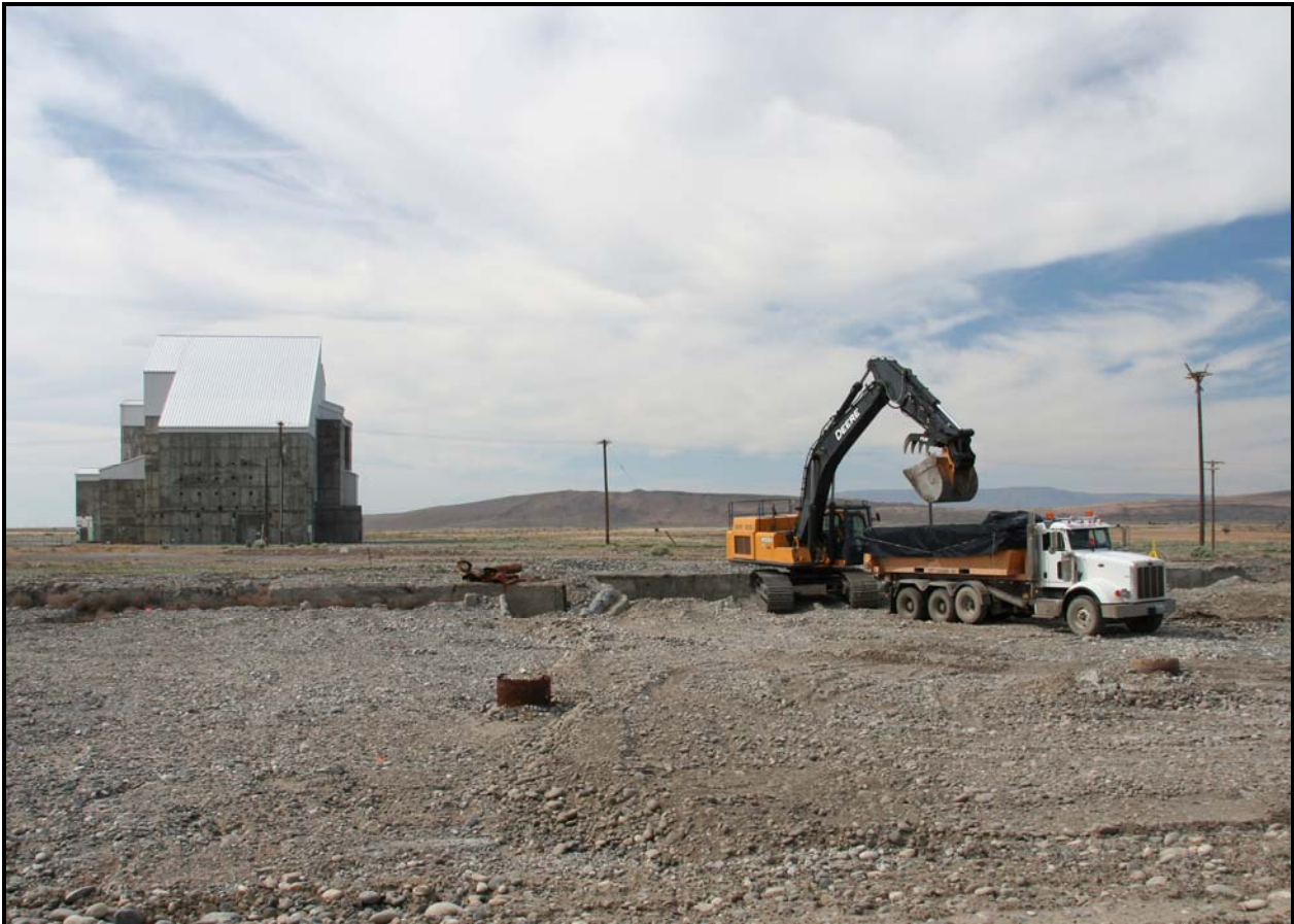
Washington Closure Hanford subcontractor Ojeda Business Ventures continues excavation and loadout of concrete at 100-F-57. (Photo 6)
