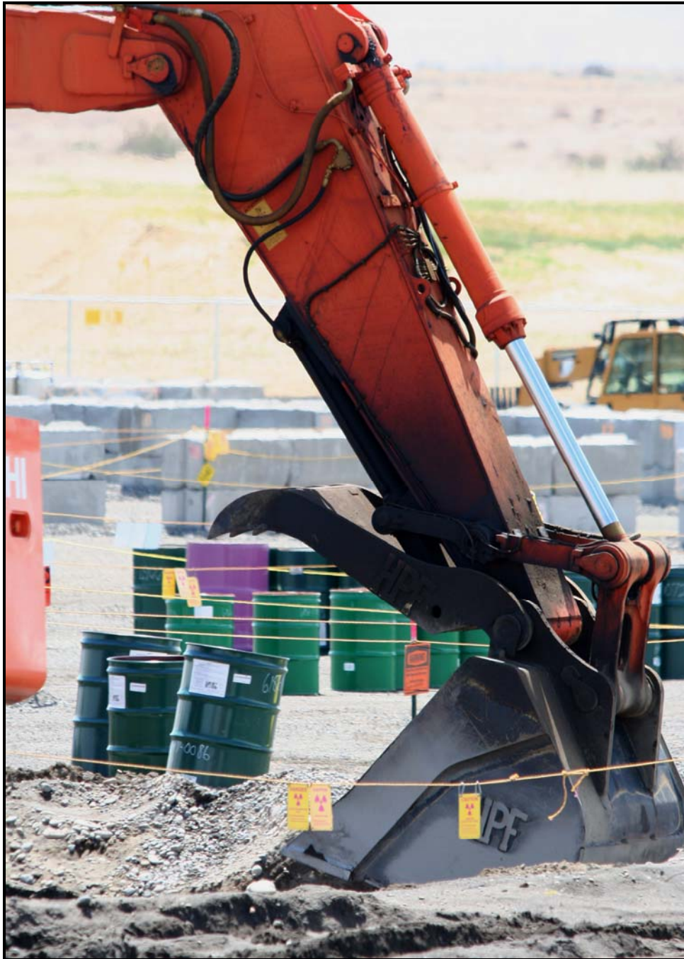
Washington Closure is working on the north and south sides of the 618-10 Burial Ground. (Photo 5)
