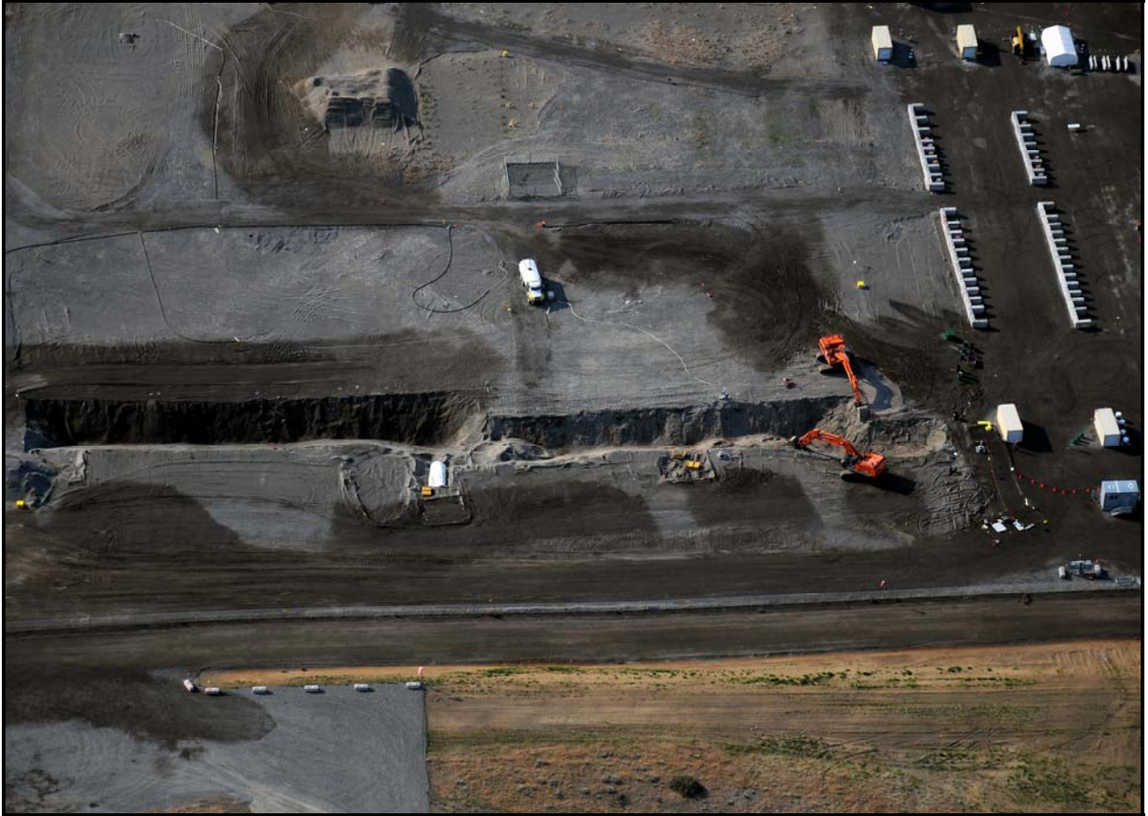
An aerial photo taken in late June shows trench excavation in the north section of the 618-10 Burial Ground. (Photo 3)
