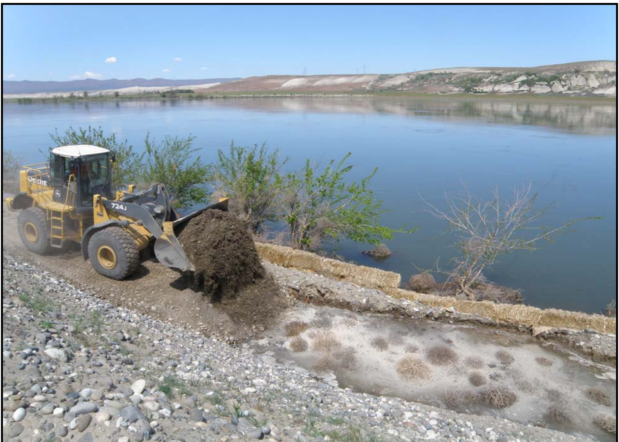
Washington Closure Hanford subcontractor Ojeda Business Ventures backfills site 100-F-45 to protect it from the Columbia River. (Photo 9)
