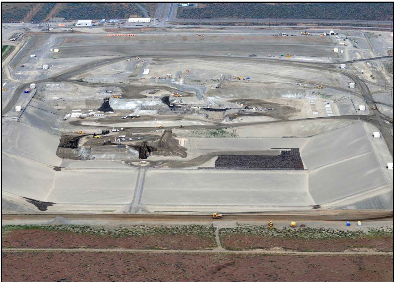
Super cell expansion increased the capacity of the Environmental Restoration Disposal facility to 16.4 million tons of waste material. Construction was completed ahead of schedule, below budget, and with zero injuries. (Photo 1)
