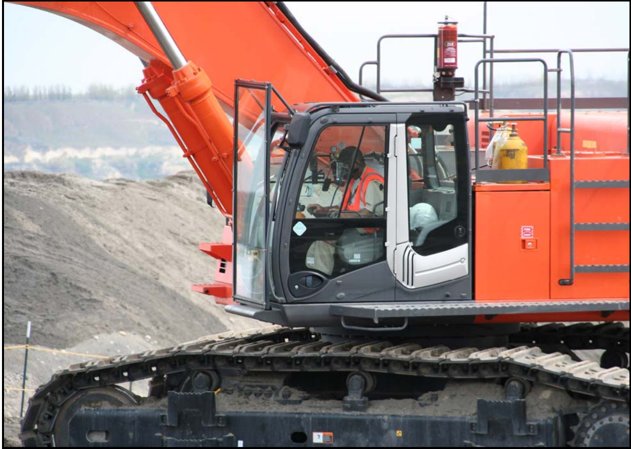
Washington Closure Hanford continues trench excavation at the 618-10 Burial Ground. The project team has started to encounter drums. (Photo 5)
