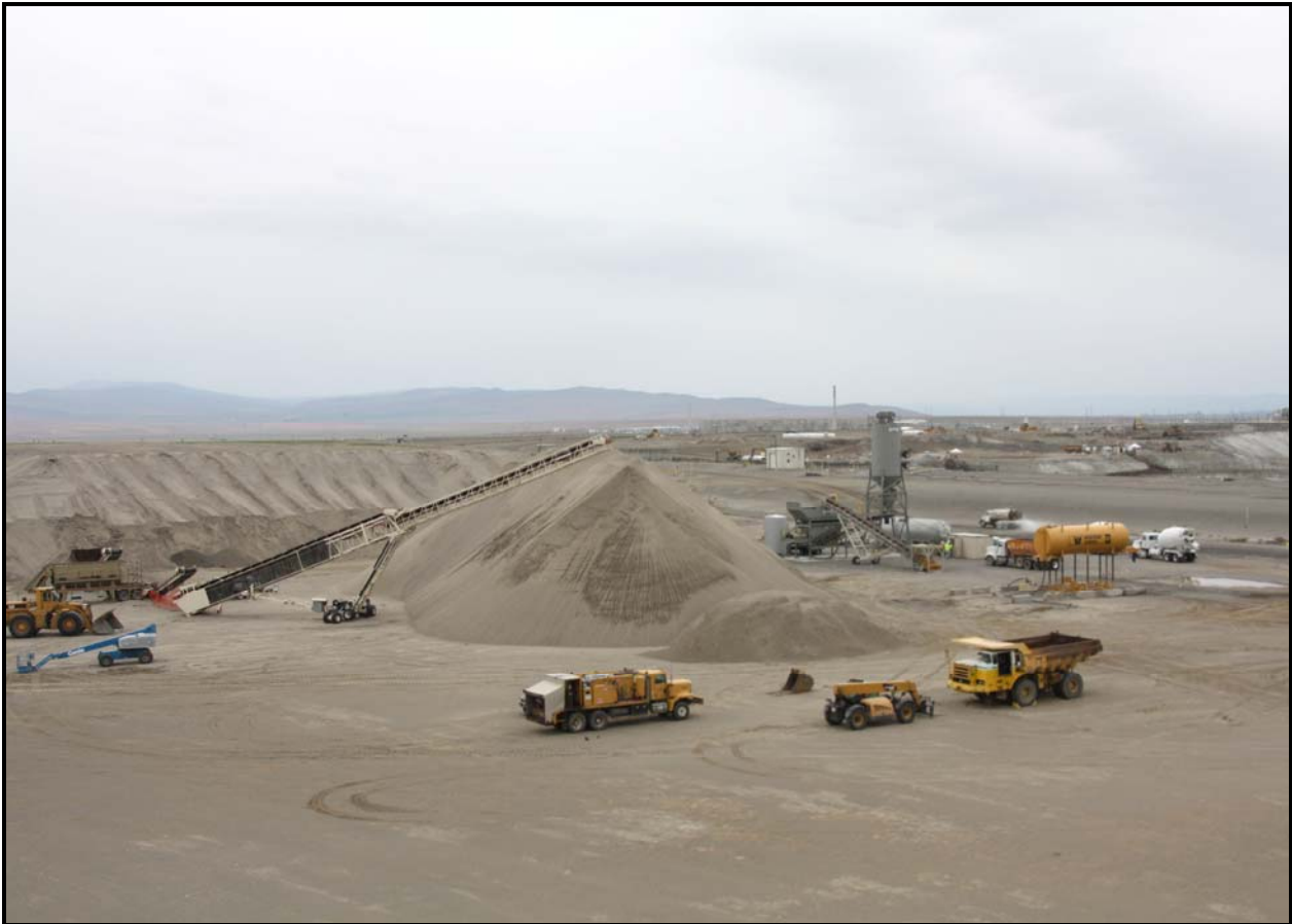
Washington Closure Hanford subcontractor TradeWind Services began operational testing of ERDF's new batch plant. The plant will be placed into service next month. (Photo 4)
