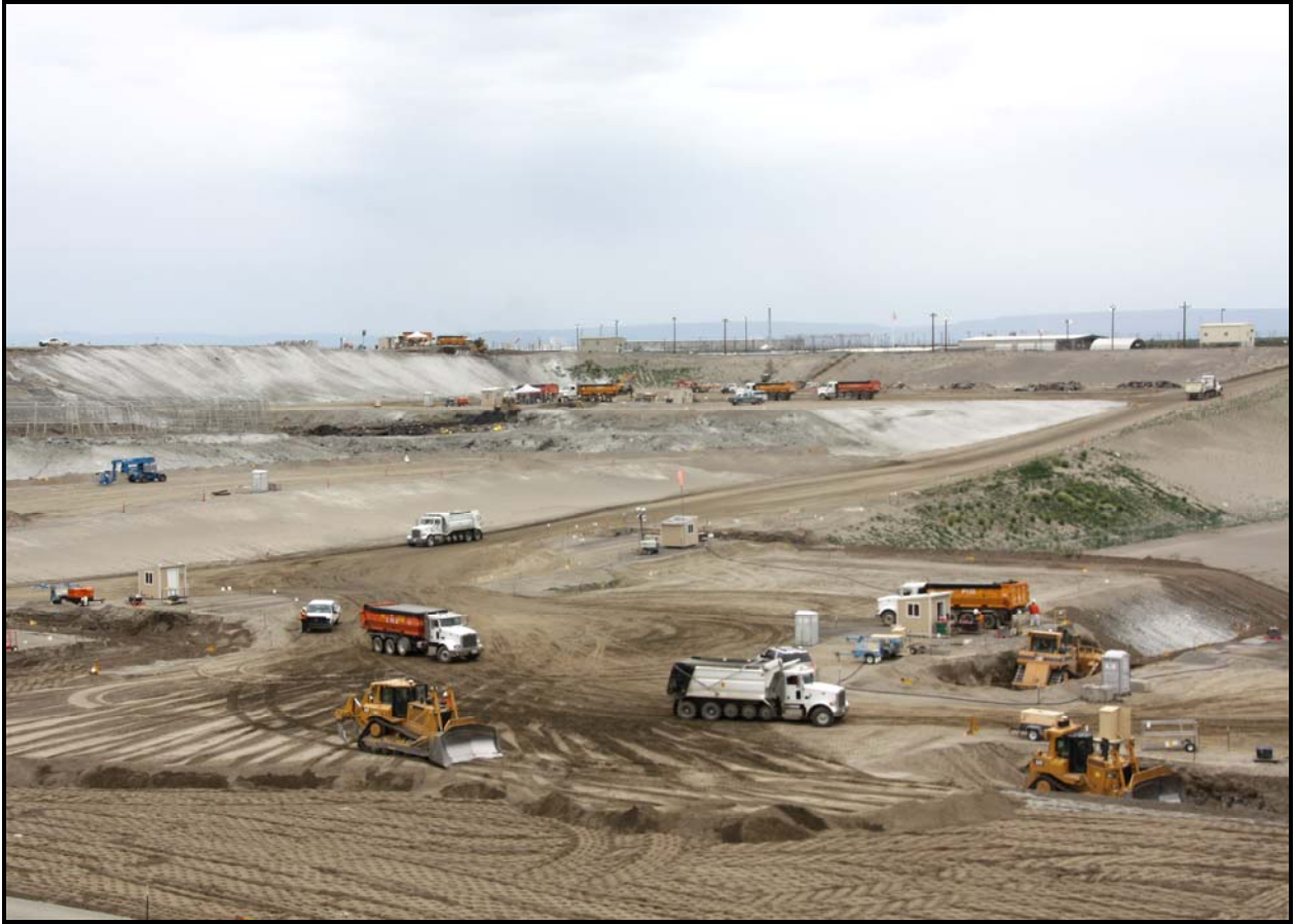
Two new dump ramps (bottom right) have been constructed in super cell 9 at the Environmental Restoration Disposal Facility. (Photo 3)
