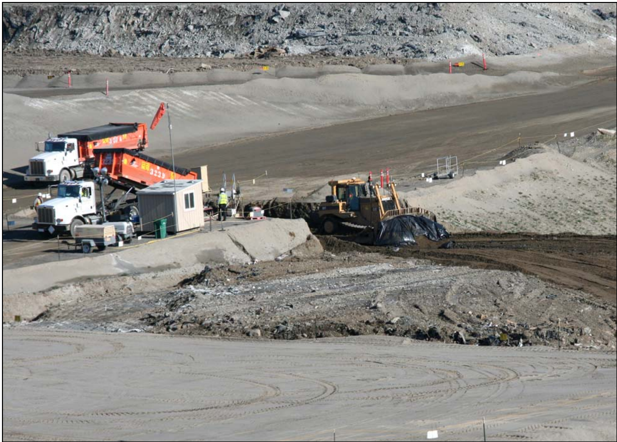
Waste is disposed in super cell 9 at the Environmental Restoration Disposal Facility. (Photo 1)
