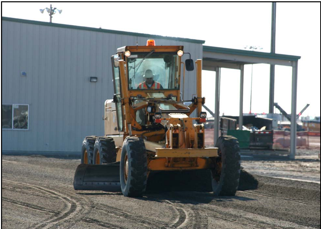
Washington Closure Hanford subcontractor ELRFowler grades the area between the container maintenance facility and the equipment maintenance facility/operations center. (Photo 2)
