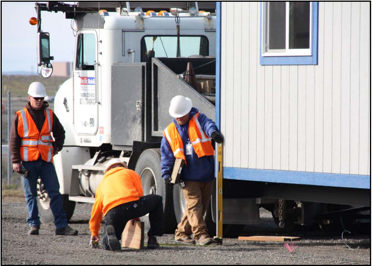
Employees from Pacific Mobile Structures set the first of two trailers at the 618-11 Burial Ground. In situ radiological characterization is expected to start later this month. (Photo 8)
