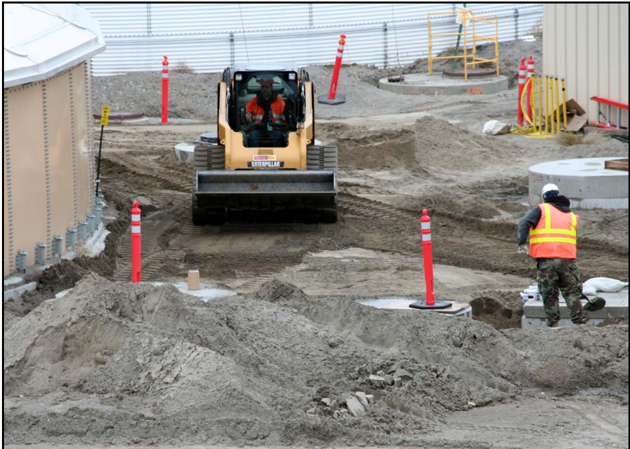
Washington Closure Hanford subcontractor DelHur Industries backfills around manholes associated with ERDF's two new leachate storage tanks. (Photo 1)
