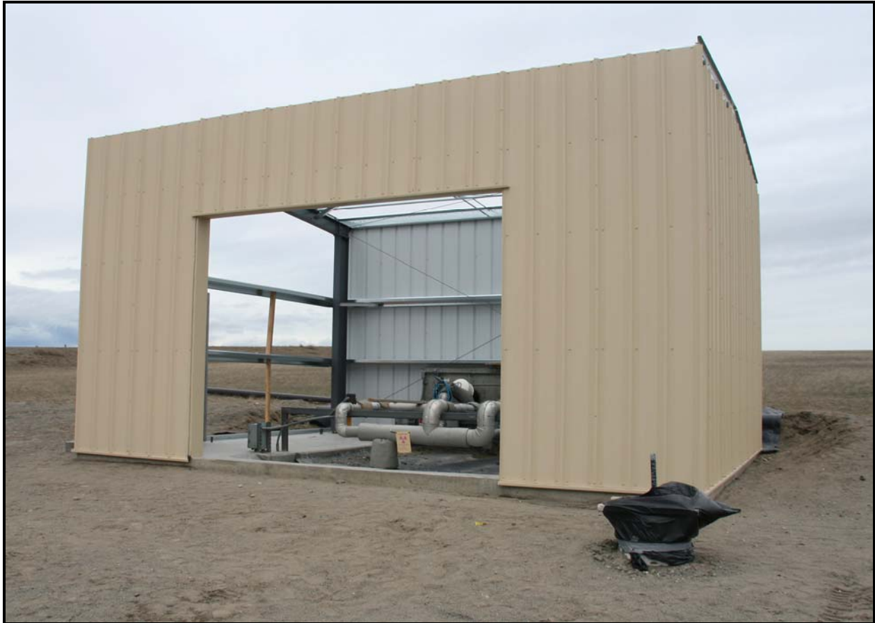
Washington Closure Hanford subcontractor TradeWind Services constructs the weather enclosure for the crest pad associated with cell 2. (Photo 4)
