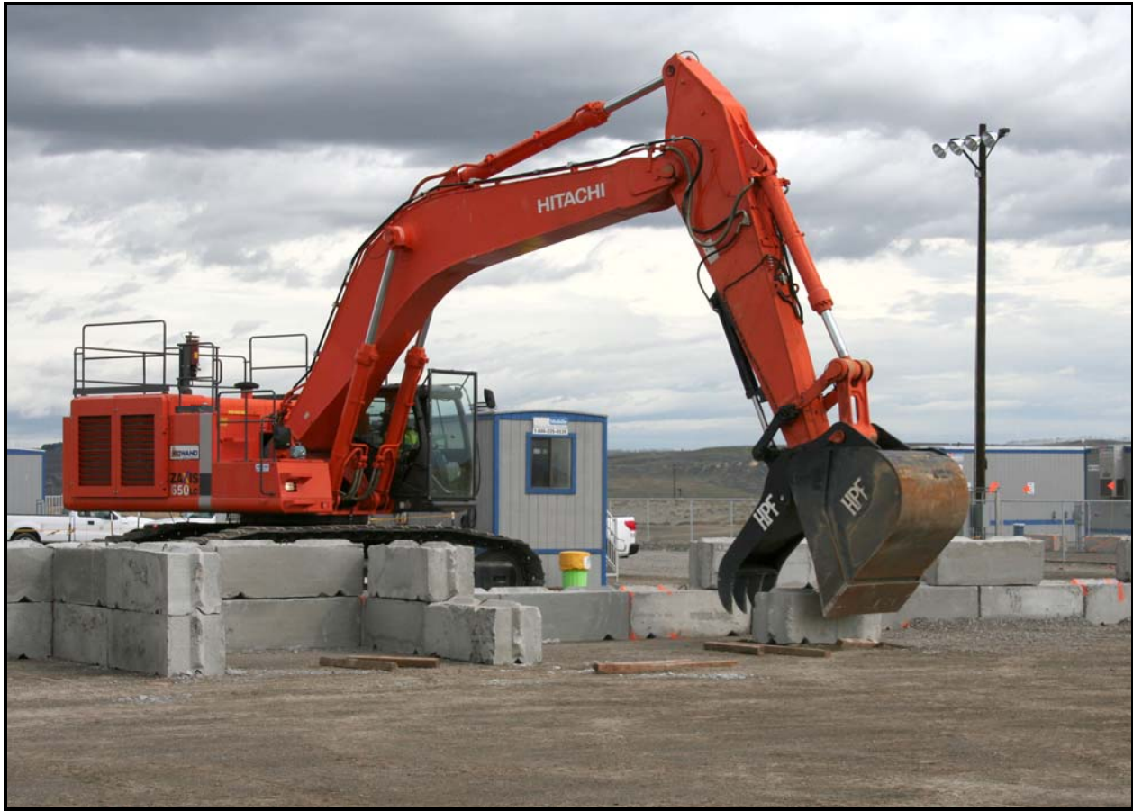
An excavator moves ecology blocks in the drum staging area during mockup exercises at the 618-10 Burial Ground. (Photo 6)
