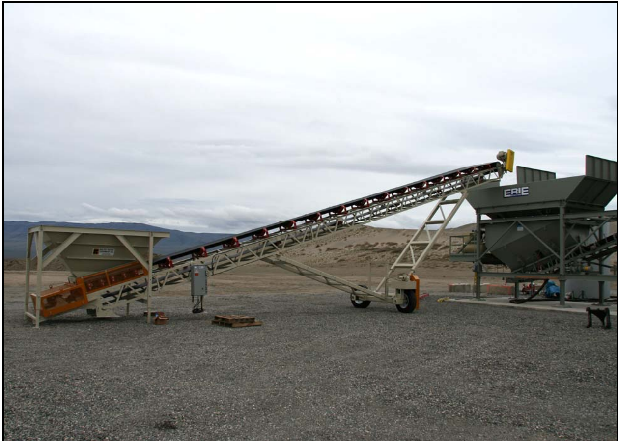
The conveyer and hopper for ERDF's new batch plant are being installed. (Photo 3)
