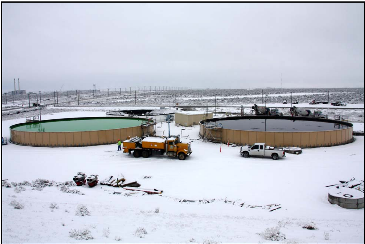
Washington Closure Hanford subcontractor TradeWind Services continues to construct two new leachate storage tanks at the Environmental Restoration Disposal Facility. (Photo 1)
