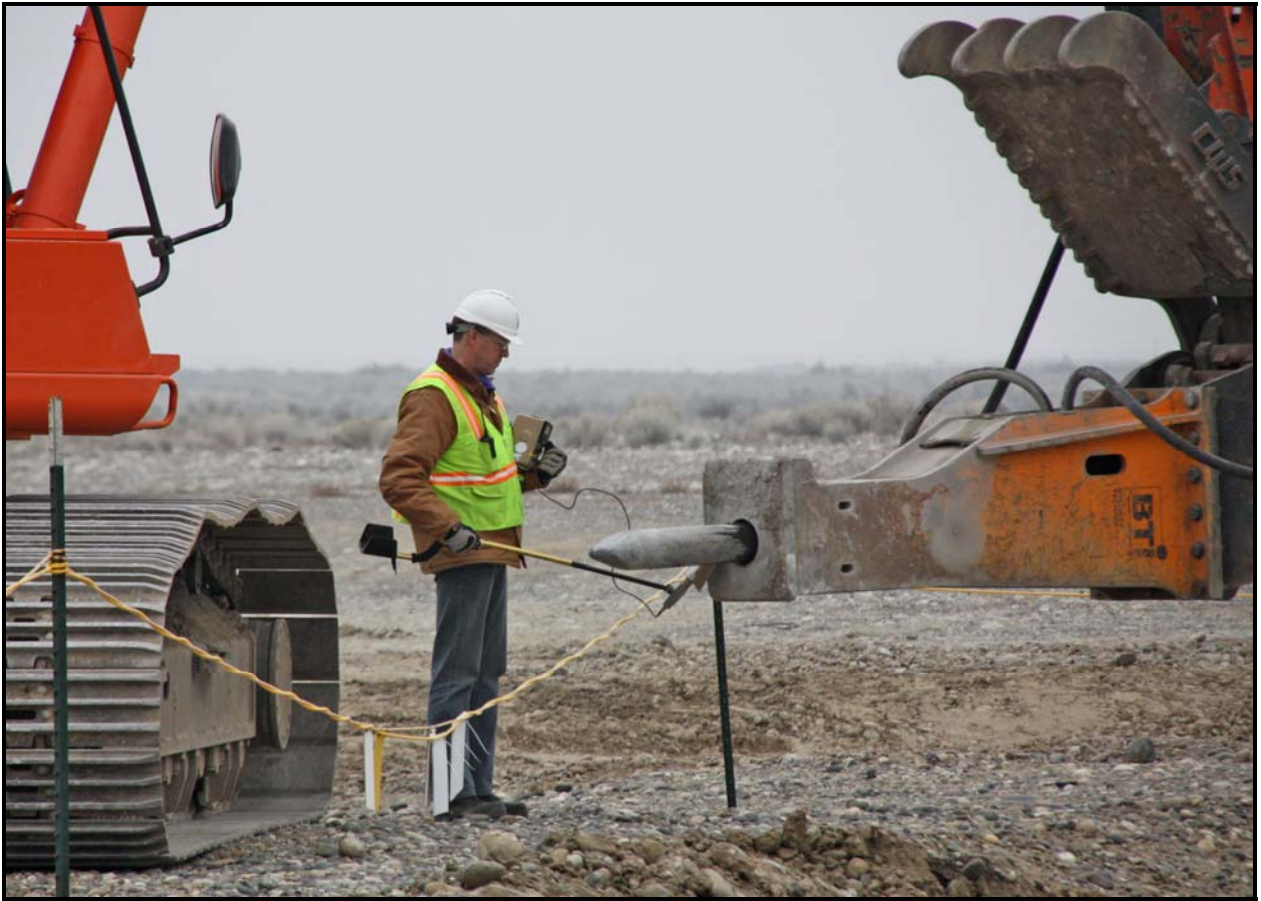
A radiological control technician takes a reading from the hammer used to demolish concrete at 100-F-44:9. Excavation and loadout activities at the site were completed. (Photo 6)
