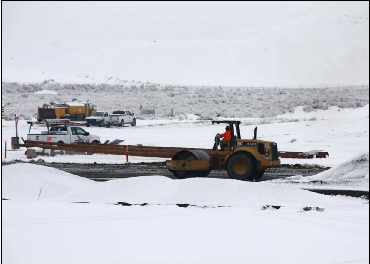
Civil work was completed on the expansion of the container transfer area at the Environmental Restoration Disposal Facility. (Photo 3)
