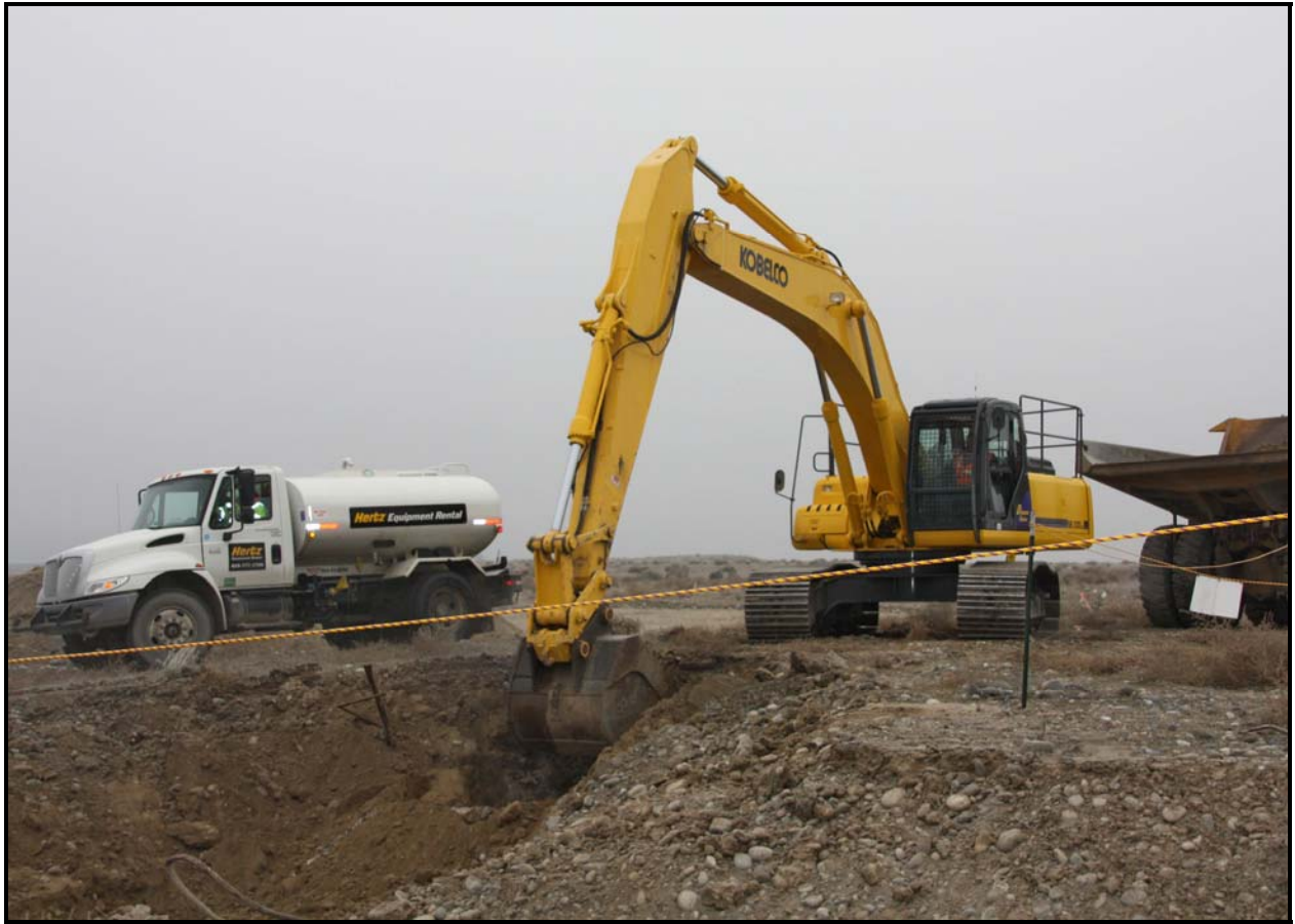
Ojeda Business Ventures conducts excavation activities at 100-F-63, which contains radioactive effluent lines from the 100-F Area experimental animal farm. (Photo 7)
