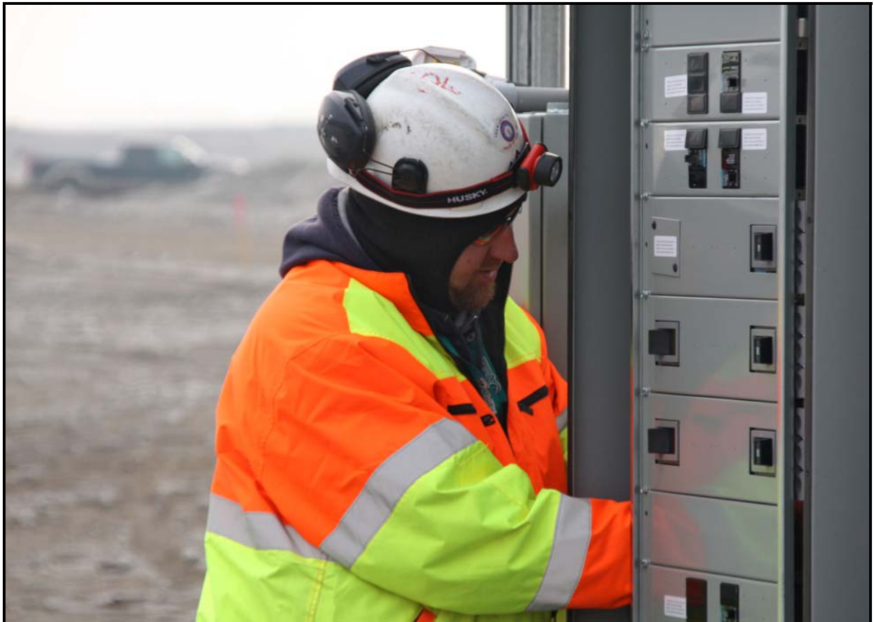
A Washington Closure Hanford subcontractor works to install electrical at the 618-10 Burial Ground. Remediation activities at the burial ground are scheduled to begin in March. (Photo 4)
