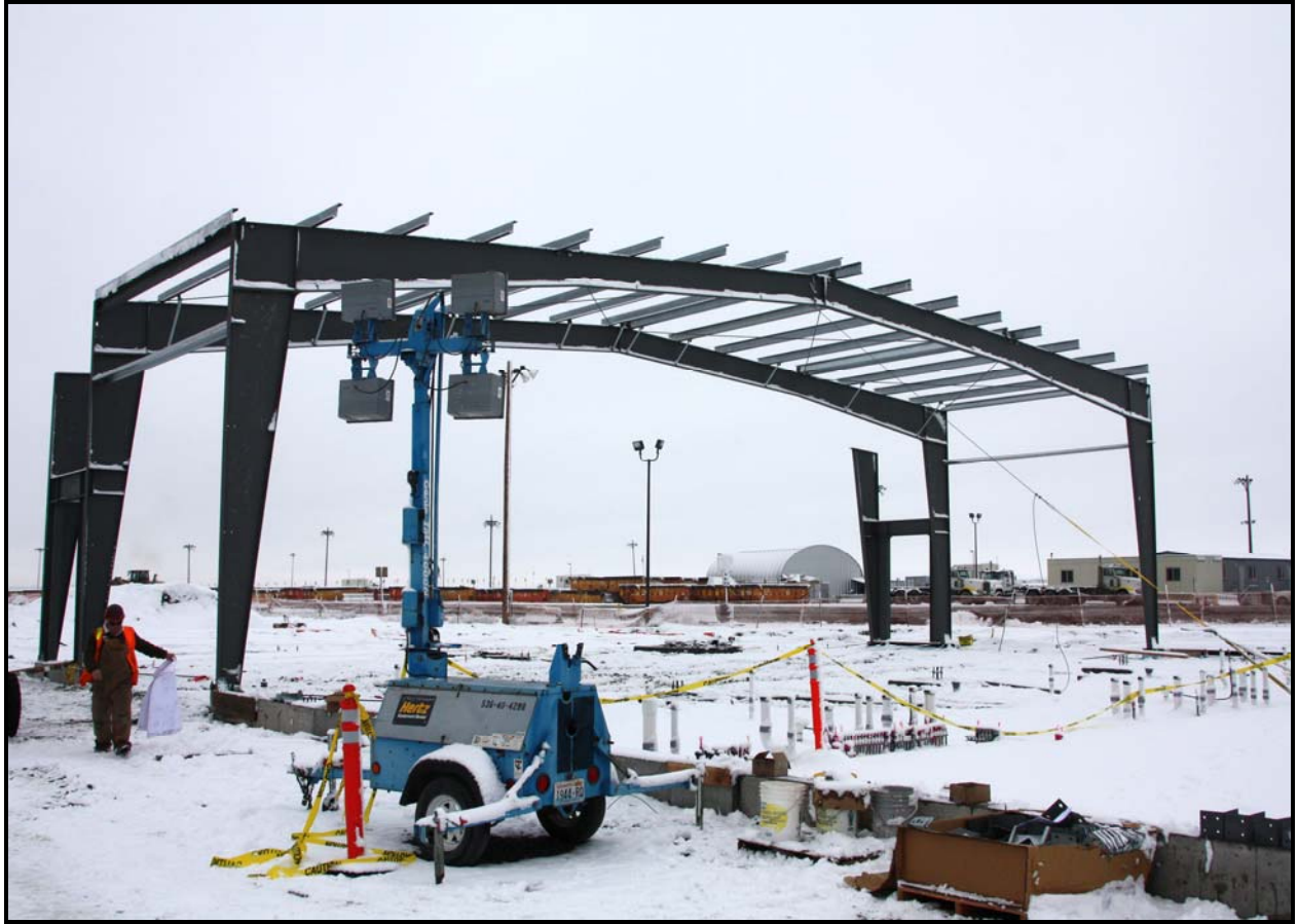
Washington Closure Hanford subcontractor Fowler General Construction begins to erect the steel structure of ERDF's equipment maintenance facility/operations center. (Photo 2)
