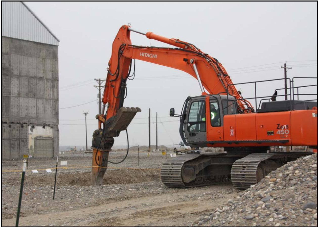
Washington Closure Hanford subcontractor Ojeda Business Ventures demolishes concrete at 100-F-44:9. The site, adjacent to F Reactor, contains process sewer line. (Photo 5)
