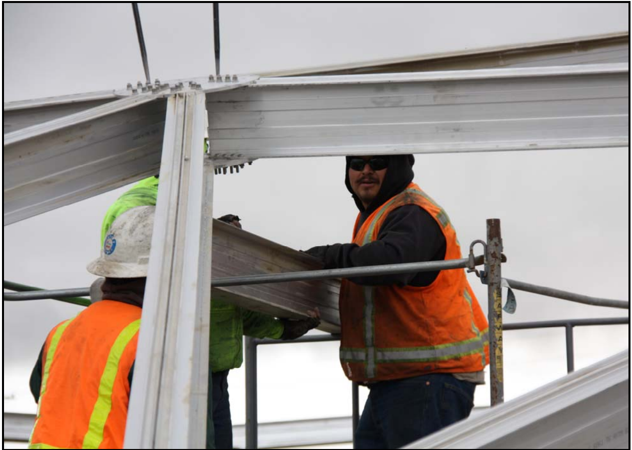
A Washington Closure Hanford subcontractor assembles the frame of the dome cover for Leachate Storage Tank No. 4 at the Environmental Restoration Disposal Facility. (Photo 3)
