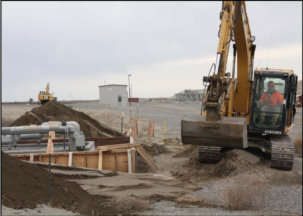
Washington Closure Hanford subcontractor DelHur Industries began construction of the weather enclosure for the crest pad associated with cell 1. (Photo 6)
