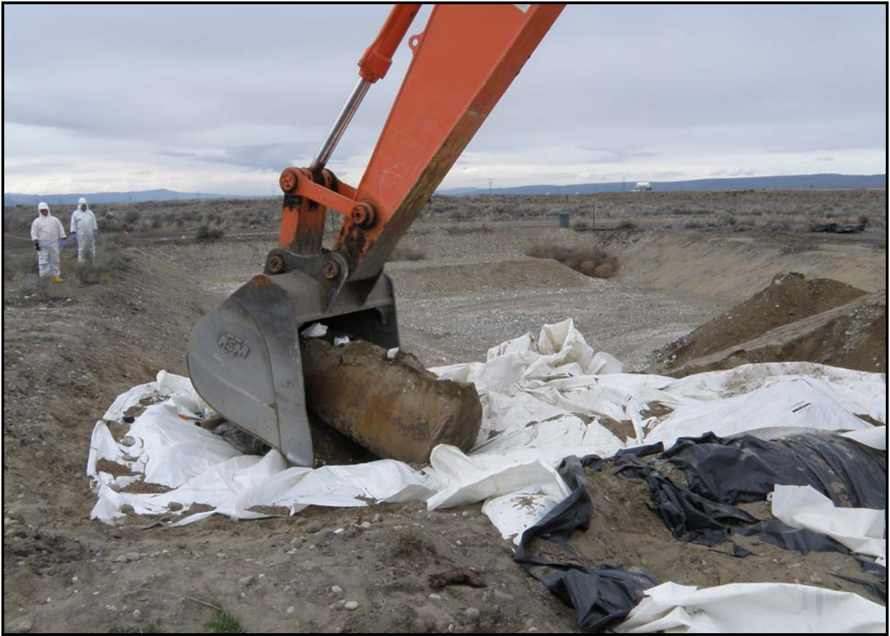
A drum containing waste oil is removed from 100-F-49. The oil was drained from the drum before removal. (Photo 13)
