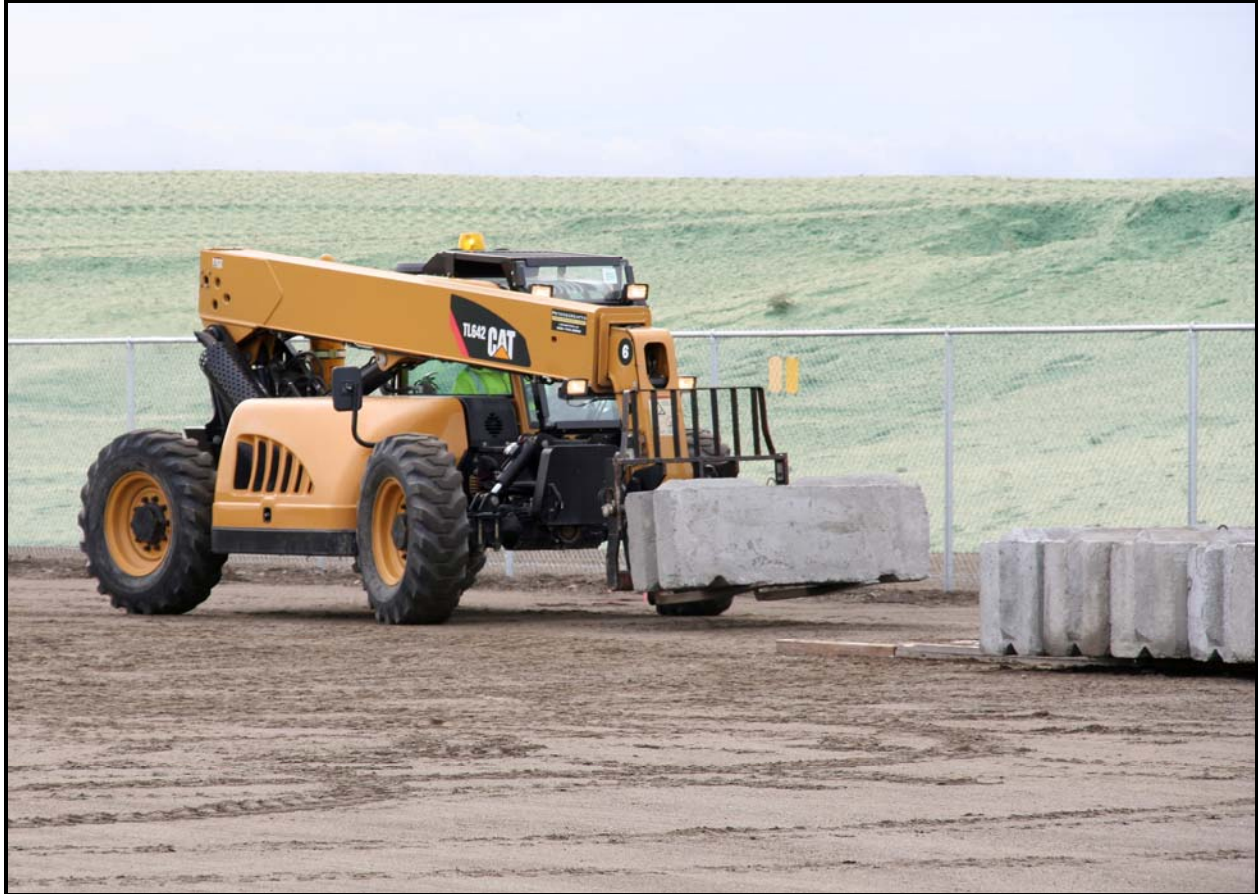
Washington Closure Hanford subcontractor White Shield/Apollo moves ecology blocks in the drum-punch area at the 618-10 Burial Ground. (Photo 7)
