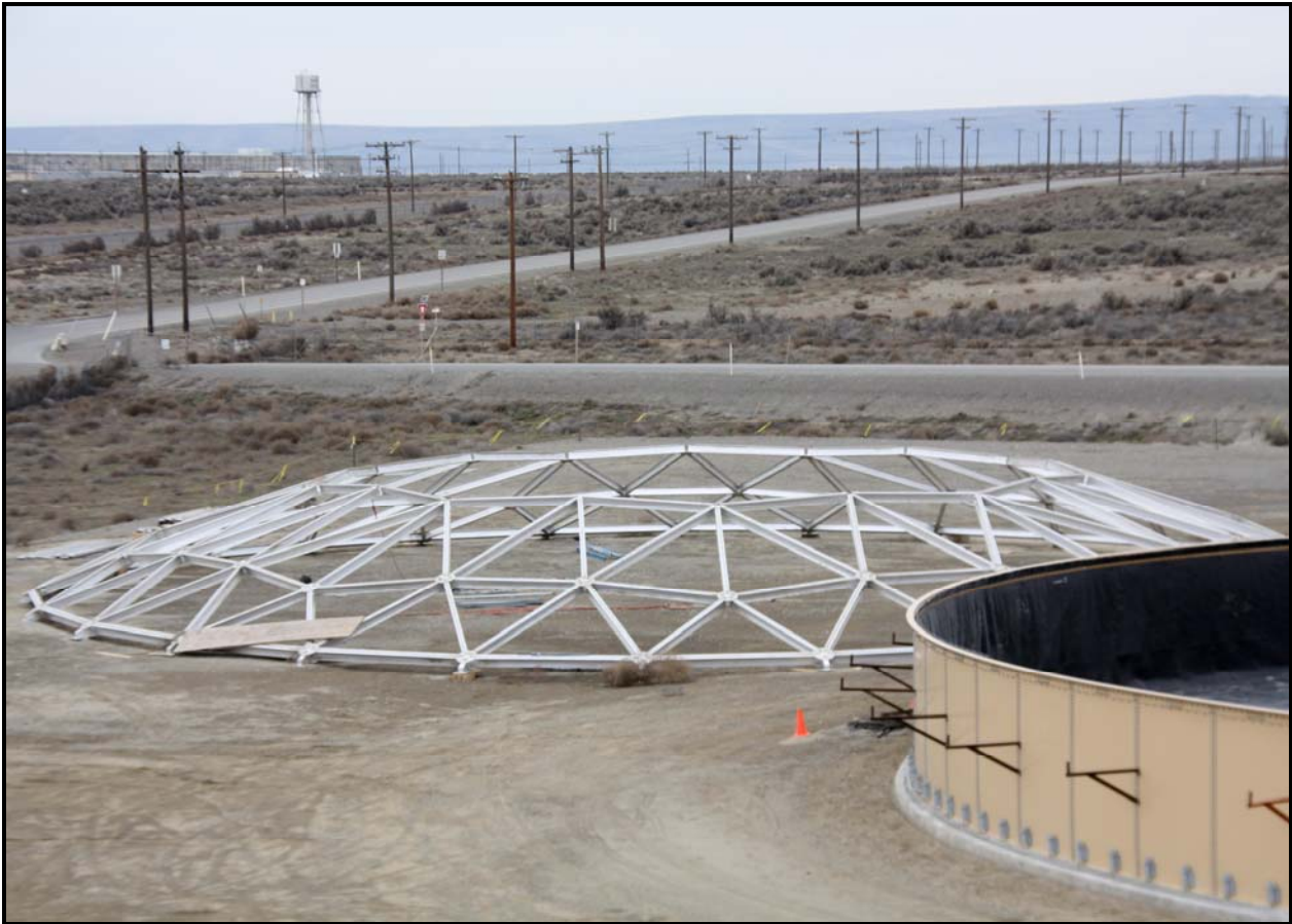
Work to place the skins over the dome frames will begin next week. The dome covers are scheduled to be set on the tanks in March. (Photo 4)
