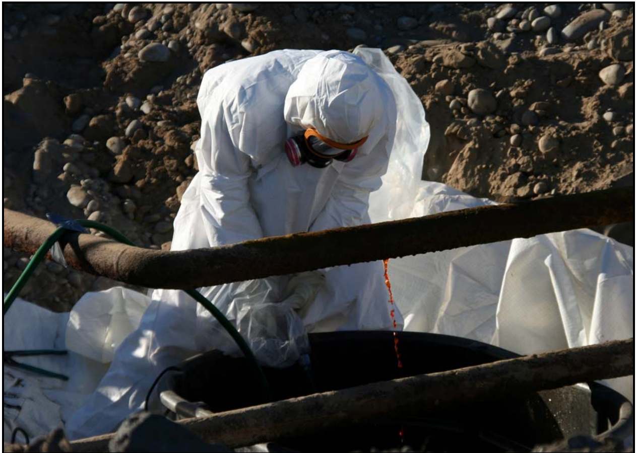
A Washington Closure Hanford subcontractor safely drains sodium dichromate from a pipe at 100-F-26:7. (Photo 10)
