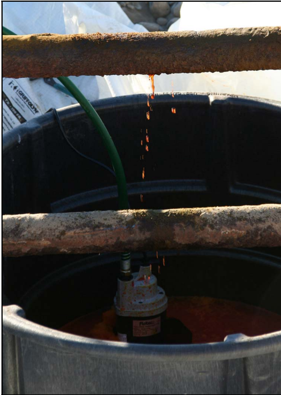
The safe and effective draining of sodium dichromate from the pipes at 100-F-26:7 prevented potential leaking and groundwater contamination. (Photo 11)
