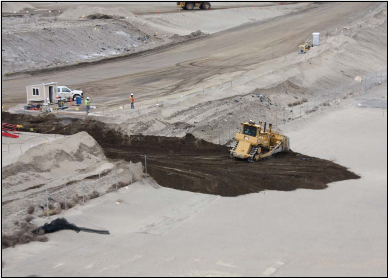
A bulldozer spreads waste in super cell 9 at the Environmental Restoration Disposal Facility. (Photo 2)
