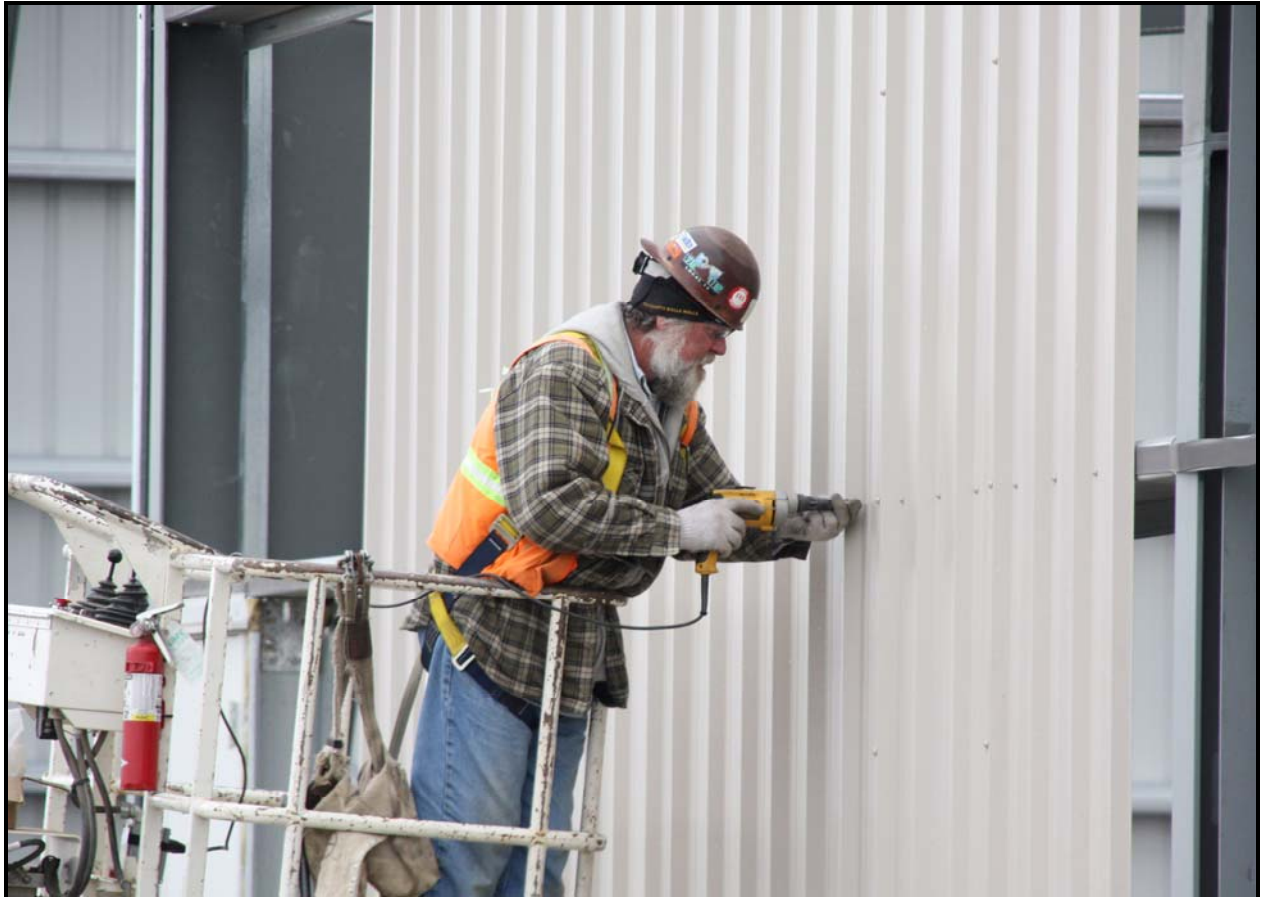
An employee from Washington Closure Hanford subcontractor ELRFowler installs siding at the equipment maintenance facility/operations center. (Photo 5)
