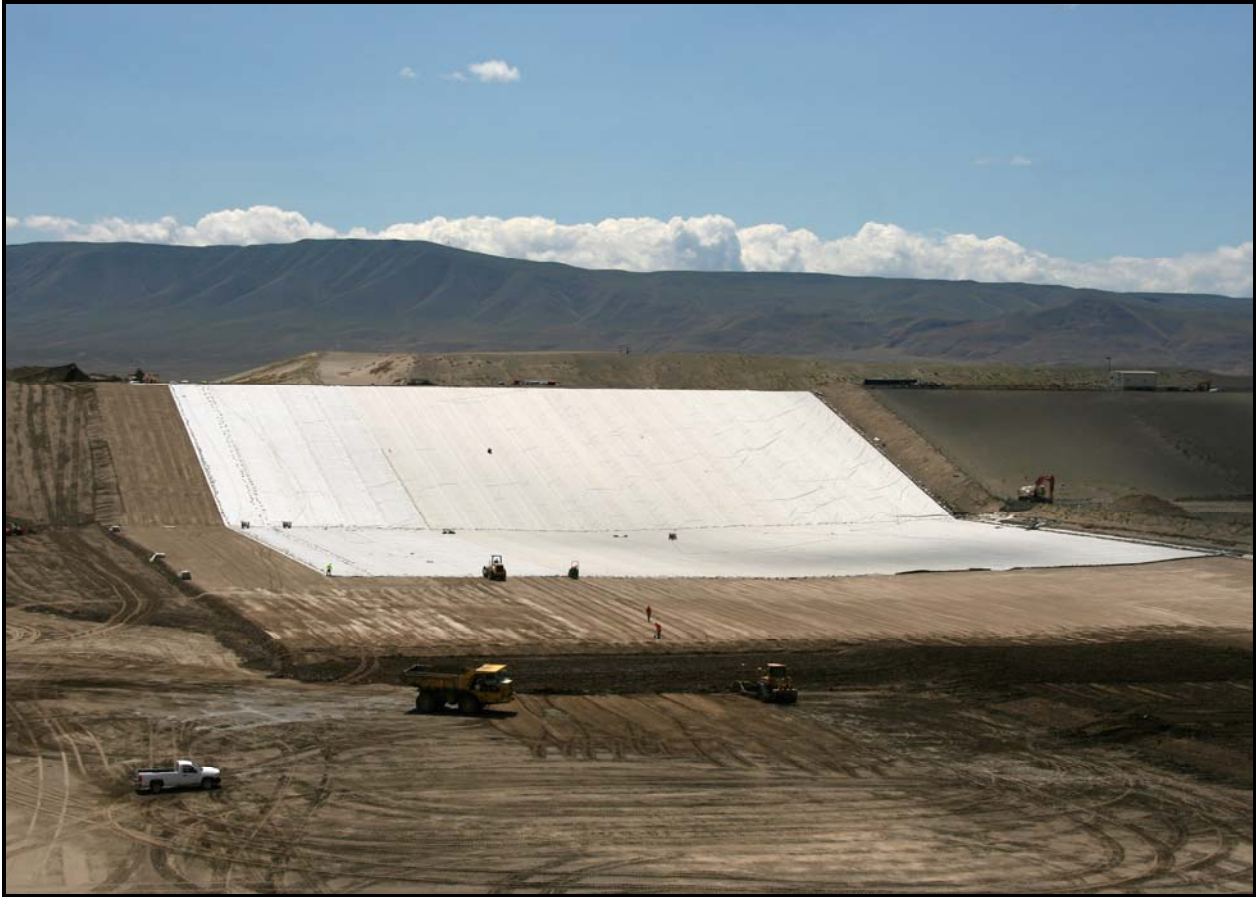
A view from the north side of super cell 9 at the Environmental Restoration Disposal Facility shows the installation of high-density polyethylene and the placement of admix.
