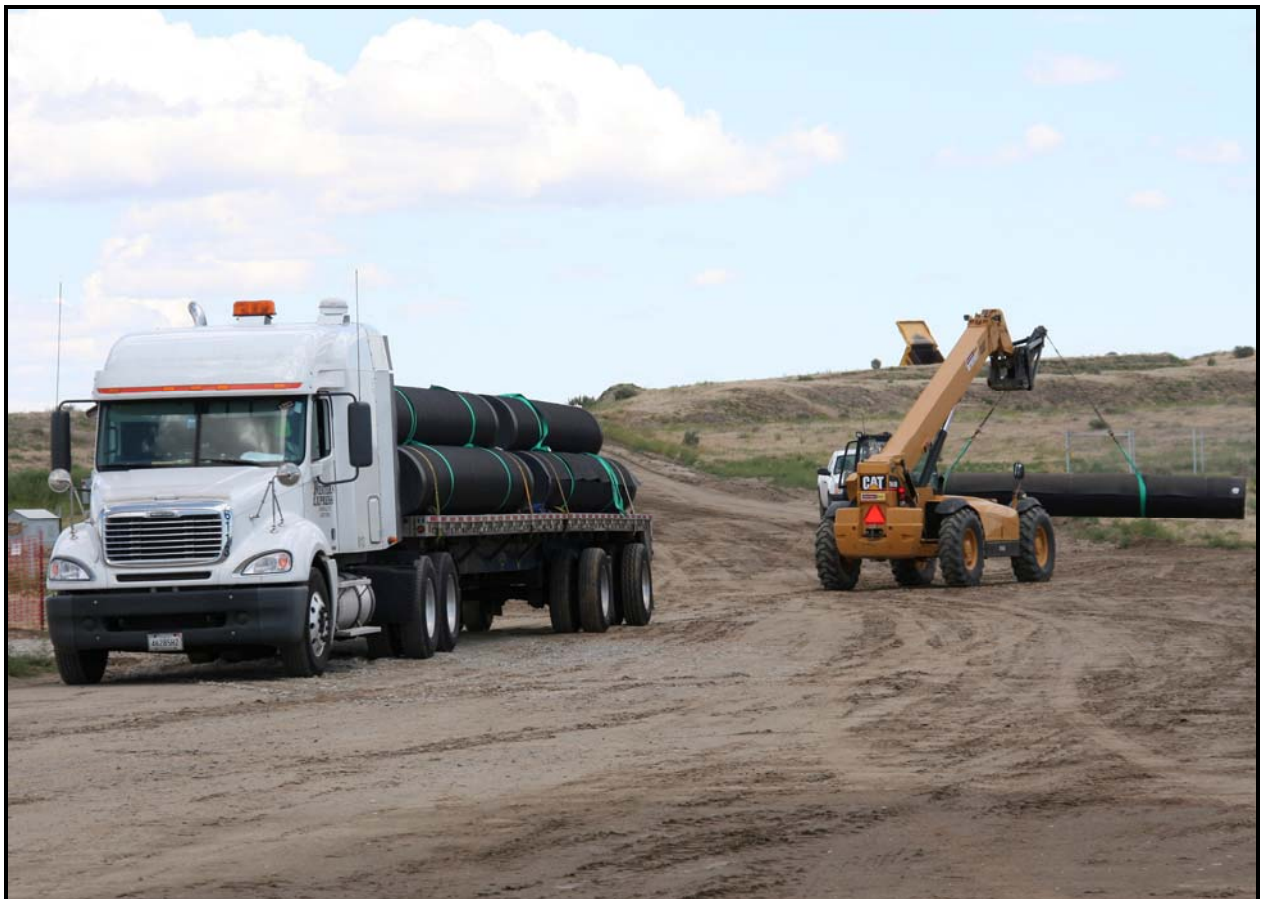
Rolls of high-density polyethylene (HDPE) arrive at the Environmental Restoration Disposal Facility. The HDPE is used in the liner system being installed in super cell 9. The material is installed in 540- by 22-foot sections and heat-welded together.
