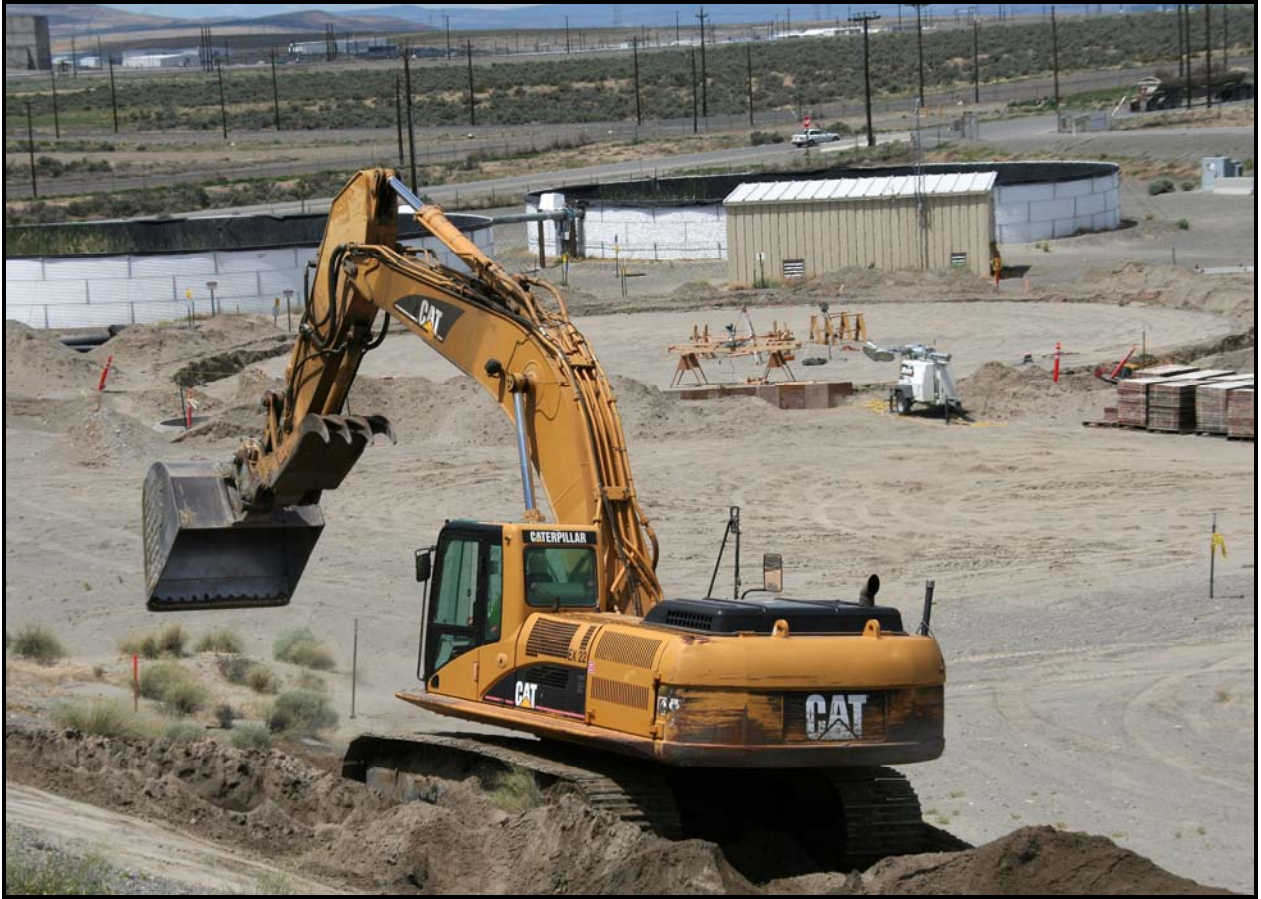
Construction of a new leachate holding tank begins at the Environmental Restoration Disposal Facility. The holding tank will accommodate leachate from super cells 9 and 10.
