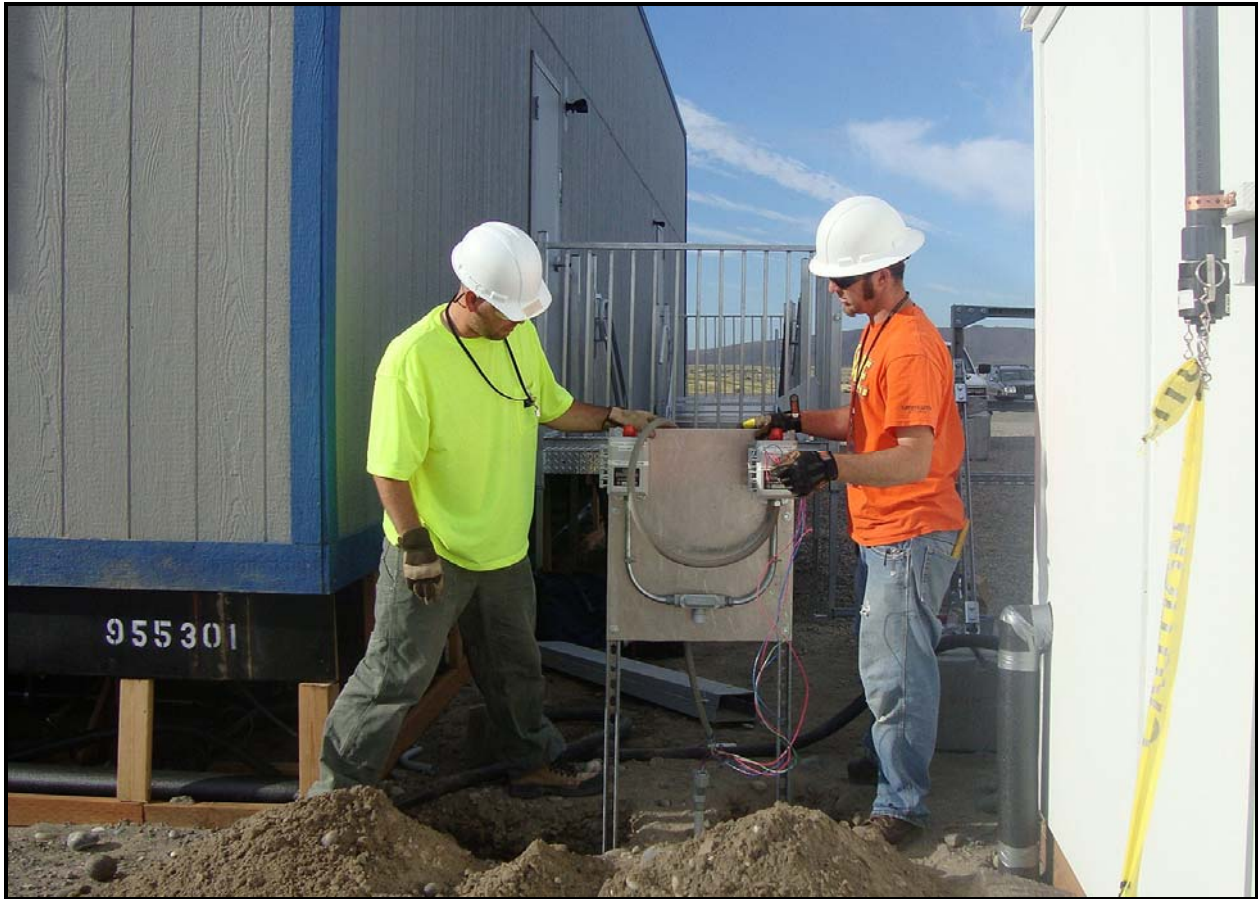
Washington Closure subcontractor Northpoint Electrical completed electrical installations to the mobile trailers at 100-F Area.
