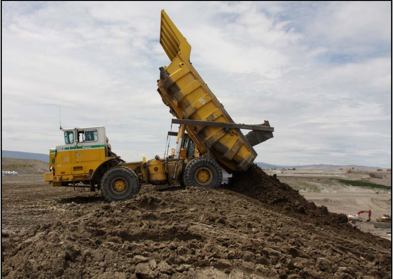
TradeWind Services/DelHur Industries personnel dump admix on the south slope of super cell 9 at the Environmental Restoration Disposal Facility.
