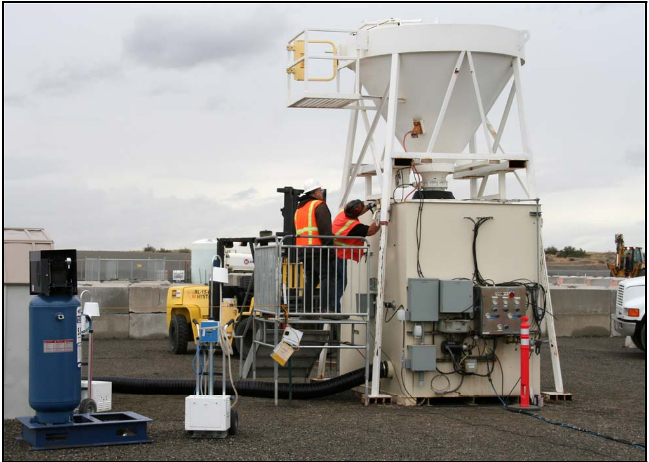
Workers install a sand hopper at the 618-10 Burial Ground. In the event an unearthed drum generates heat, sand will be dropped from the hopper onto the drum inside the enclosure.
