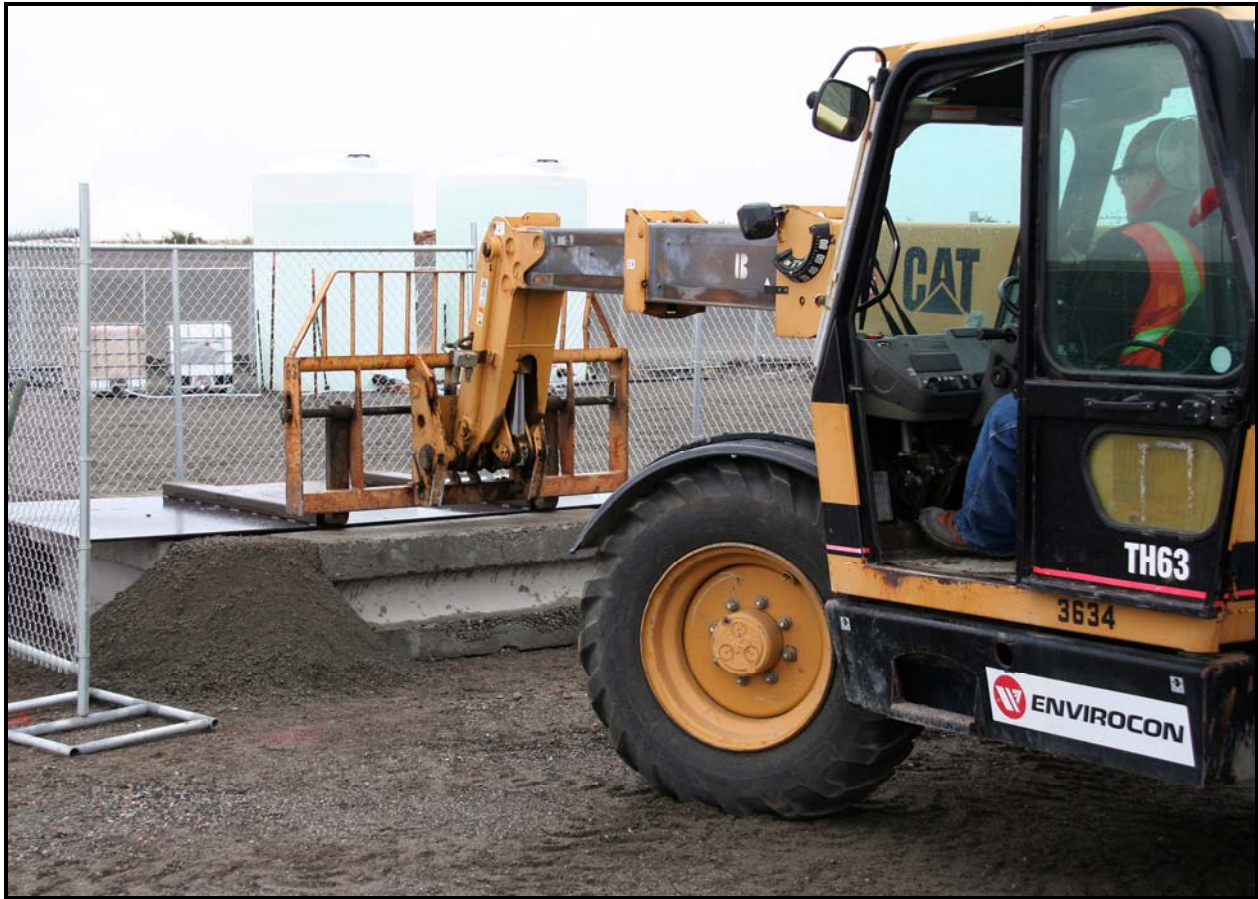
Work begins on a bunker that will be used to contain suspect spent nuclear fuel at the 618-10 Burial Ground.
