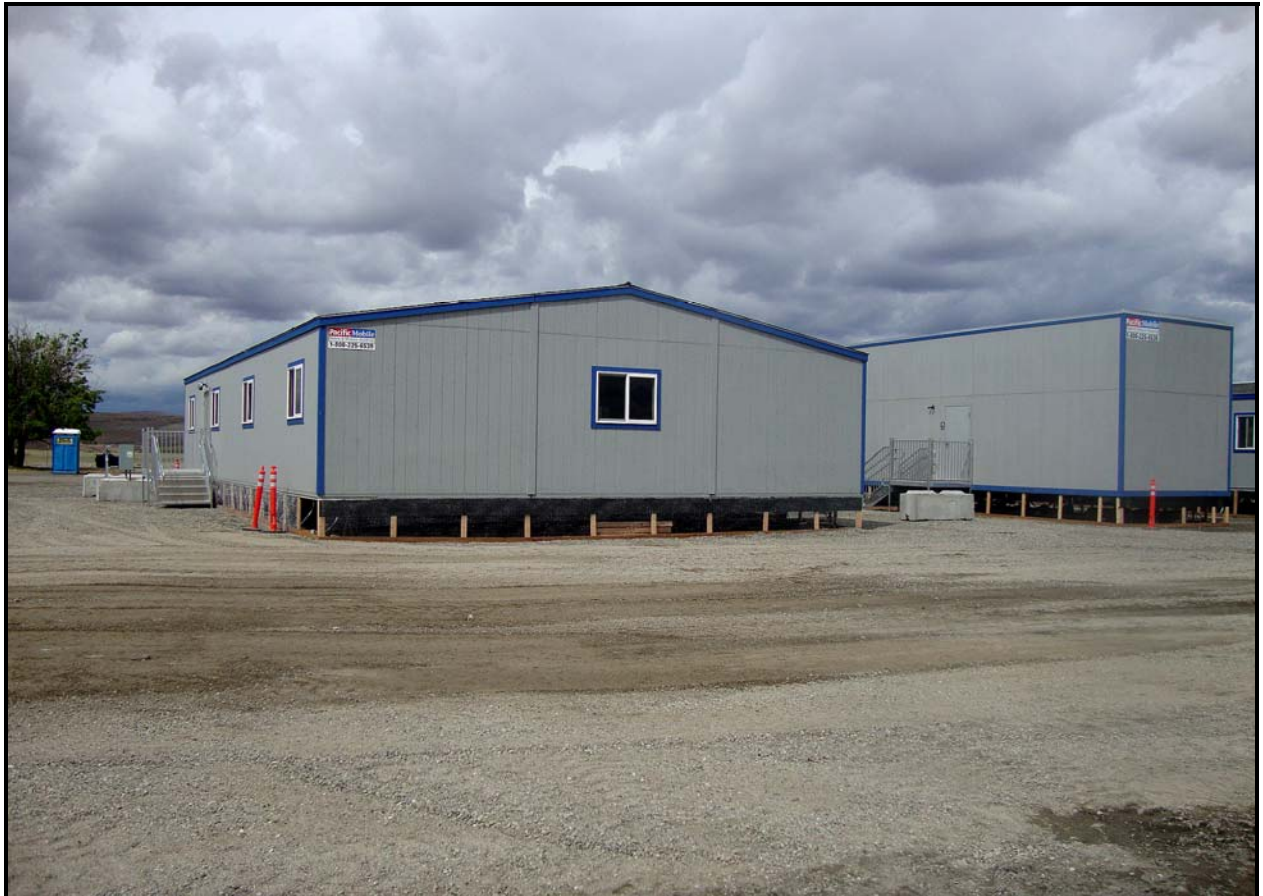
Preparations continue at 100-F Area. Trailers are being installed, and trenches for electrical communication have been backfilled.
