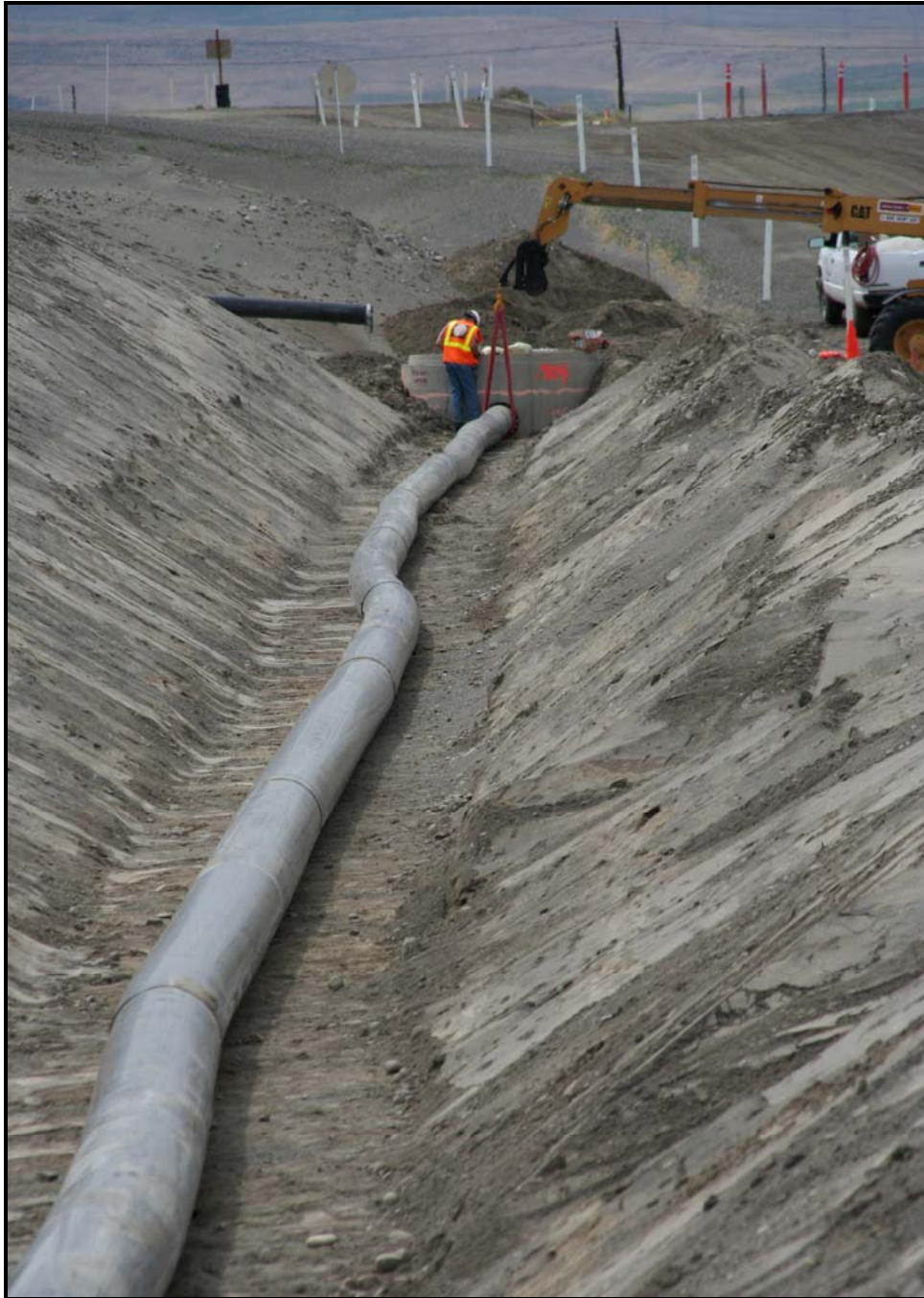
Work continues on the installation of the leachate transfer pipe from super cell 9 at the Environmental Restoration Disposal Facility
