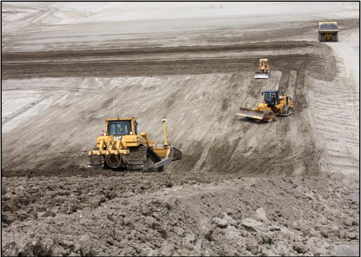
A bulldozer (left) spreads admix on the south slope of super cell 9 at the Environmental Restoration Disposal Facility. A sheepfoot compactor (right) prepares to climb the slope.
