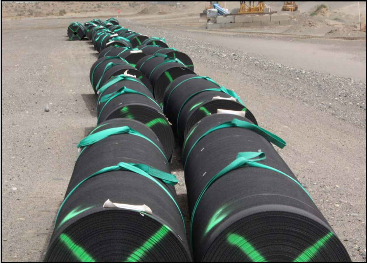
High-density polyethylene (HDPE) is used as part of the cell liners system at the Environmental Restoration Disposal Facility. Construction of the liner for super cell 9 will begin next week.
