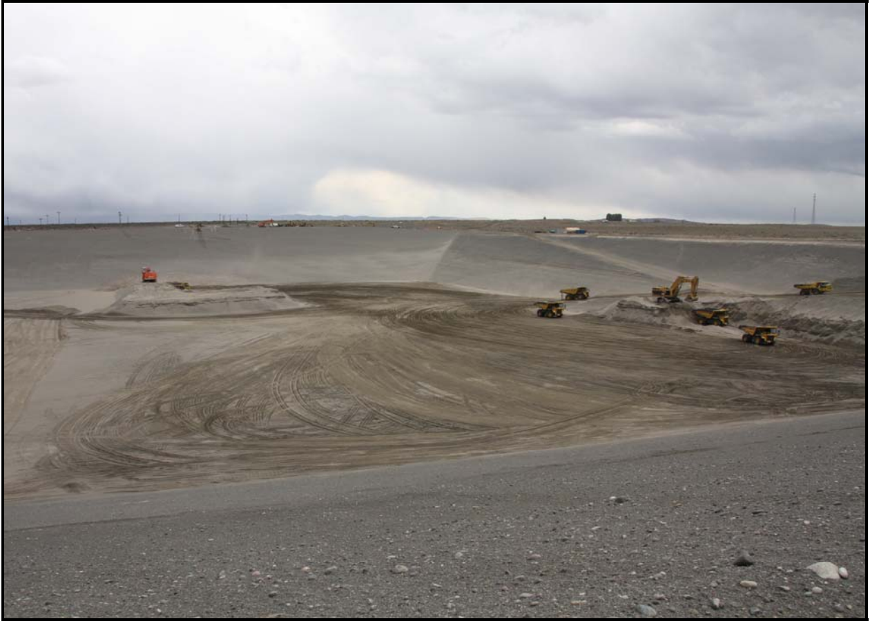
This photo was taken May 5, the day before mass excavation of super cell 10 was completed at the Environmental Restoration Disposal Facility.
