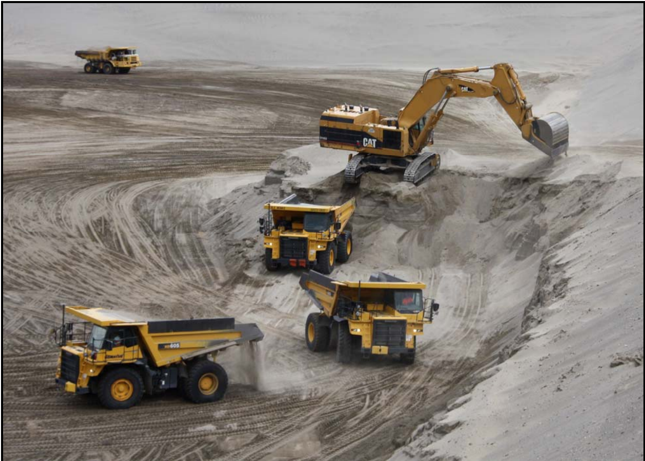
TradeWind Services/DelHur Industries personnel excavate the final portion of an estimated 1.675 cubic yards of soil from super cell 10 at the Environmental Restoration Disposal Facility.
