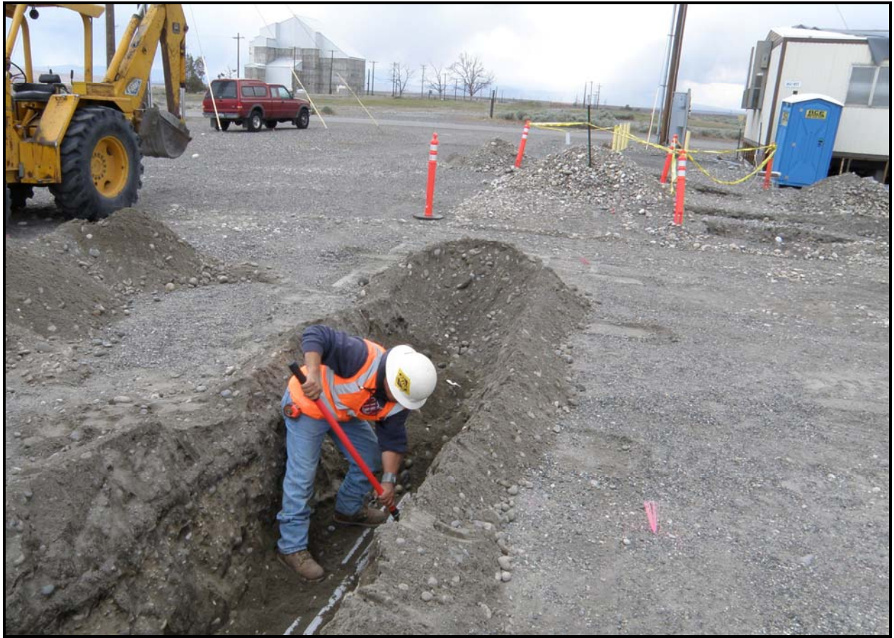
A Washington Closure subcontractor works on the installation of electrical conduit to support mobile offices at the 100-F Area. Work to remediate 12 additional waste sites at the 100-F Area is scheduled to begin this summer.
