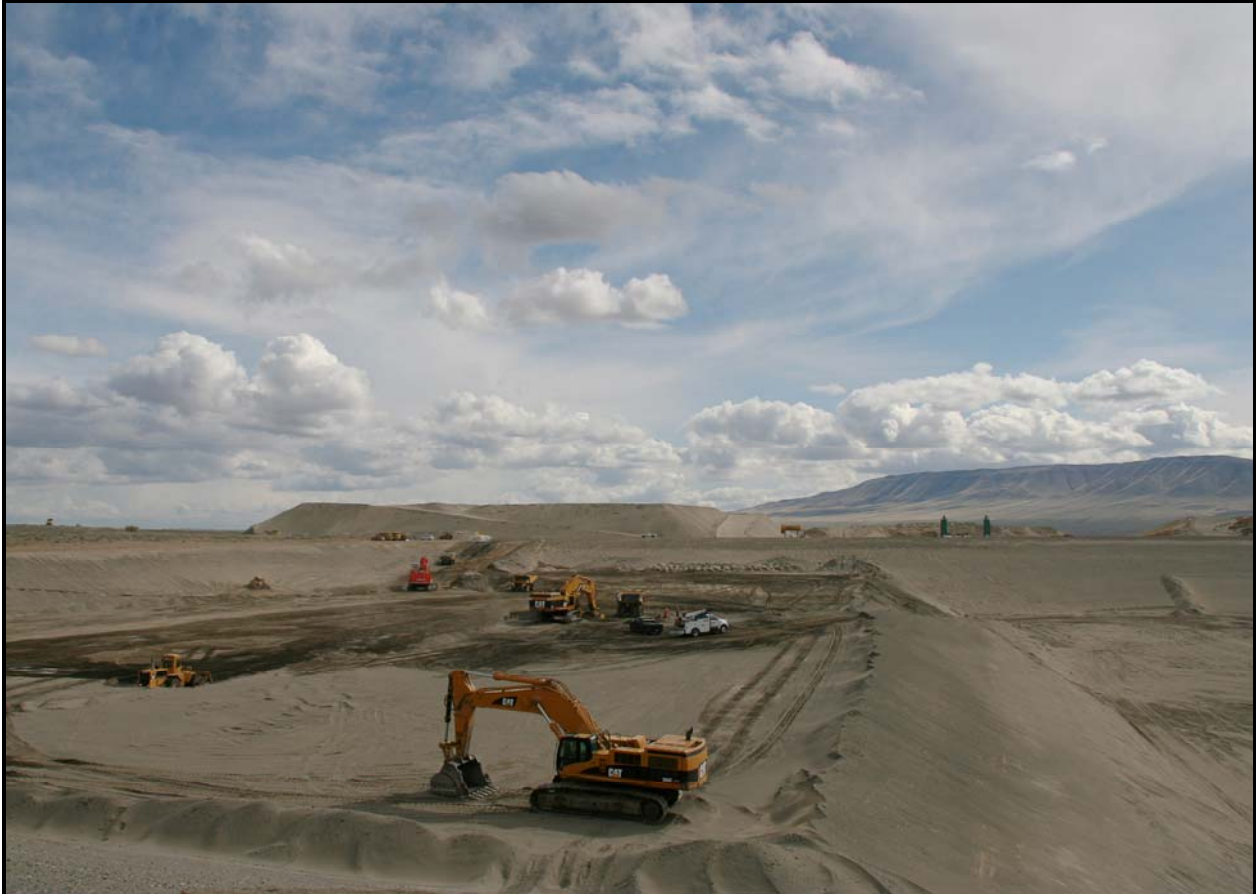
DelHur Industries continues work on super cell 10 at the Environmental Restoration Disposal Facility.
