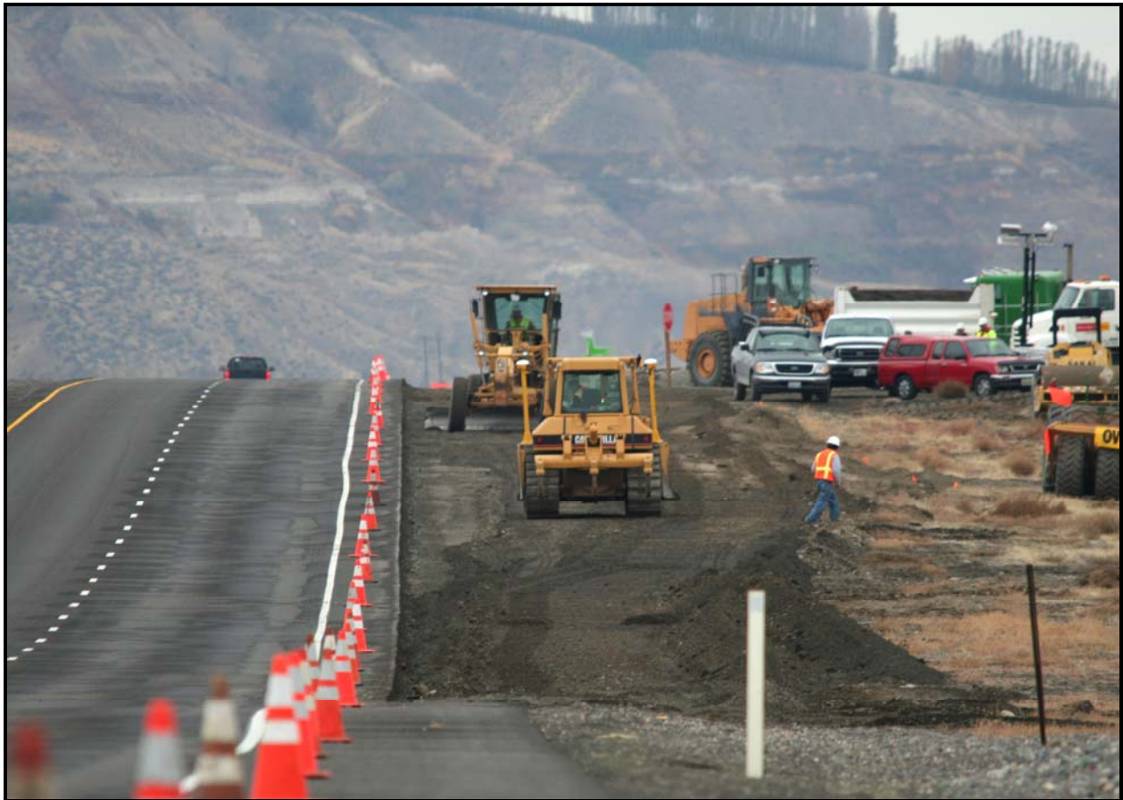
Road construction is underway near the 618-10 Burial Ground, about 4 miles north of the 300 Area. Road crews are working to remove and dispose of the asphalt shoulder and preparing to build entrance and exit lanes.
