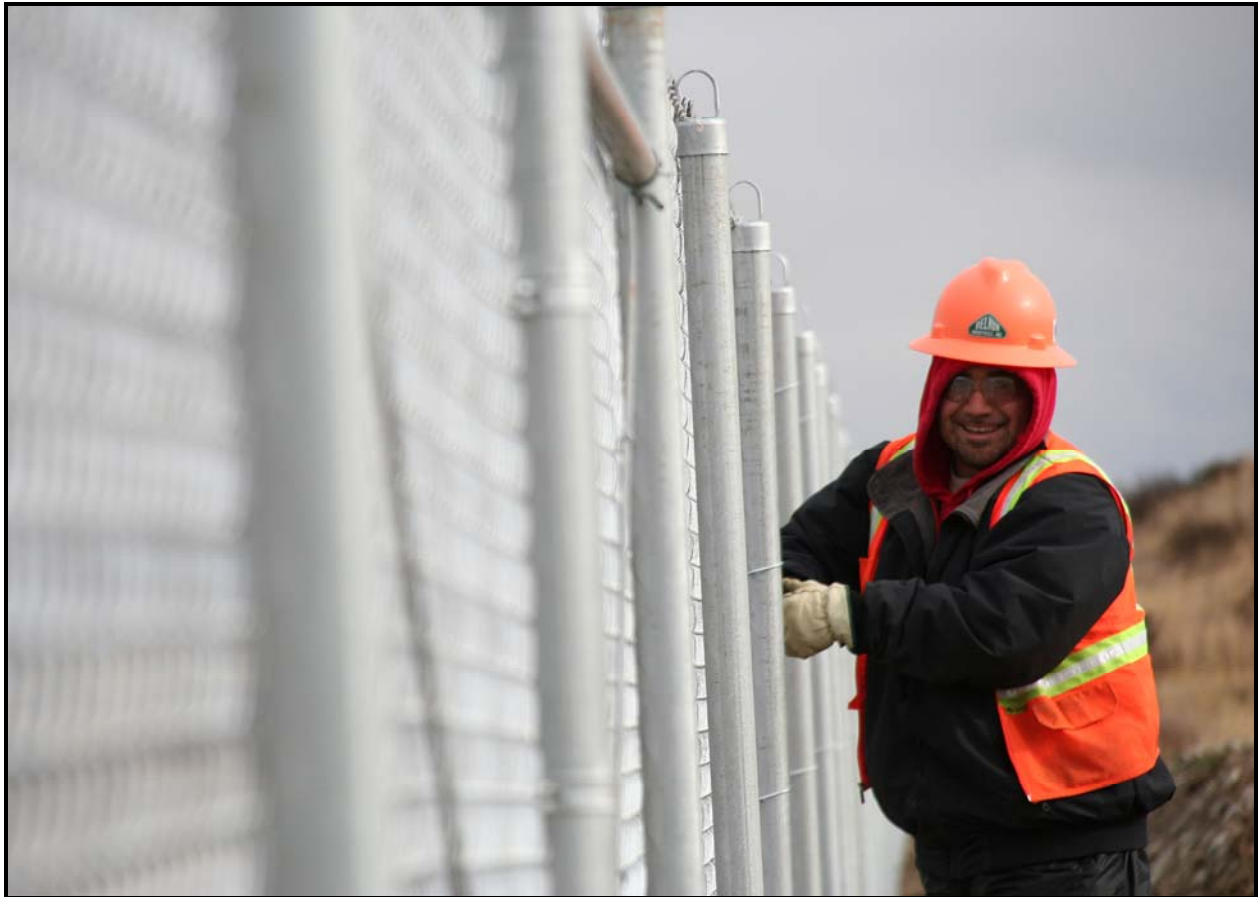
A DelHur Industries employee works on the boundary fence for super cells 9 and 10 at the Environmental Restoration Disposal Facility. The fence contractor is American Fencing of Hermiston.
