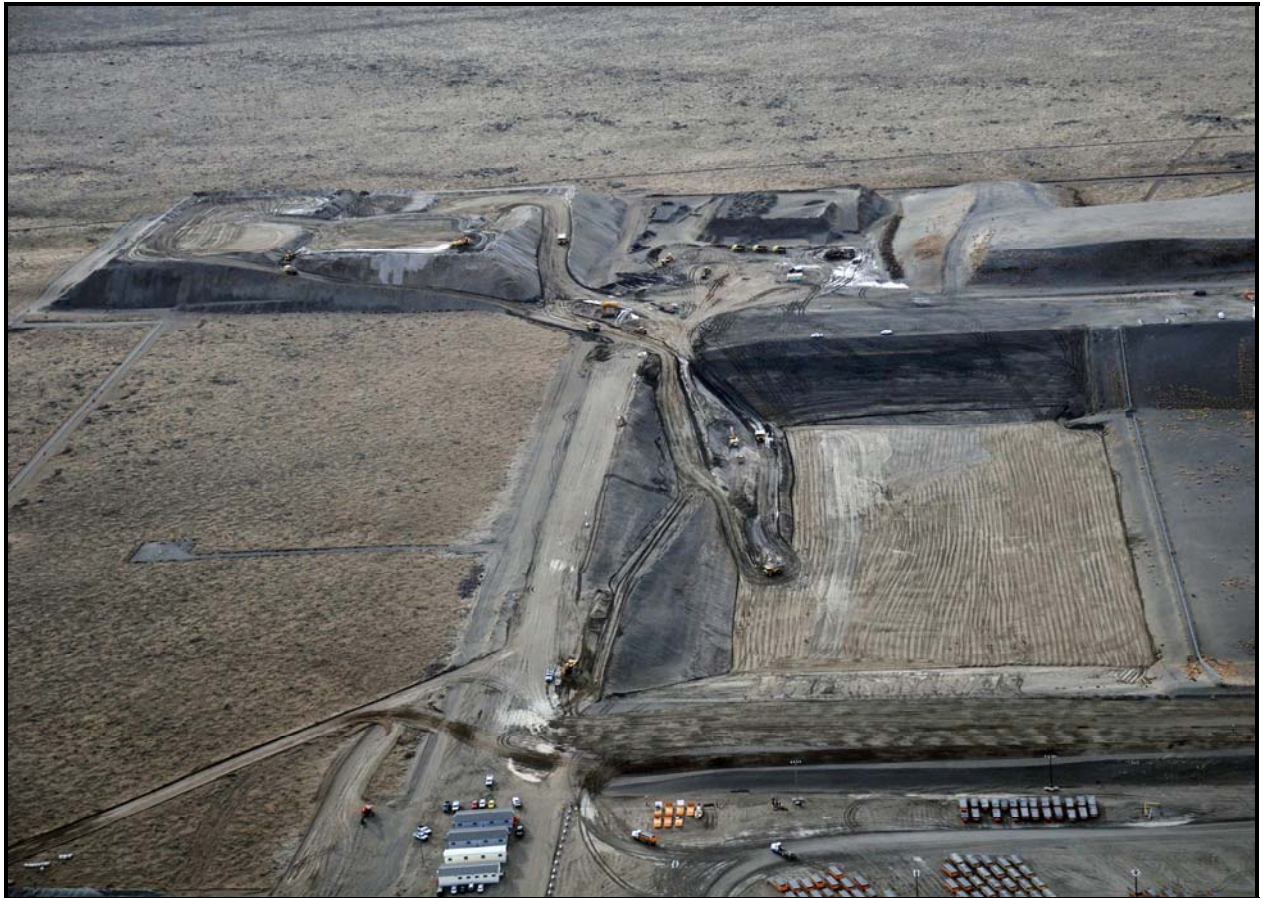
An aerial photo shows the conclusion of excavation activities at super cell 9, right, and the site of super cell 10 at the Environmental Restoration Disposal Facility.
